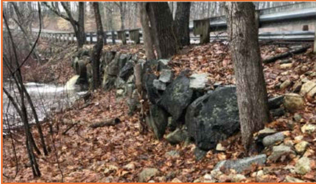
Woodman Brook - Downstream Showing Perched Outlet and Compromised Retaining Wall and Embankment
