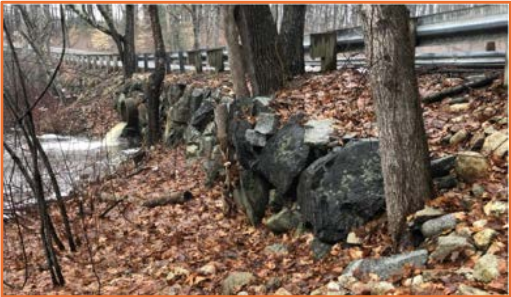
Woodman Brook - Downstream Showing Perched Outlet and Compromised Retaining Wall and Embankment
