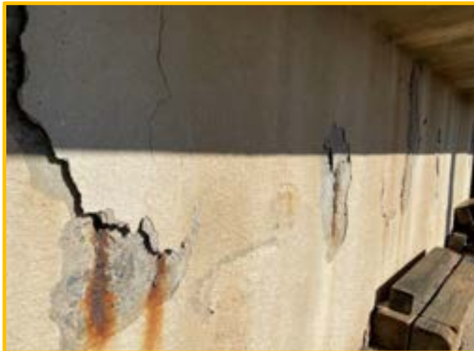
Control Building exhibiting concrete failure.
