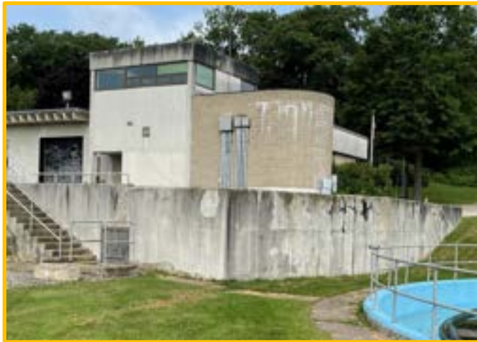
Retaining Wall requiring repair.
