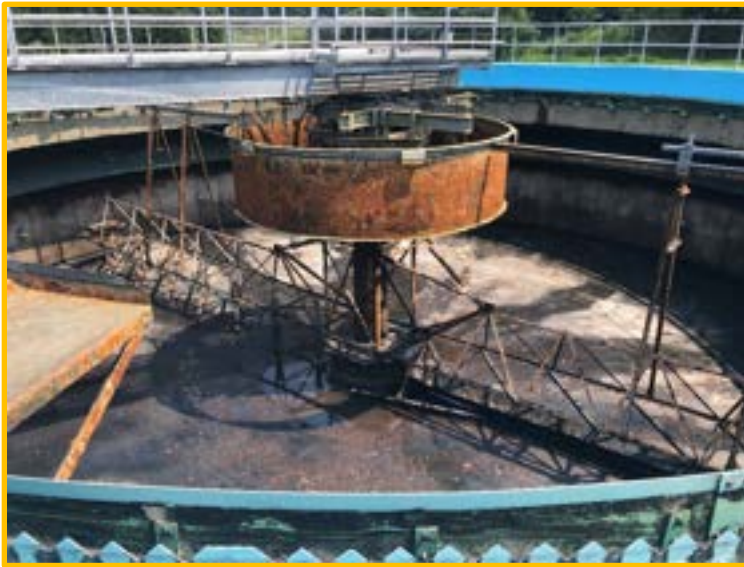
Secondary Clarifier with extensive corrosion. Note significant corroded/rusted material that fell off the mechanism shown on floor of clarifier.
