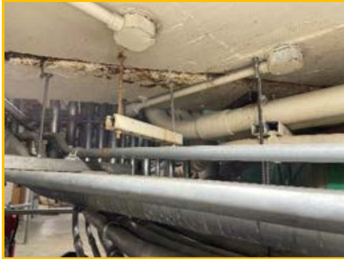
Pipe Gallery showing water intrusion at ceiling joint.
