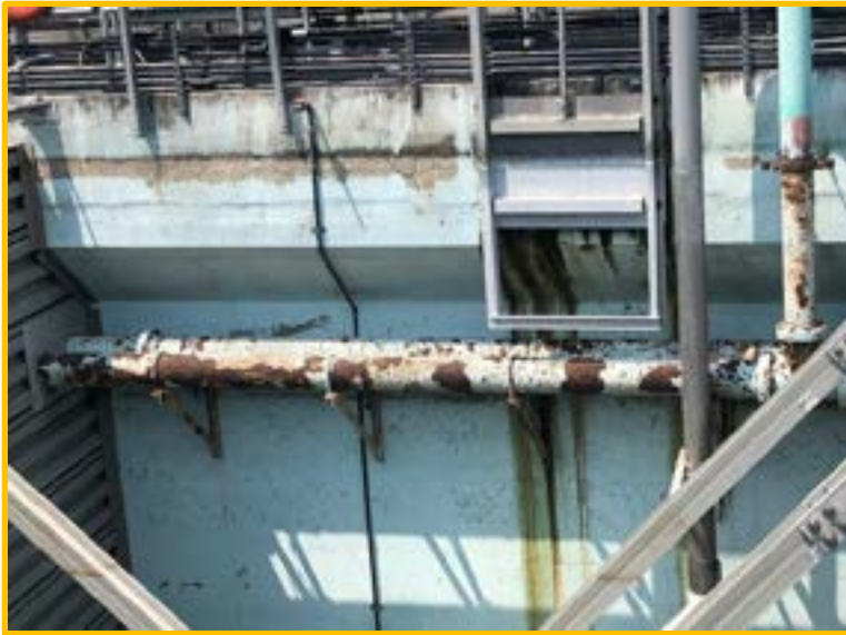
Aeration Tank showing corroded header and pipe supports.
