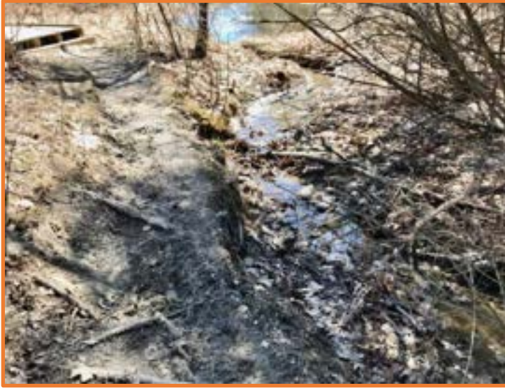
Figure 2 - Existing trail with substantial erosion into wetland and tidal marsh
