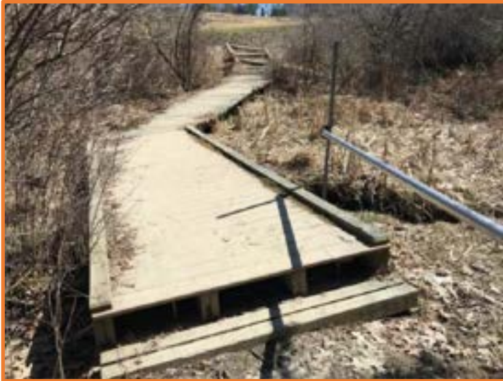
Figure 3 - Existing bridge crossing in disrepair
