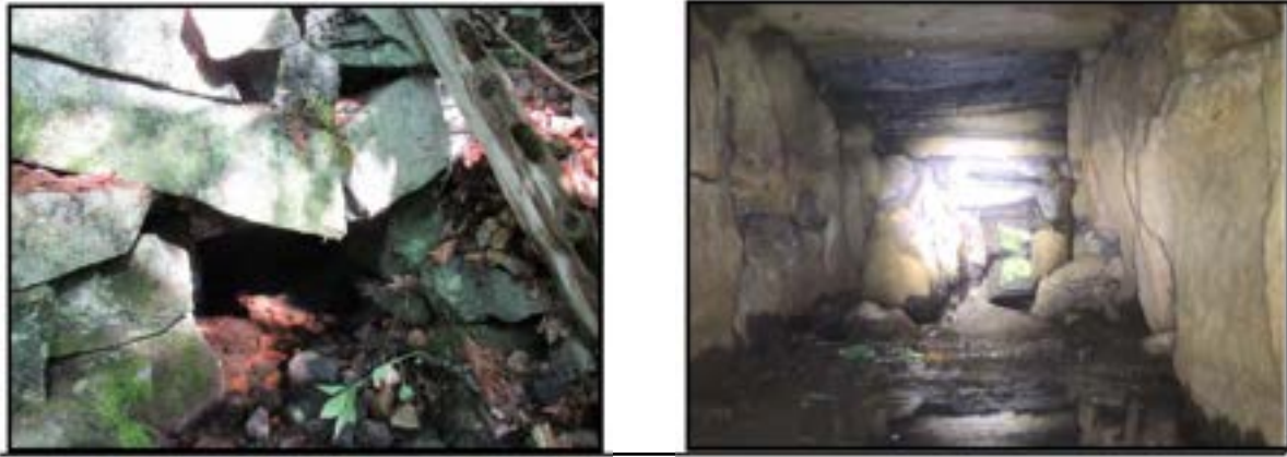
Snapped Stone at Outlet headwall – (Left) and Fallen Stones from Sidewall and Ceiling (Right) Littlehale Brook at Edgewood Road Stone Box Culvert
