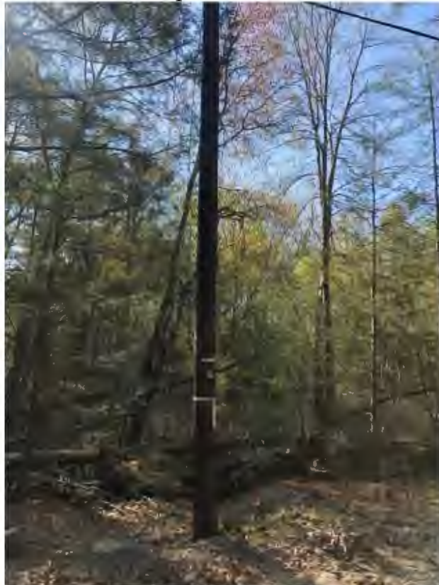
Figure 2 – Utility Pole Placement Near Dame Road Travel Lane
