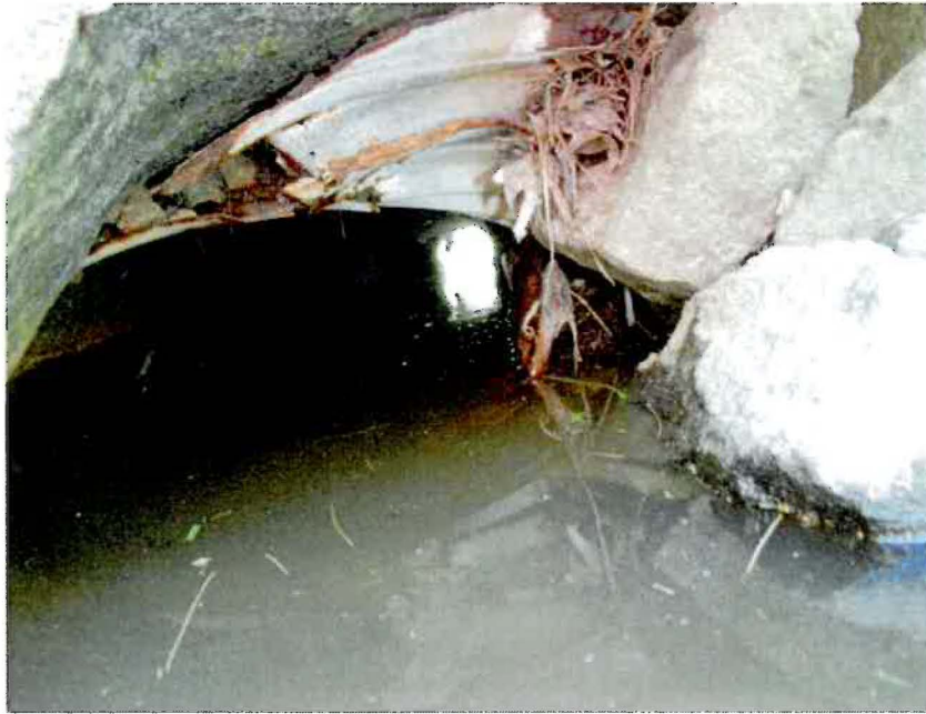
Collapsed Pipe at Ross Road over Ellison Brook Culvert Outlet
