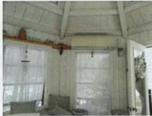
Inside Gazebo Finished Space Mini-Split for heat and A/C
