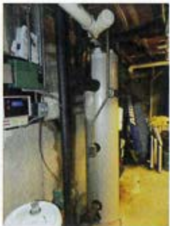
Hot Water Maker Basement
