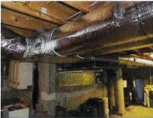
HydroAir Air Exchange & Hot Water Maker Basement
