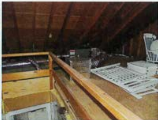
Air Exchange System Attic
