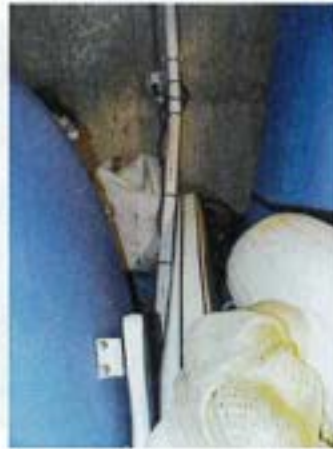
Sump Pump Basement
