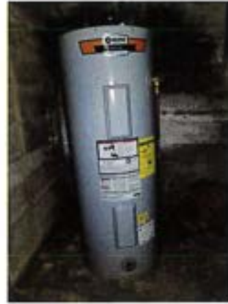
Hot Water Heater
