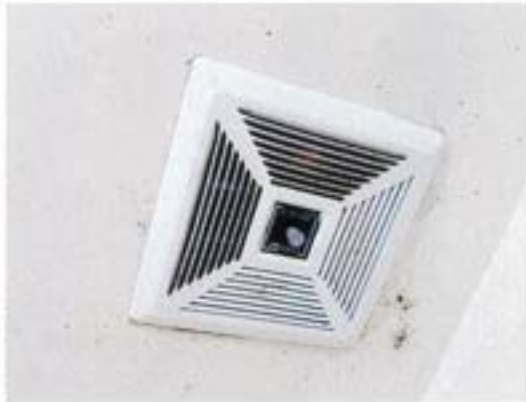
Full Bath — Ceiling Staining / Vent Area
