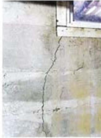
Foundation — Vertical Crack Observed
