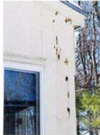
Exterior Siding — Woodpecker Damage
