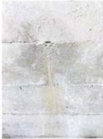
Foundation — Evidence of Moisture Intrusion
