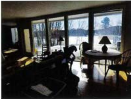
Living Room Windows — Fogged / Failed Thermal Glass
