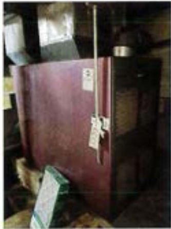
Primary Heating System
