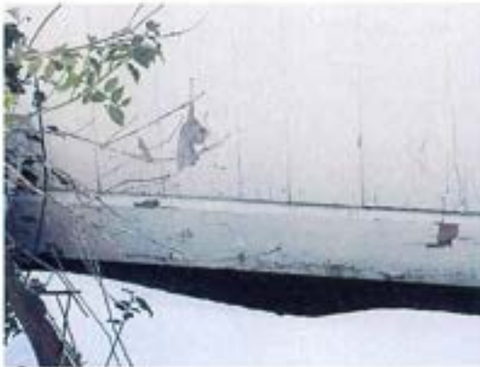
Exterior Siding — Peeling Paint / Deterioration
