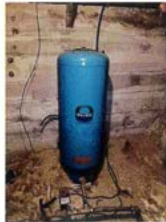
Well Pressure Tank
