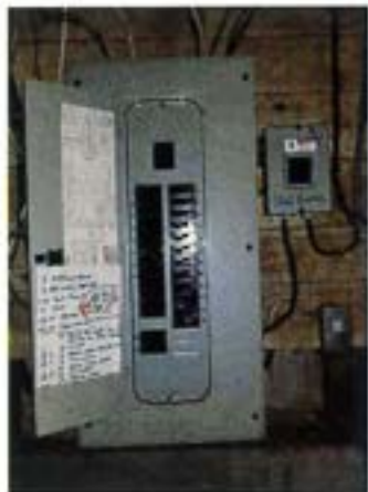
Electrical Panel - Main House
