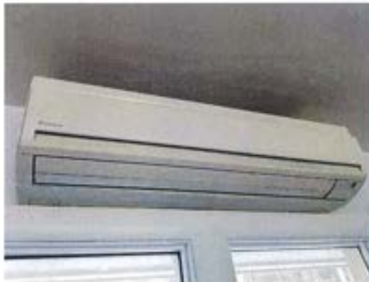
Ductless Heat & A/C Mini-Split
