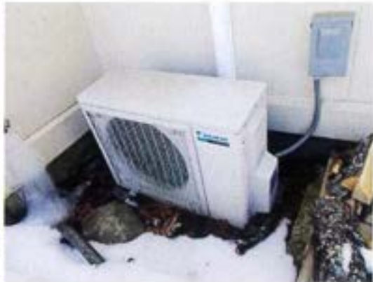
Ductless Mini-Split Heat Pump
