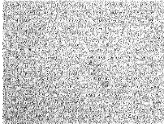
Living Room — Ceiling Damage / Prior Patch
