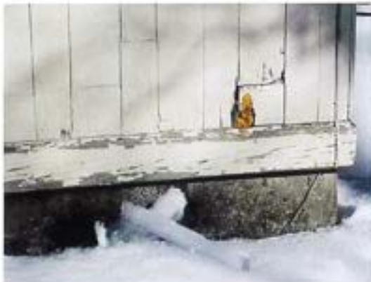
Exterior Siding — Peeling Paint / Deterioration
