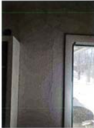
Bedroom #3 — Wall Cracking
