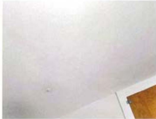
Bedroom #2 — Ceiling Damage / Prior Patch
