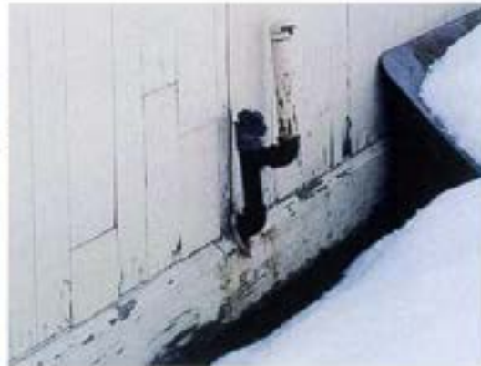
Exterior Siding — Peeling Paint / Deterioration
