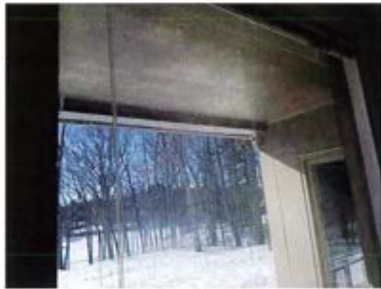
Living Room Windows — Fogged / Failed Thermal Glass
