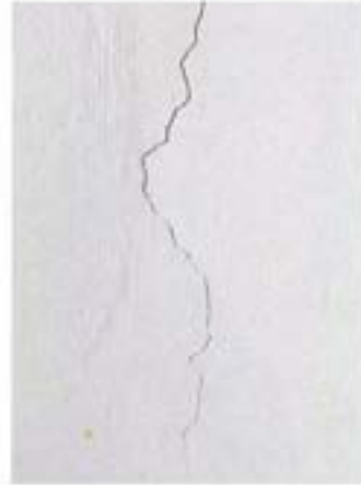
Bedroom #3 — Wall Cracking
