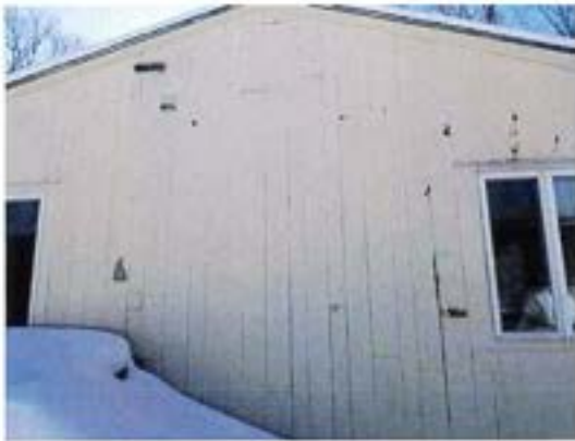
Exterior Siding — Peeling Paint / Deterioration
