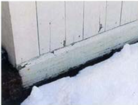
Exterior Siding — Peeling Paint / Deterioration
