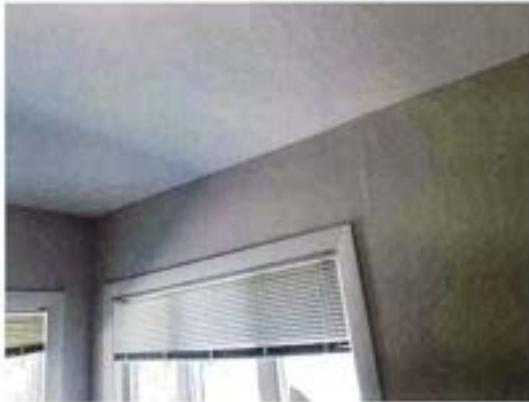
Bedroom #2 — Wall Damage / Prior Patch
