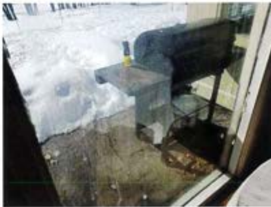
Living Room Windows — Fogged / Failed Thermal Glass
