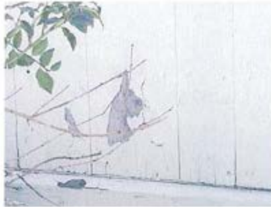
Exterior Siding — Peeling Paint / Deterioration
