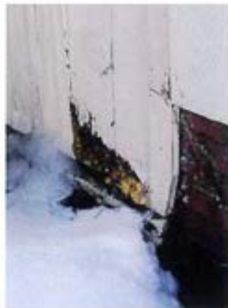
Exterior Siding — Localized Rot Observed
