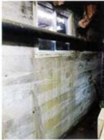
Foundation — Evidence of Moisture Intrusion
