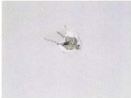
Primary Bedroom — Wall Damage
