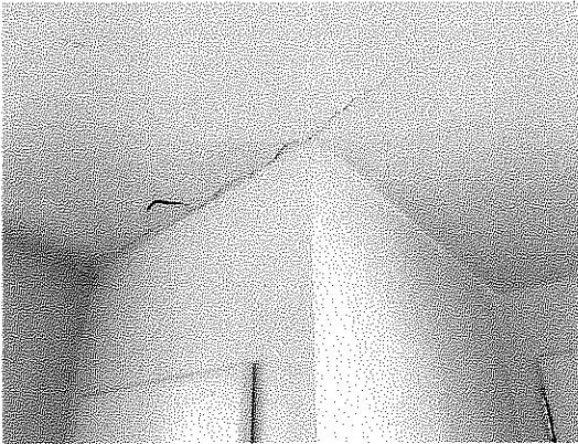
Kitchen — Ceiling Cracking / Drywall Separation
