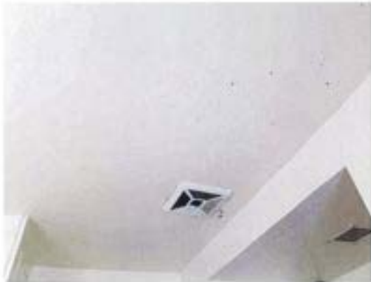
Full Bath — Ceiling Staining
