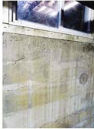
Foundation — Evidence of Moisture Intrusion
