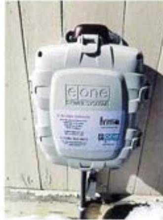
Sewer System Alarm Panel (See Attached Addendum)
