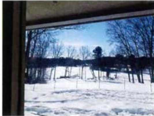
Living Room Windows — Fogged / Failed Thermal Glass
