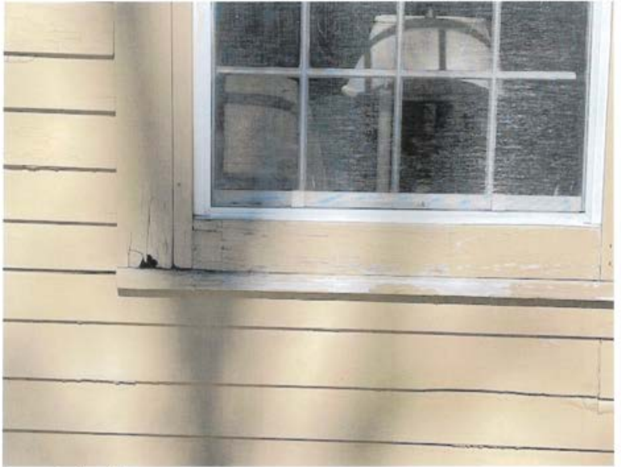
Rotten window sill
