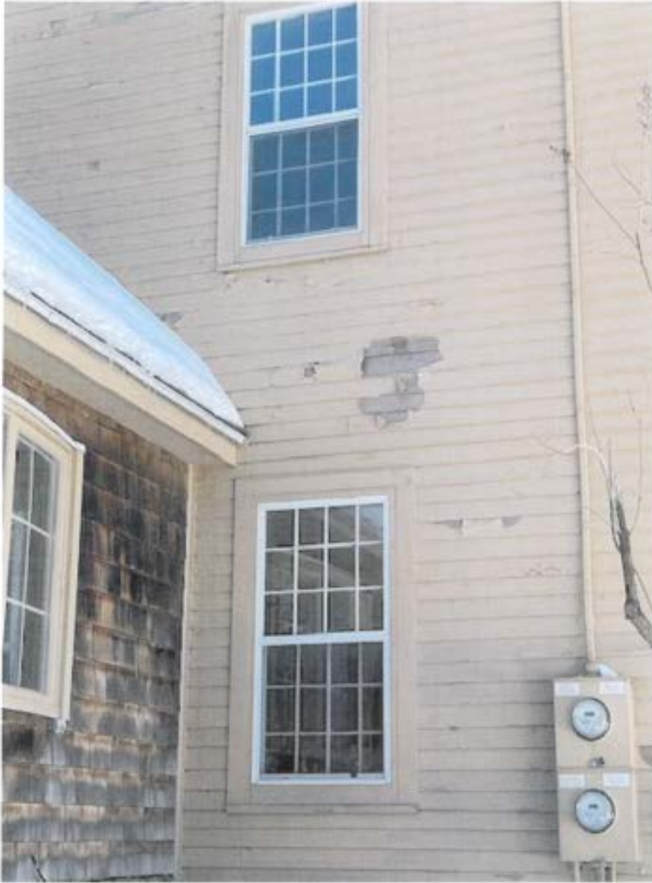
House requires painting/woodwork
