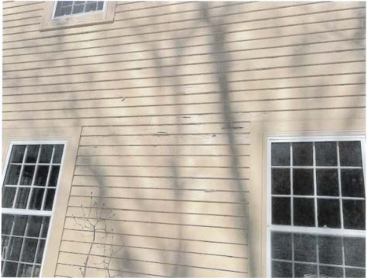
House requires painting
