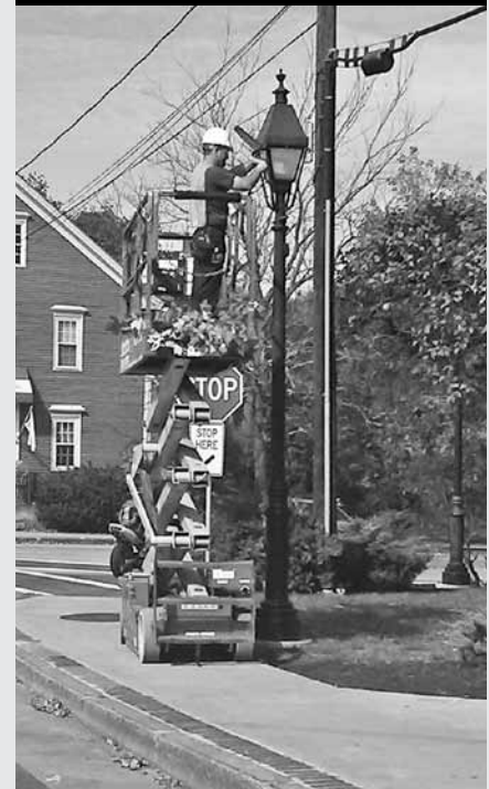
An employee from Sylvania installs light emitting diodes (LED) retrofit kits on the ornamental street lighting along the Main Street corridor and intersecting roadways fixtures. The Town competed for and was successful in obtaining an Energy Efficiency Block Grant valued at $167,310. The grant reimbursed the Town for 100% of the cost of the retrofitting. Todd I. Selig Photo
