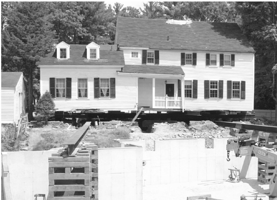
The foundation is poured and the platforms are in place to begin moving the Dewey Hannah House located on Packers Falls Road. RICHARD LORD PHOTO
