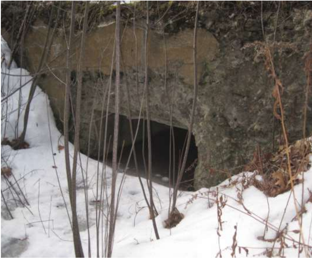
Image 50: Concrete culvert for Tom Hall Brook where it flows under the 1910 railroad embankment, Tom Hall Brook flows east to join Beards Creek in the Stolworthy Nature Preserve
