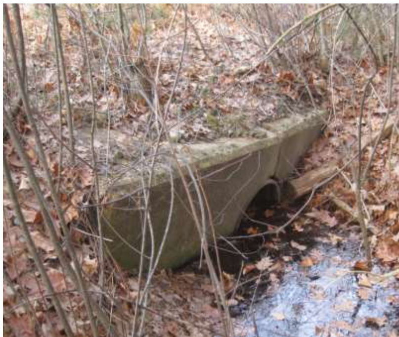
Image 49: Deteriorated concrete culvert under the track section dating from 1910
