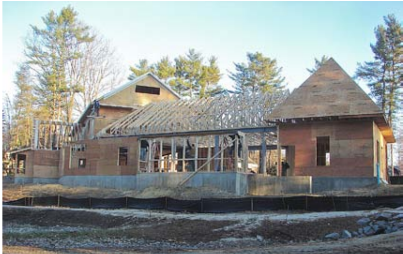
By late November 2012 the new library building was beginning to take shape with much of the wood framed portion of the exterior skin completed, roof trusses set, most of the roof sheathing installed, and exterior wall sheathing nearly complete. Courtesy Walter Rous
