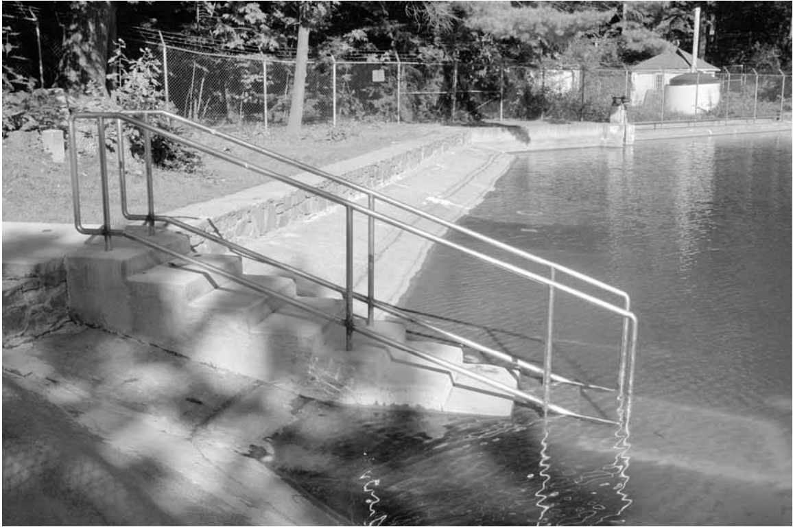
Photo 17: Northern end of pool, new stairs and railing, looking toward dam and treatment plant
