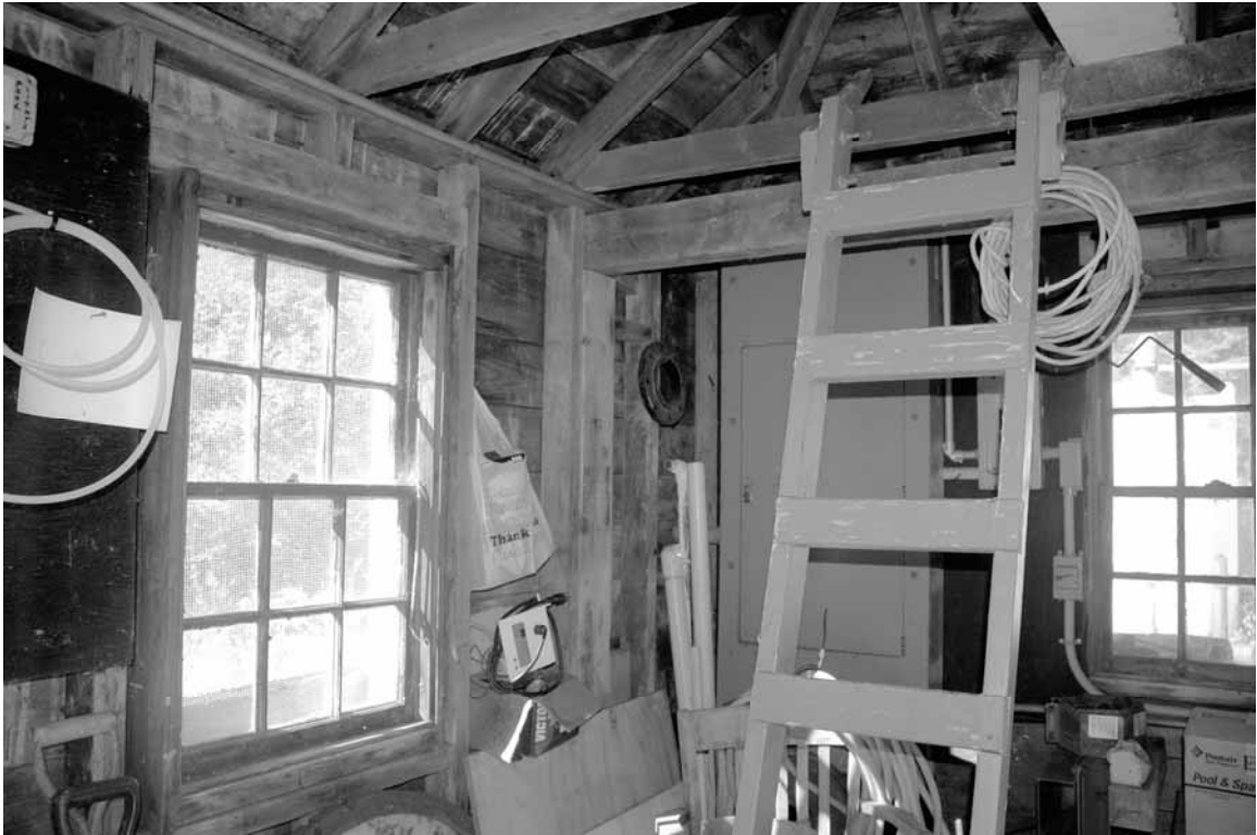
Photo 30: Filter House Interior
