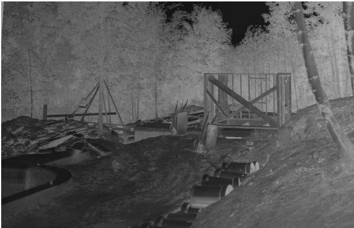
June 1938 Negative, construction of filtration building northeast corner of pool, facing northeast (UNH Archives 13.768).
