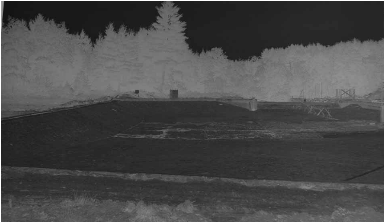
June 1938 Negative, facing-northeast, northern end of pool, looking toward dam and filter plant being built (UNH Archives 13.766)
