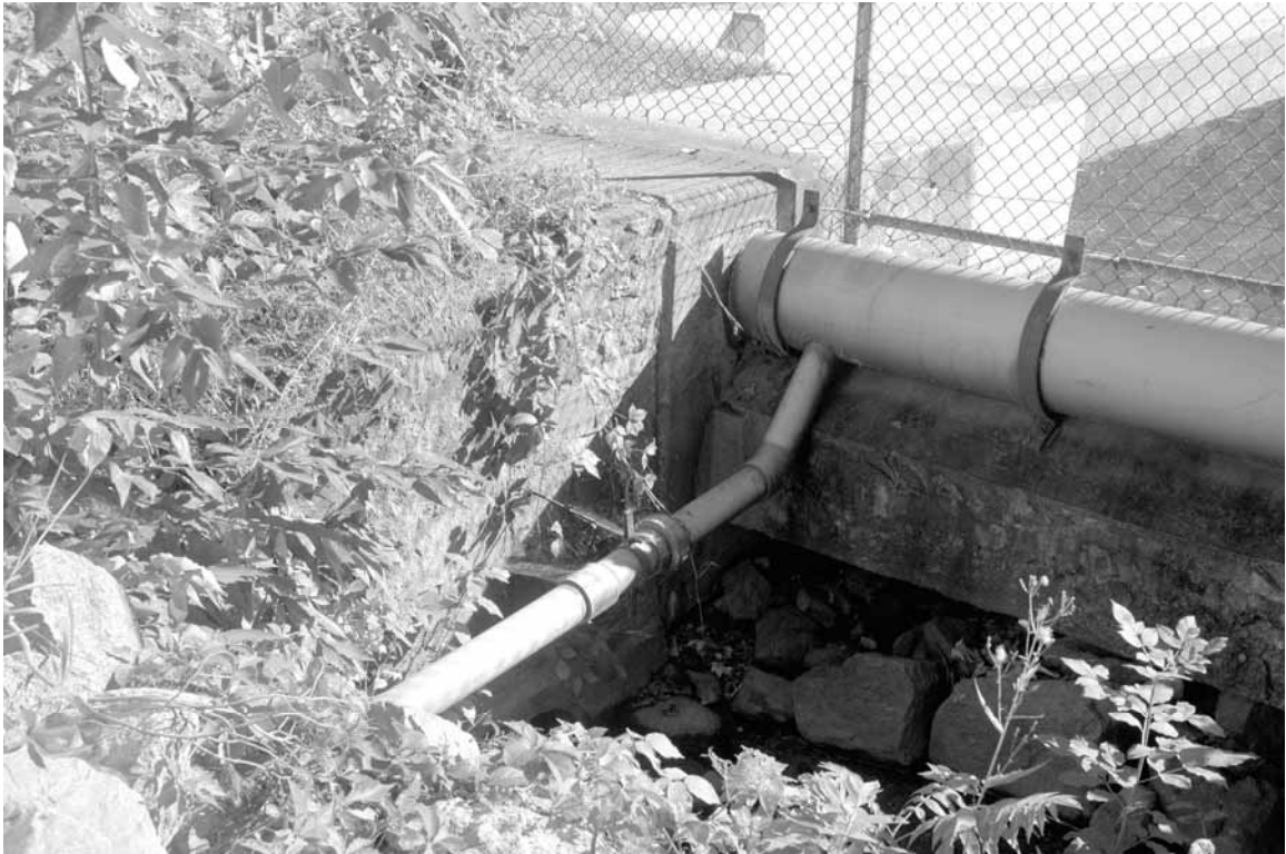
Photo 24: Dam back side, showing overflow catch piping
