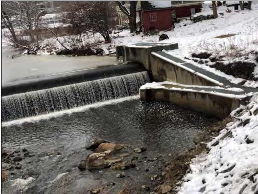
Photo No. 53: Overview of the fish ladder at the left end of the spillway..
