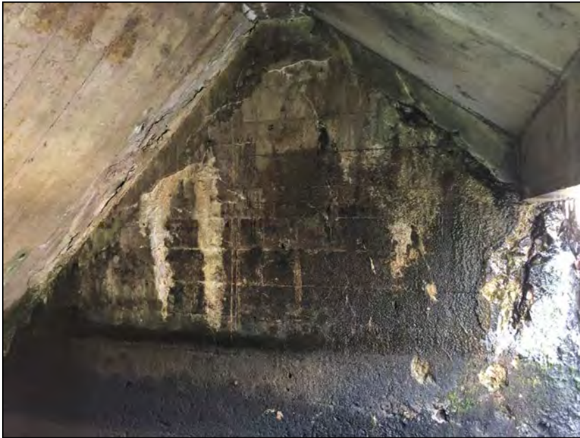
Photo No. 17: Left wall. Note scour and spalling on the downstream end and delamination on the upstream joint with the ceiling.
