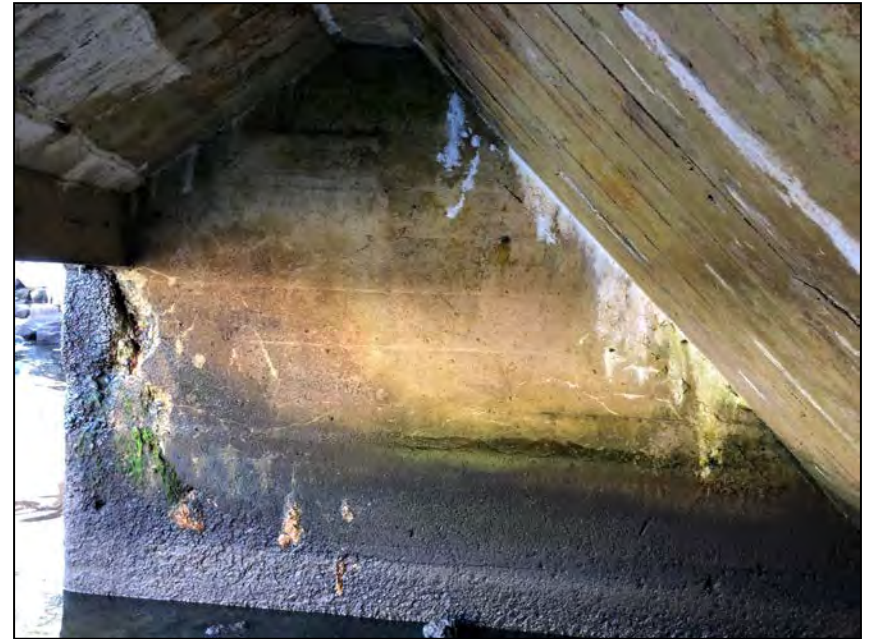
Photo No. 18: Right wall. Note scour and spalling on the downstream end.
