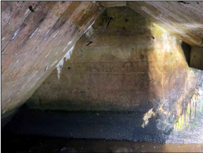
Photo No. 33: Left wall. Note efflorescent staining.
