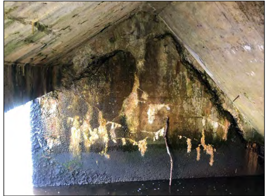
Photo No. 34: Right wall. Note crack and delamination extending along the upstream and upper side of the wall.
