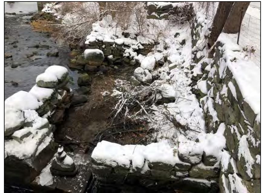
Photo No. 52: Remnants of the mill foundation downstream of the gate structure.
