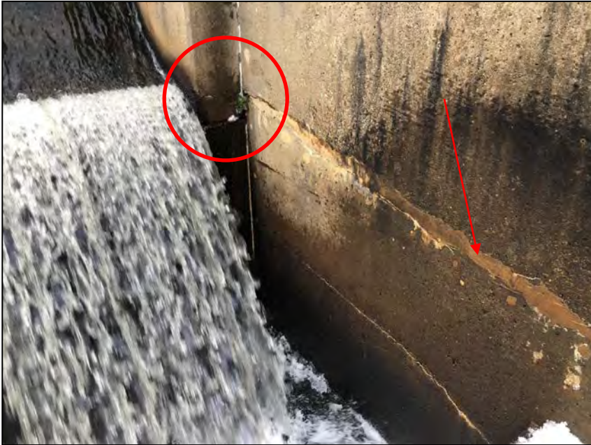
Photo No. 5: Area of the previously reported leakage from the left training wall. Note vegetation within the joint and repair along the wall.
