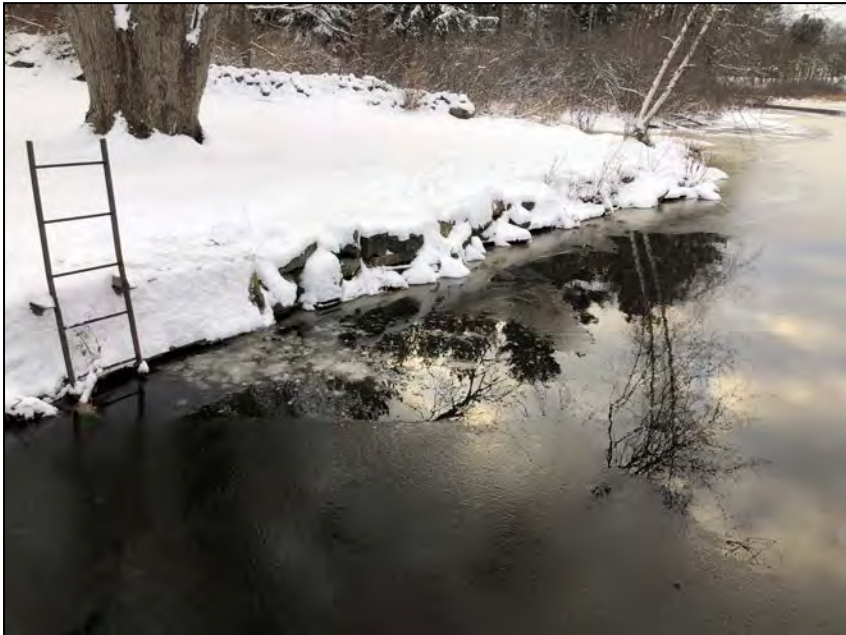
Photo No. 47: Right abutment upstream of the dam from the gate structure. Note snow cover.
