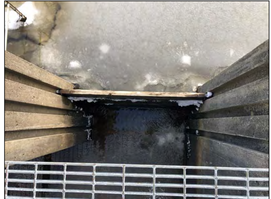
Photo No. 54: Fish ladder inlet with stop logs in. Note leakage from the stop logs.
