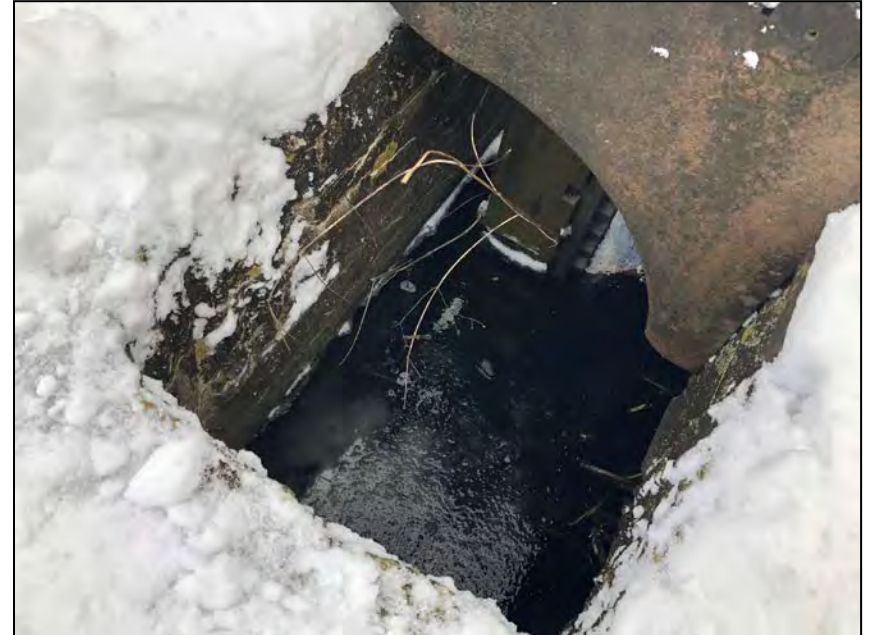
Photo No. 48: Inside of the top of the gate opening. Note irregular concrete typical in both gate openings.
