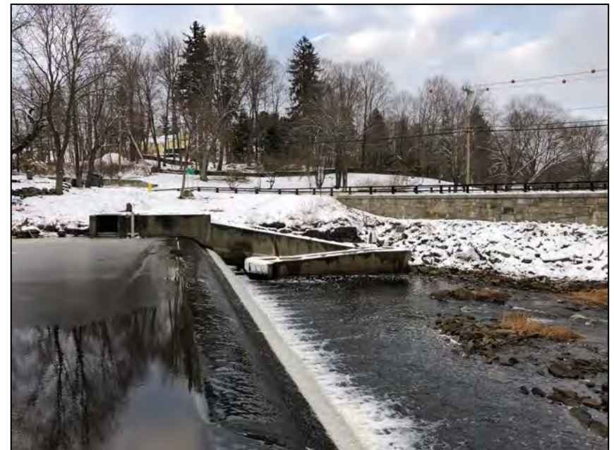
Photo No. 4: View of the left end of the primary spillway and training wall.
