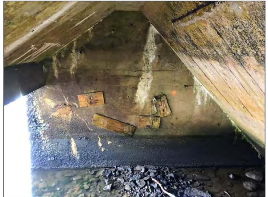
Photo No. 38: Right wall. Note repairs covered with timber falsework and spalling on the downstream end.
