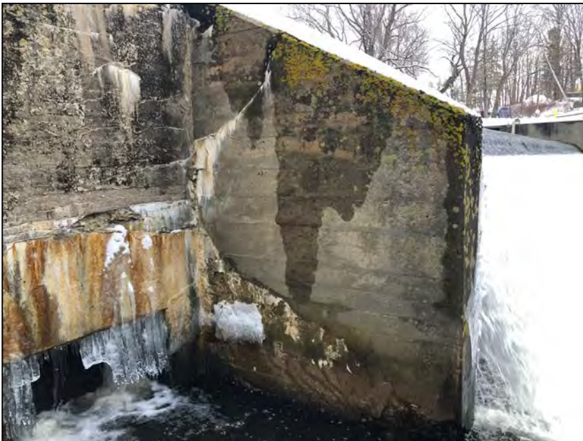
Photo No. 51: Right side of the right training wall and concrete downstream of the left gate. Note cracking with efflorescent staining and ice on the concrete. Additionally, note the leakage through the left gate.
