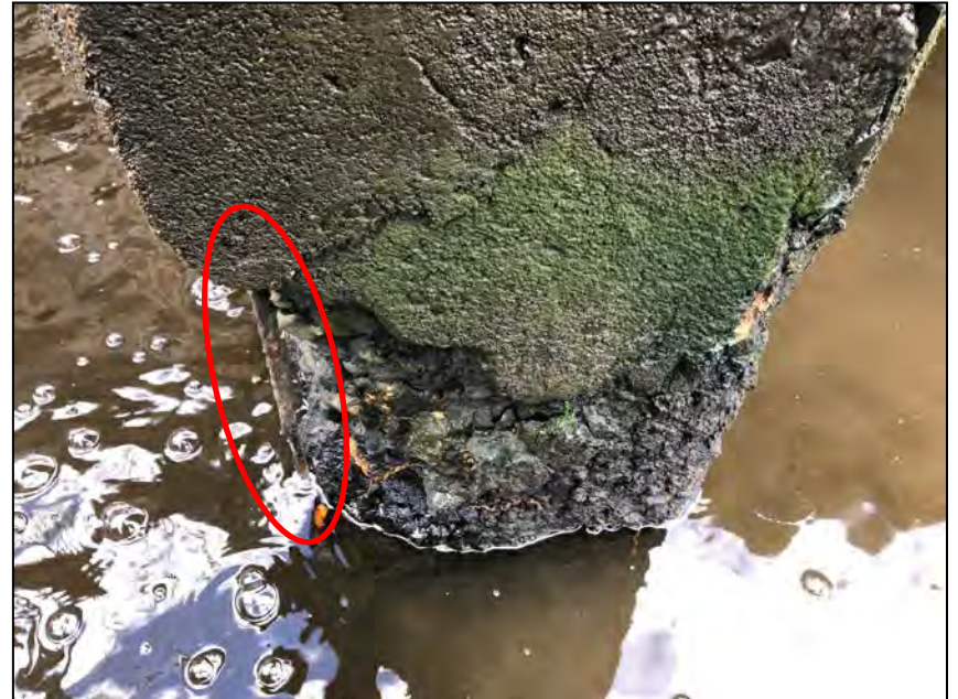
Photo No. 8: Scoured and severely deteriorated concrete with debonded rebar at the downstream side of the right training wall.
