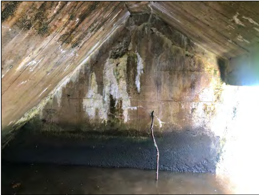
Photo No. 29: Left Wall. Note efflorescent staining and cracks.
