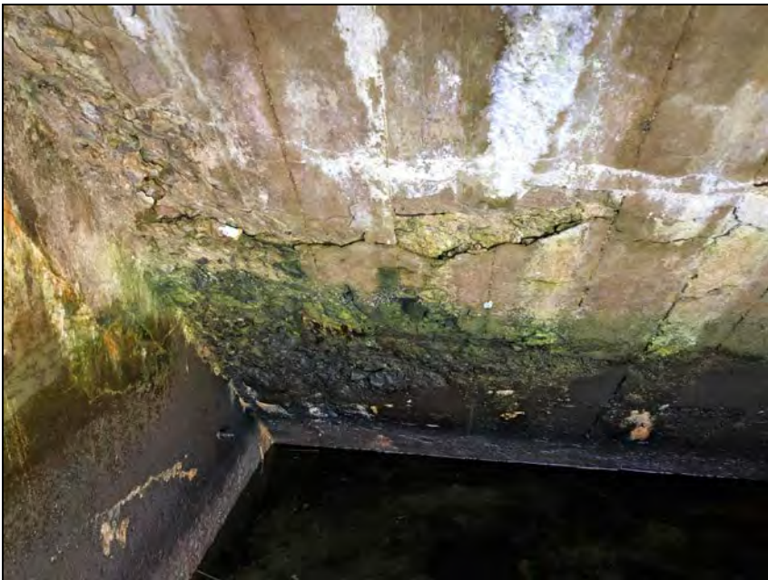
Photo No. 15: Delamination on the lower part of the upstream sloped ceiling (ceiling face no. 5).
