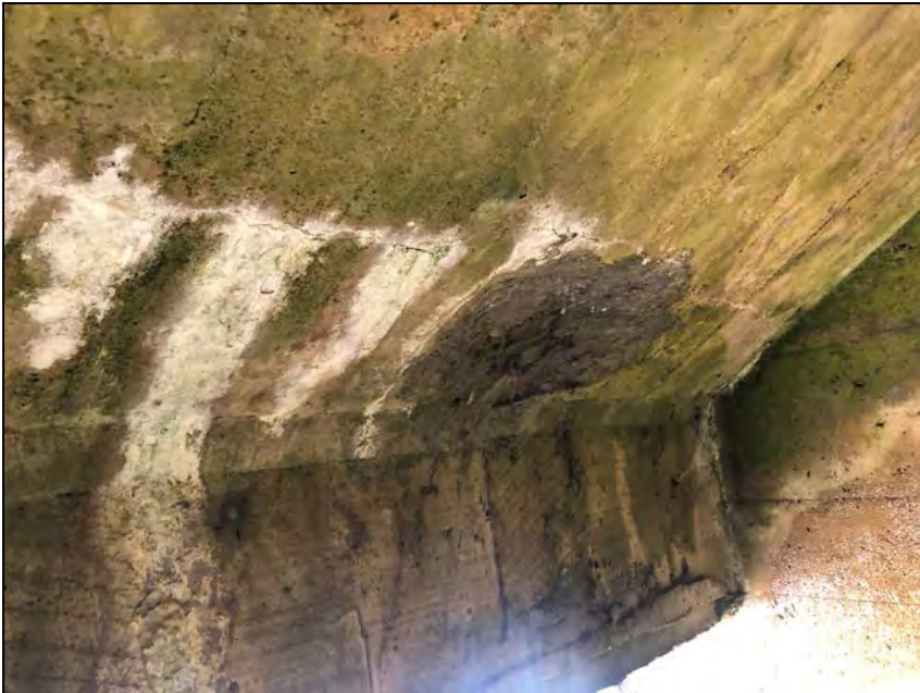
Photo No. 31: Repair on the right side of the downstream sloped ceiling,
