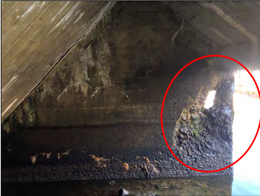
Photo No. 9: Left wall. Note section loss with spalling and scour on the downstream end.
