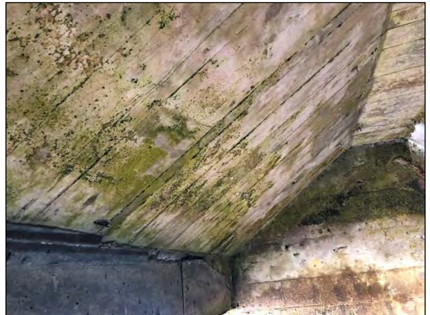
Photo No. 28: Downstream sloped ceiling (ceiling face no. 3).
