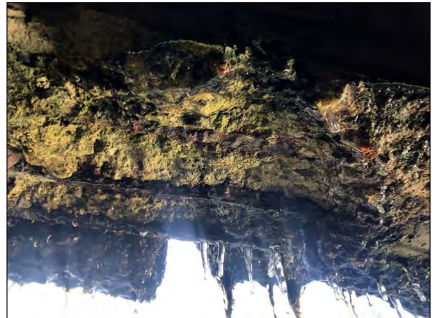
Photo No. 32: Spalling with debonded rebar on the underside of the downstream most ceiling (ceiling face no. 1).
