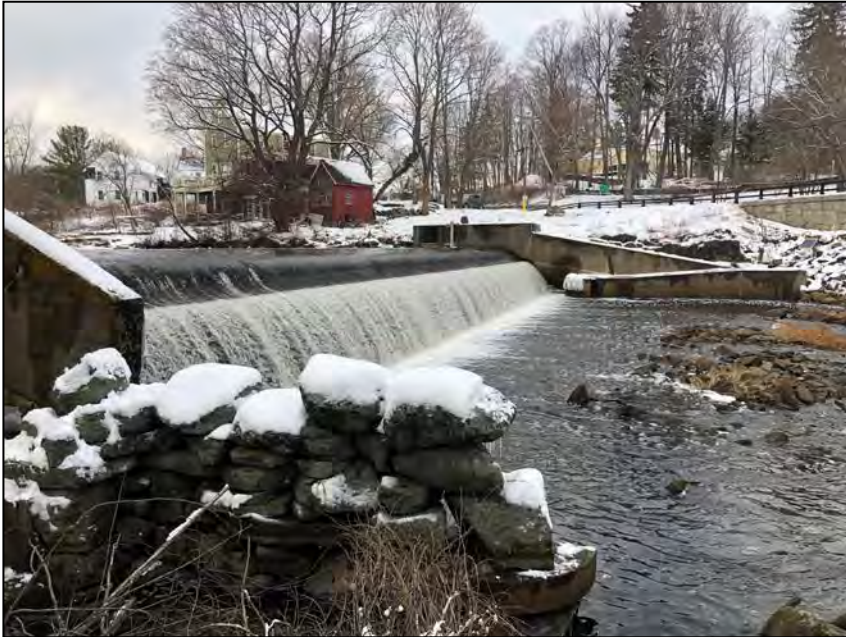
Photo No. 1: Dam from the right abutment looking left with flow over the spillway.
