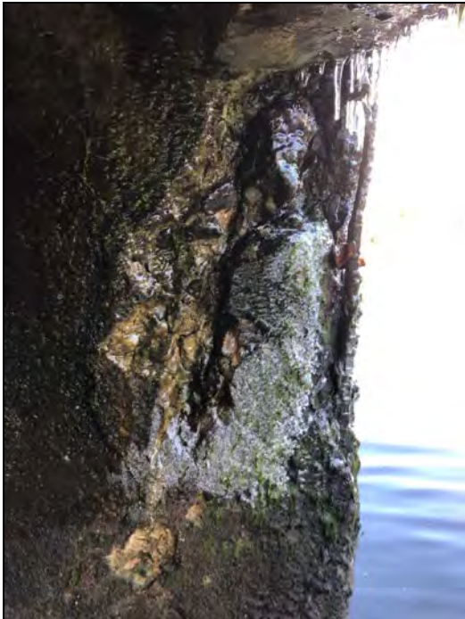
Photo No. 19: Delaminated rebar on the rib between Cell 3 and Cell 4.
