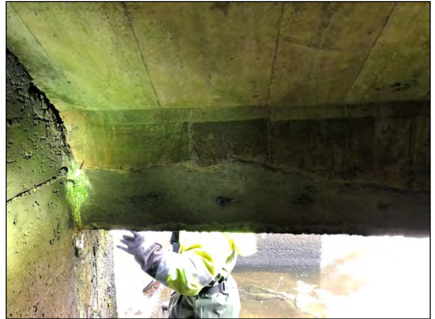
Photo No. 42: Repair on the downstream side of the cell (ceiling face no.2).
