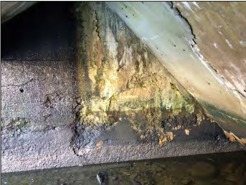
Photo No. 11: Right wall. Note spalling and delamination throughout the wall.
