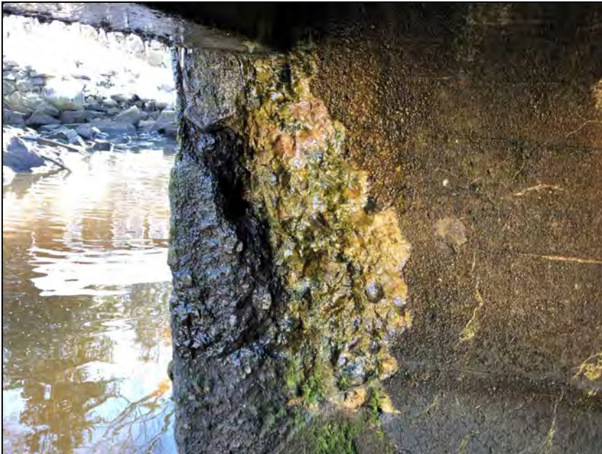
Photo No. 23: Spall with debonded rebar and 5-inch deep hole on the downstream end of the right wall.
