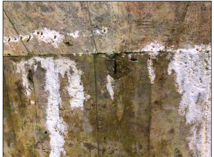
Photo No. 40: Area of exposed and deteriorated rebar on the downstream sloped ceiling.
