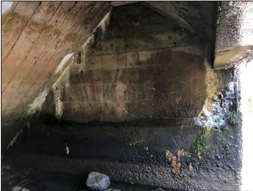
Photo No. 21: Left wall. Note debonded rebar and spalling on the downstream end.
