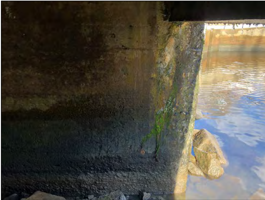
Photo No. 25: Left wall. Note scour and spalling on the downstream end approximately 1 foot above the waterline.
