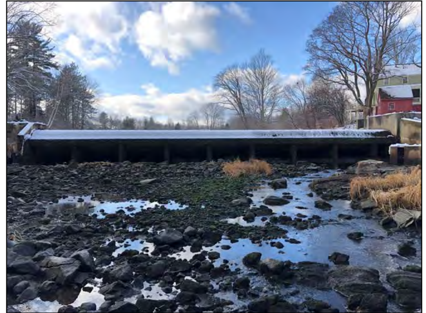
Photo No. 6: View of the downstream side of the dam with no flow over the spillway from under the bridge at Newmarket Road looking upstream.
