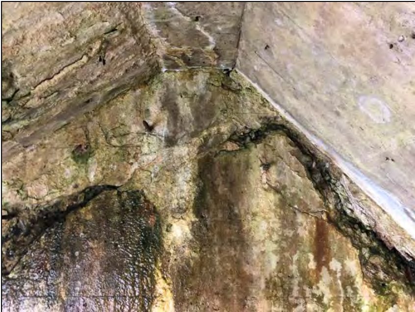
Photo No. 35: Delamination and crack with seepage below on the top of the right cell wall.
