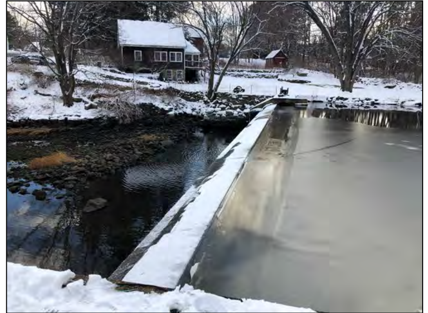
Photo No. 2: View of the upstream side of the crest from the top of the fish ladder looking right.
