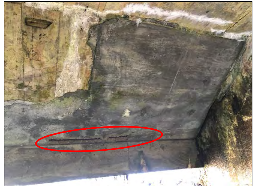
Photo No. 24: Downstream sloped ceiling with repair and exposed rebar.
