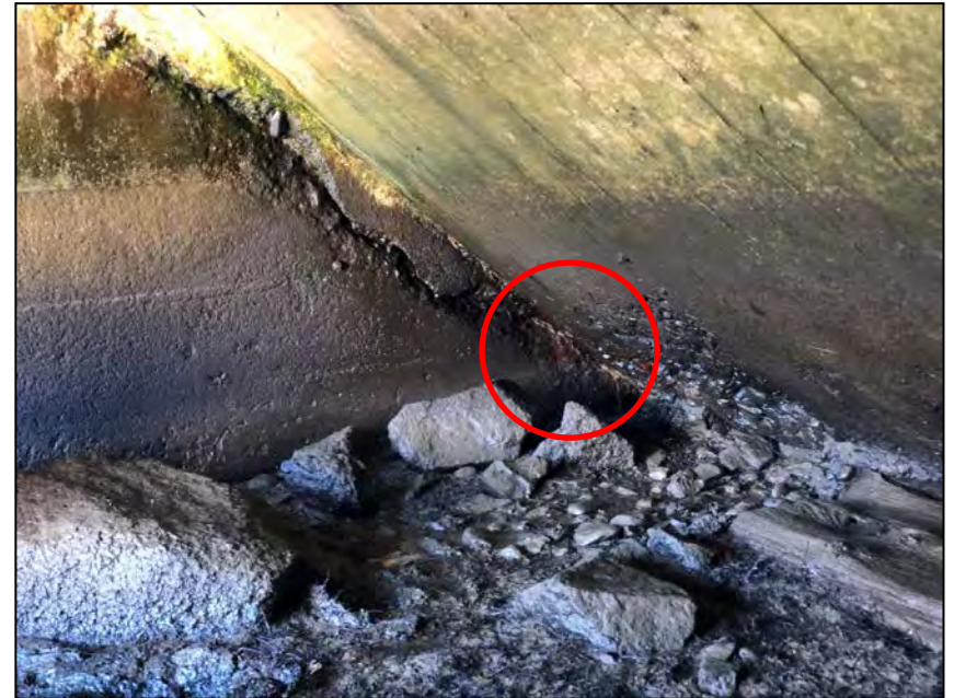
Photo No. 22: Large crack and spall along the right wall with iron oxide staining on the upstream end.
