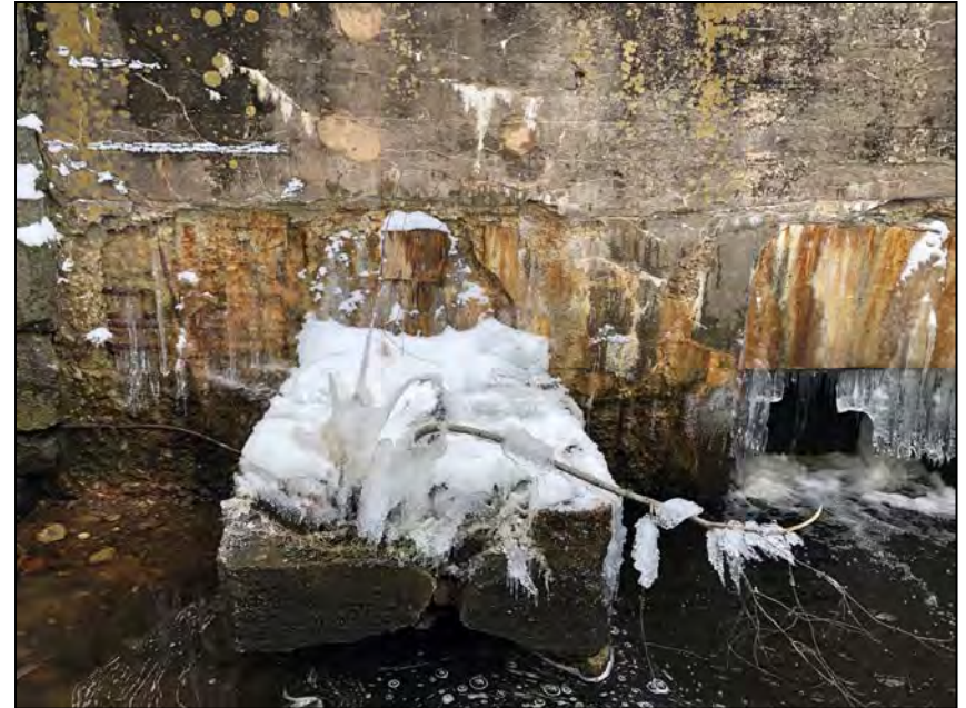
Photo No. 50: Left and right low-level outlets. Note the severe concrete deterioration and ice buildup throughout the downstream face of the structure.
