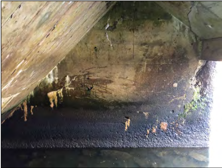
Photo No. 13: Left Wall. Note the scour and spalling on the downstream end.
