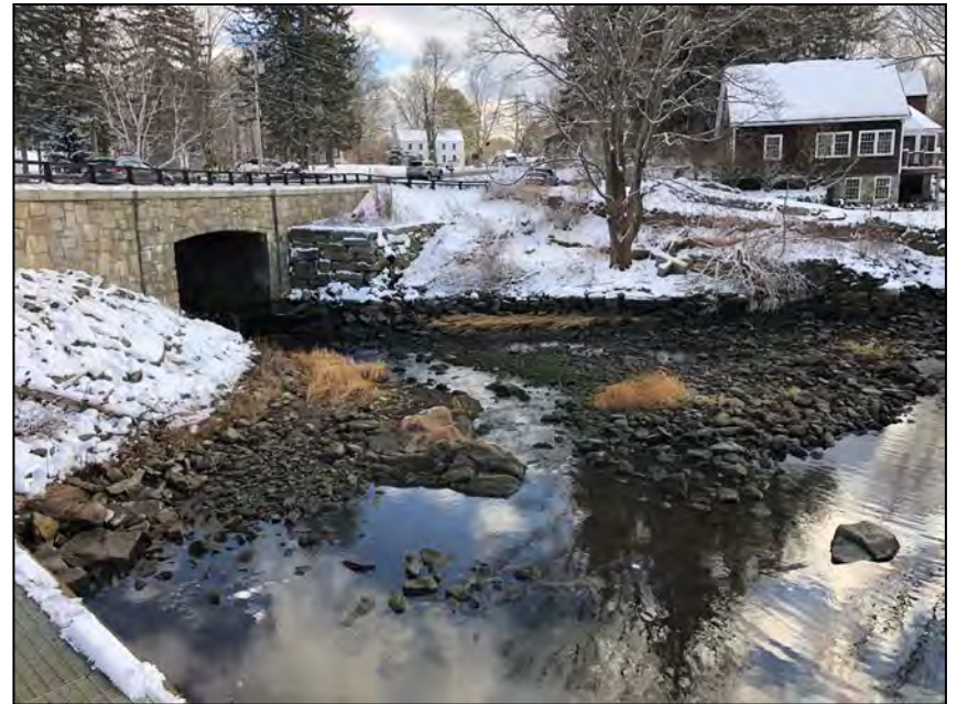
Photo No. 58: Downstream area of the dam from the top of the fish ladder.
