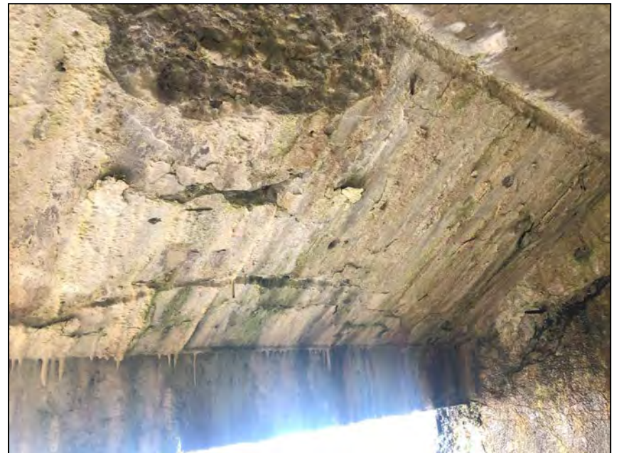
Photo No. 36: Delamination and efflorescence throughout the downstream sloped ceiling.
