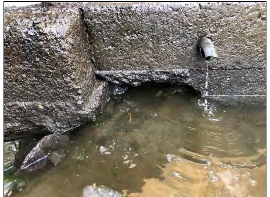
Photo No. 56: Scour and undermining underneath the right training wall of the fish ladder. Note void probed up to 3 feet.
