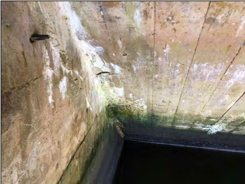
Photo No. 27: Efflorescent staining and delamination on the right side of the upstream sloped ceiling
