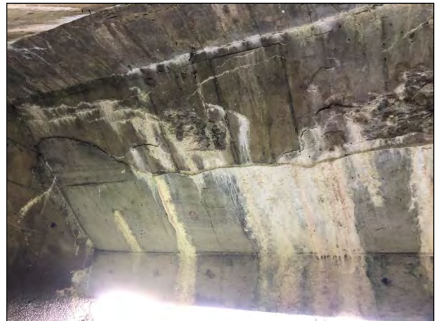
Photo No. 12: Repair on the downstream sloped ceiling section (ceiling face no.3). Note delamination above the repair and efflorescence.
