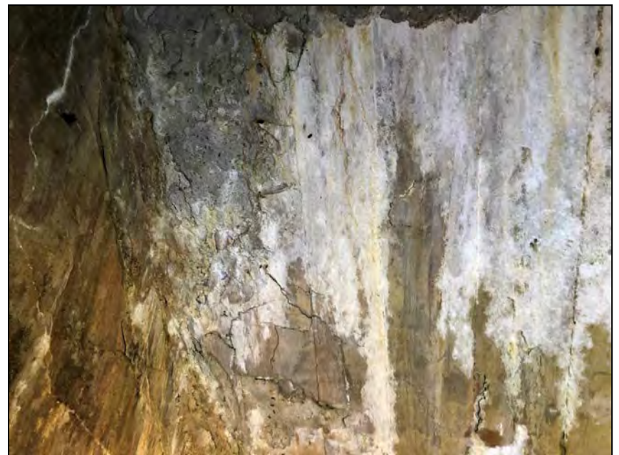
Photo No. 16: Delamination on the upper part of the upstream sloped ceiling (ceiling face no. 5).
