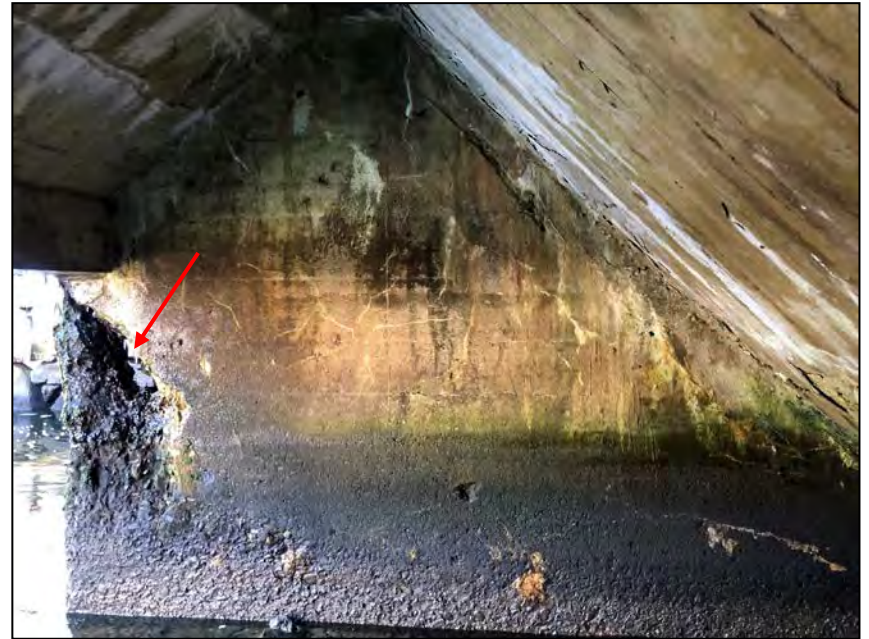
Photo No. 14: Right Wall. Note the section loss on the downstream end.
