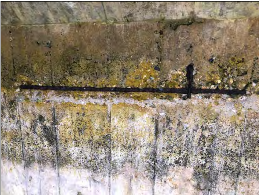
Photo No. 39: Exposed and deteriorated rebar on the upstream sloped ceiling.
