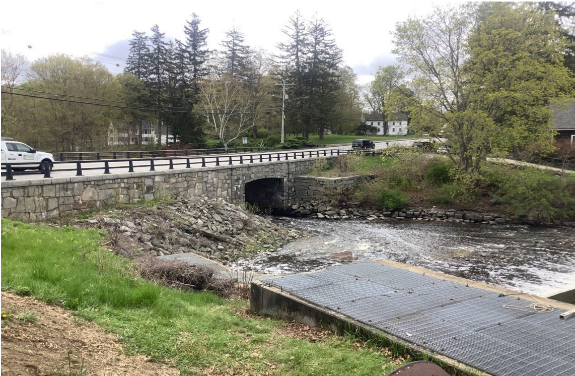
Photo 4: View southeast of the upstream side of the Newmarket Road bridge over the Oyster River. 05/05/2023.
