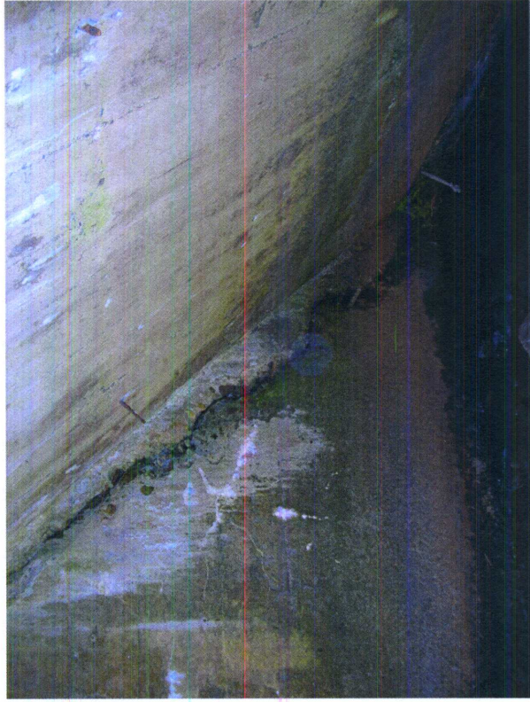
bay 5 - Cracking in Bay 5/4 support wall
