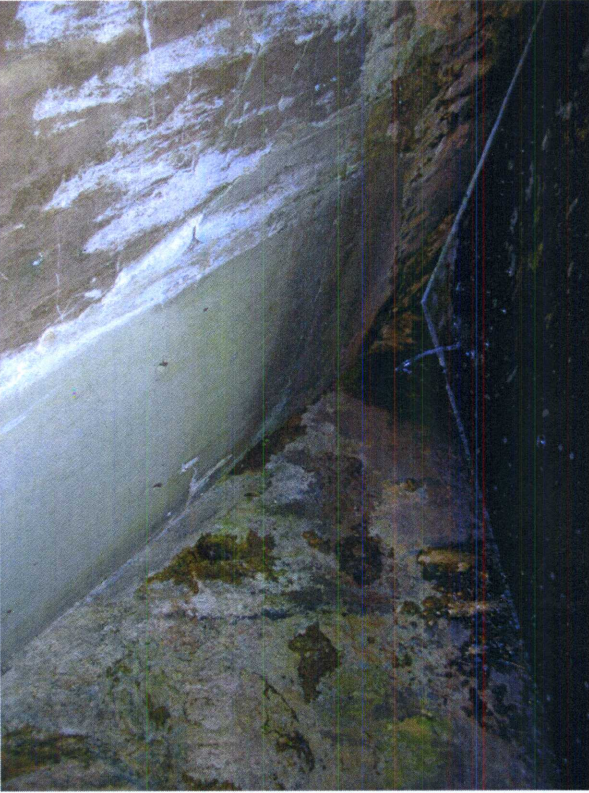
Bay 1 - active leak on connecting gate house wall
