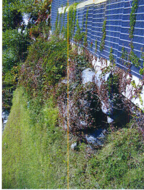
Some settlement of left embankment near fishway
