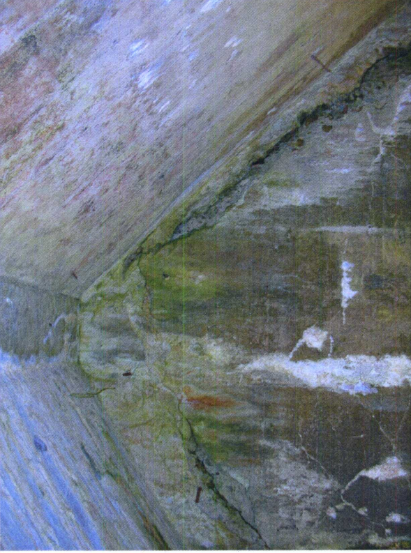
Bay 5 - cracking in bay 5/4 support wall
