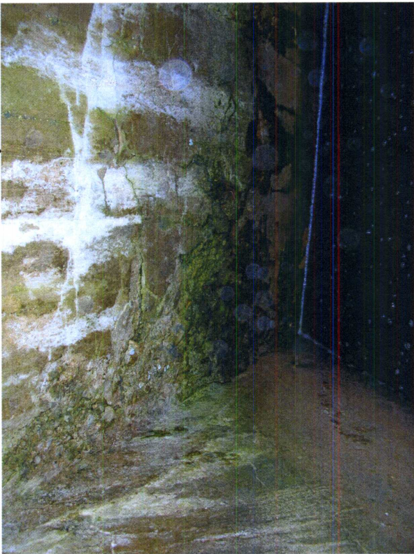
Bay 2 - concrete deterioration
