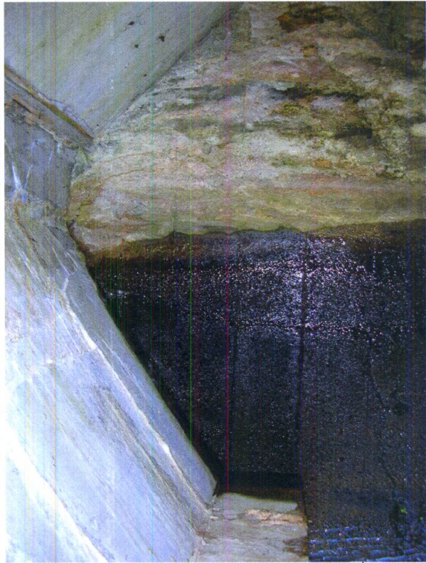
Bay 1 - active leakage from spillway slab adjacent to gate chamber
