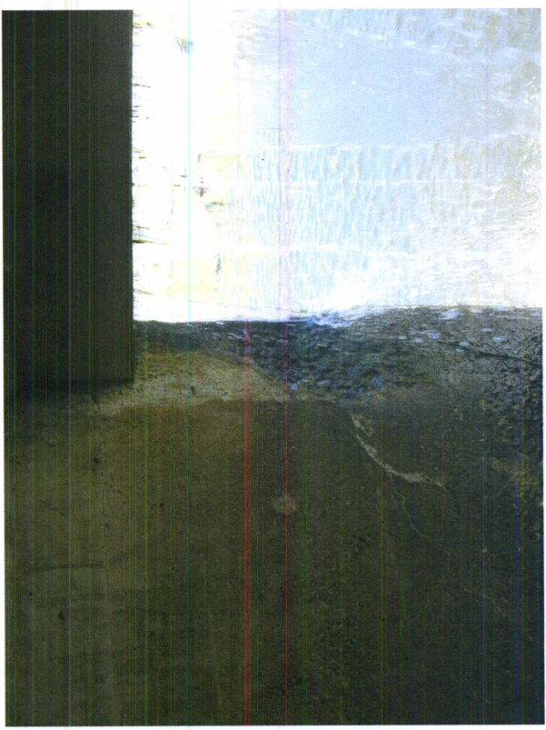
Bay 3 - Deterioration on Pier 3/4
