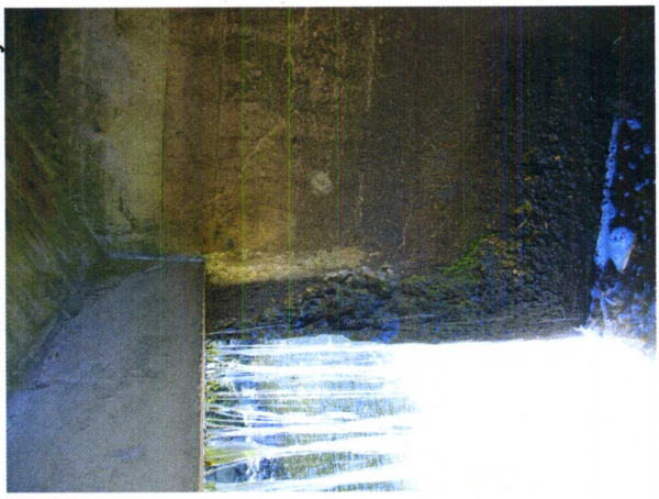
Bay 4 - Deterioration on Bay 4/3 pier
