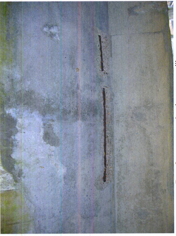
Bay 2 - exposed rebar on ceiling
