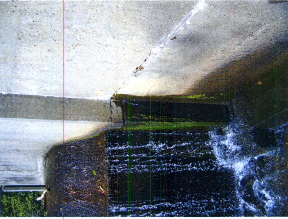
Leak in left spillway training wall at fishway
