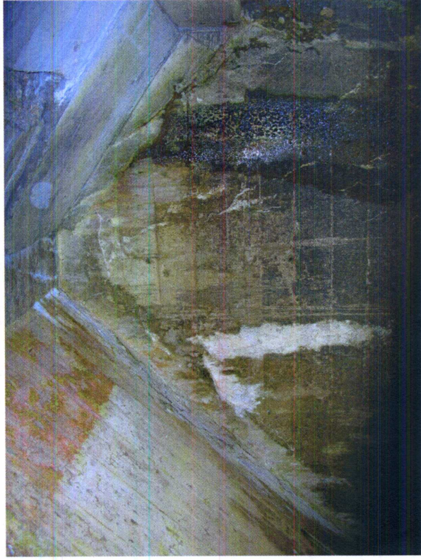
Bay 2 - leaking on pier 2/3
