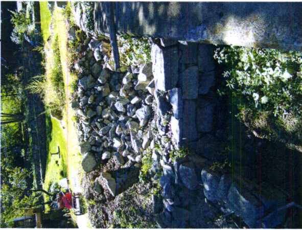
Failed mill foundation - stone was added to stabilize area
