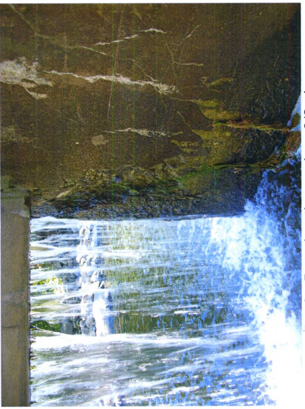
Bay3 - Deterioration on bay 3/2 pier
