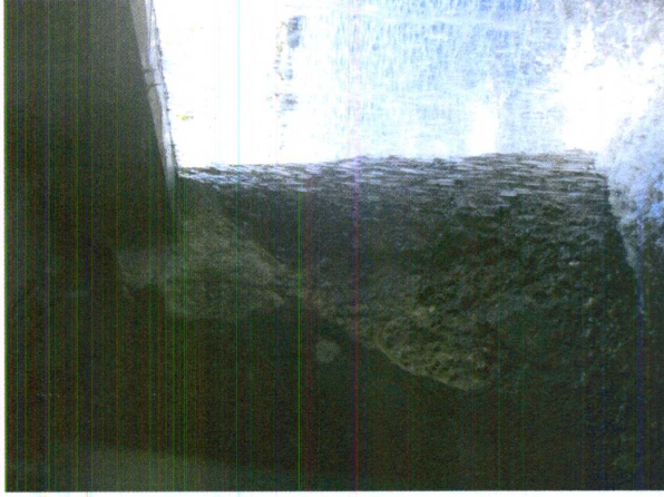
Bay 1 - concrete deterioration on Pier 1/2
