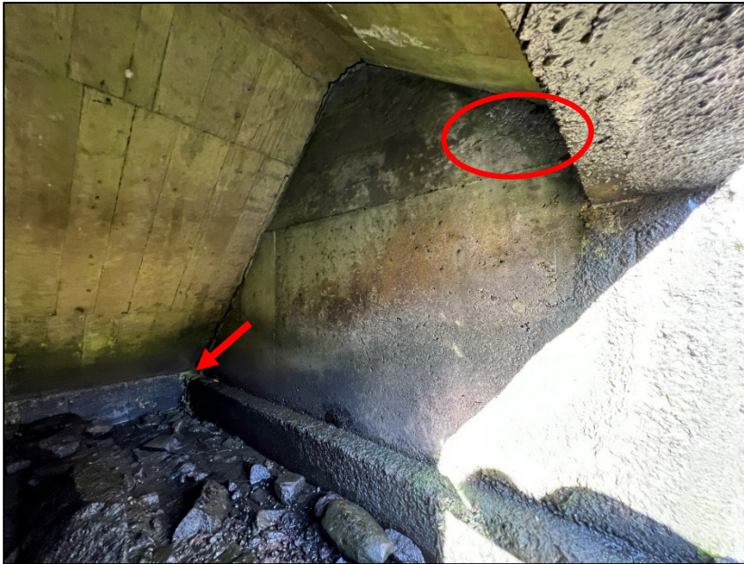
Photo No. 41.: Left Wall. Note evidence of poor concrete consolidation along the top of the wall at ceiling face no. 3 (circle). Previous location of iron oxide staining (arrow)
