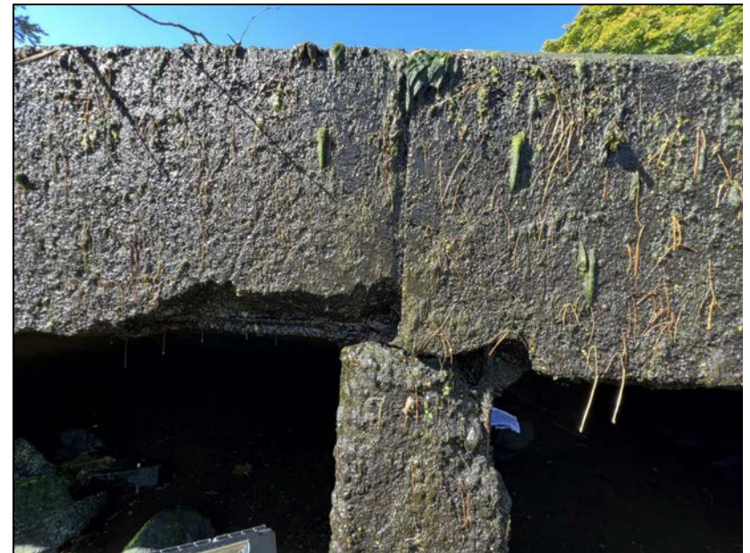
Photo No. 32.: Section loss and debonded rebar along the top of the rib between Cell 6 and Cell 7.
