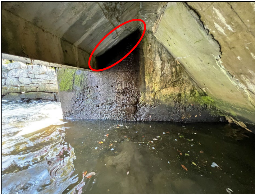
Photo No. 10.: Right wall. Note leakage along the interface between the ceiling and the right wall.
