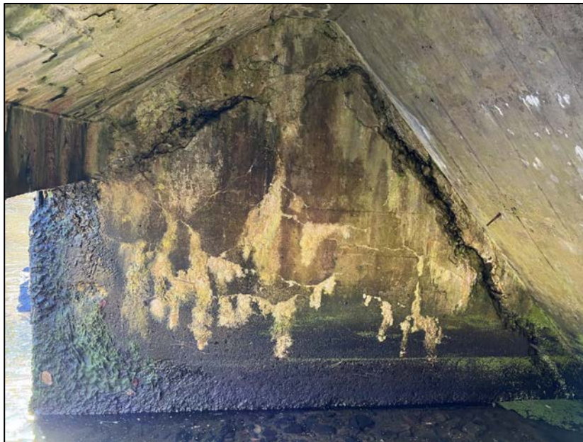
Photo No. 34.: Right Wall. Note cracking and spalling throughout the right wall and the upstream slope of the right wall.
