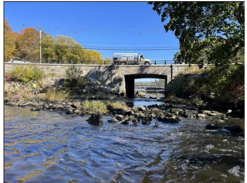
Photo No. 56.: Downstream area of the dam looking downstream at the bridge carrying Newmarket Road.
