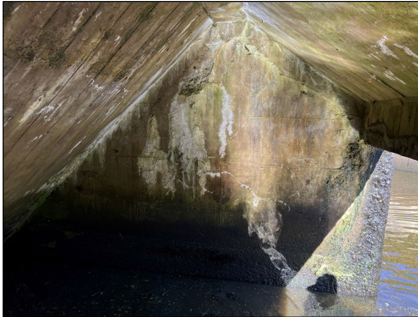
Photo No. 29.: Left Wall. Note efflorescent staining and cracking.
