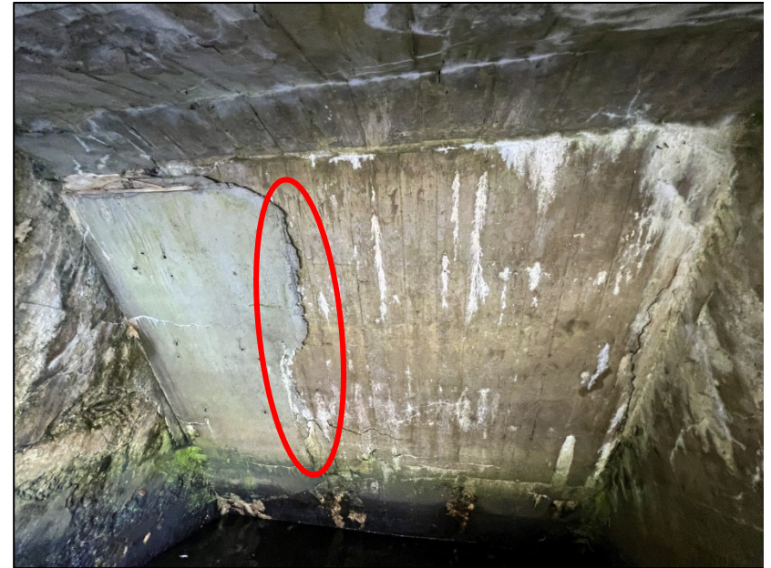
Photo No. 11.: Upstream sloped ceiling. Note location of delamination along repairs.
