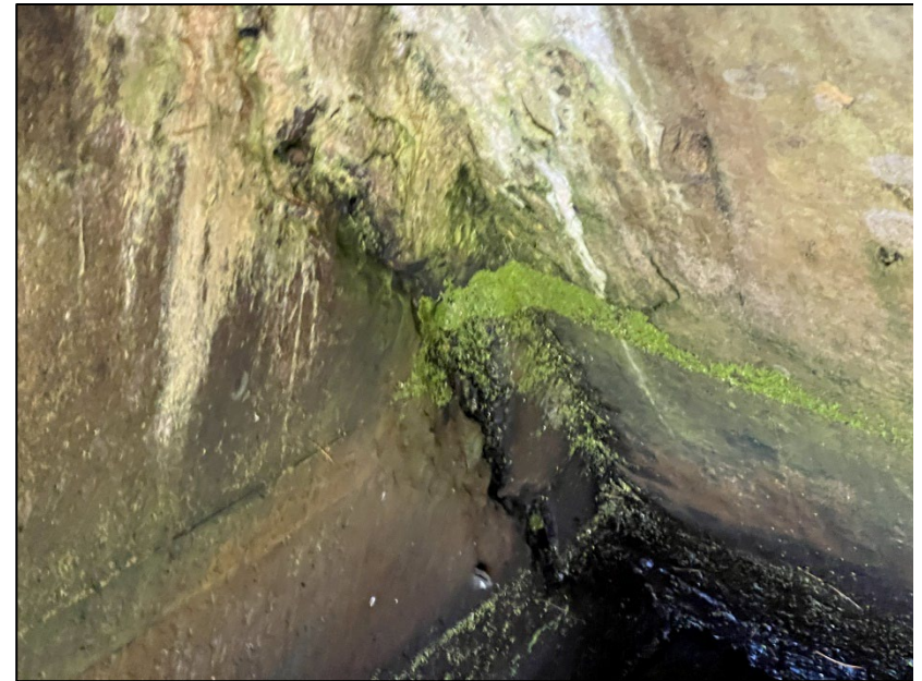
Photo No. 24.: Close-up view of the crack along the upstream side of right wall. Note iron oxide was previously observed within crack but not observed during this inspection.
