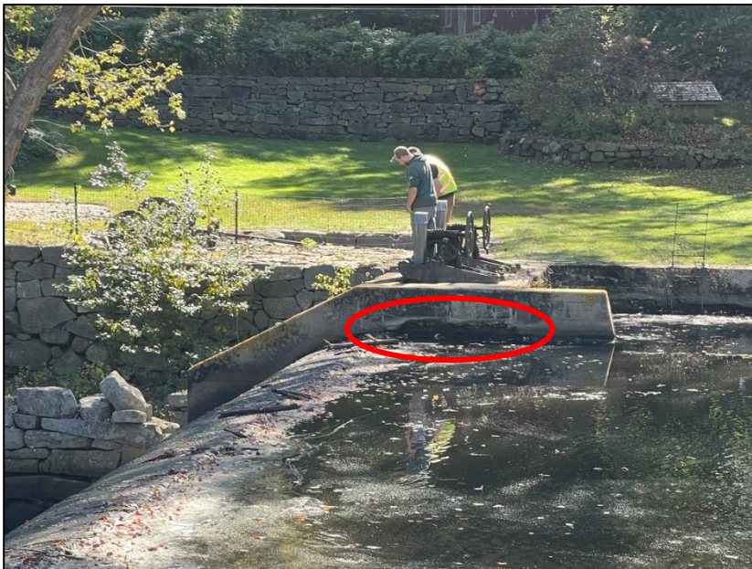
Photo No. 6.: View of the right spillway channel wall. Note scoured concrete behind the spillway crest.
