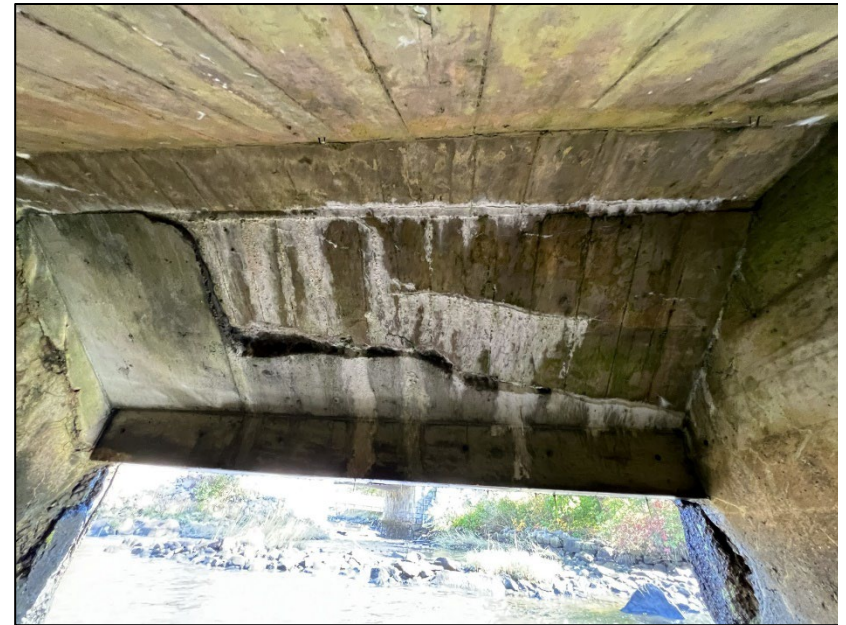
Photo No. 20.: Deterioration along the top of the concrete repair along downstream face of the ceiling (ceiling face No. 3).
