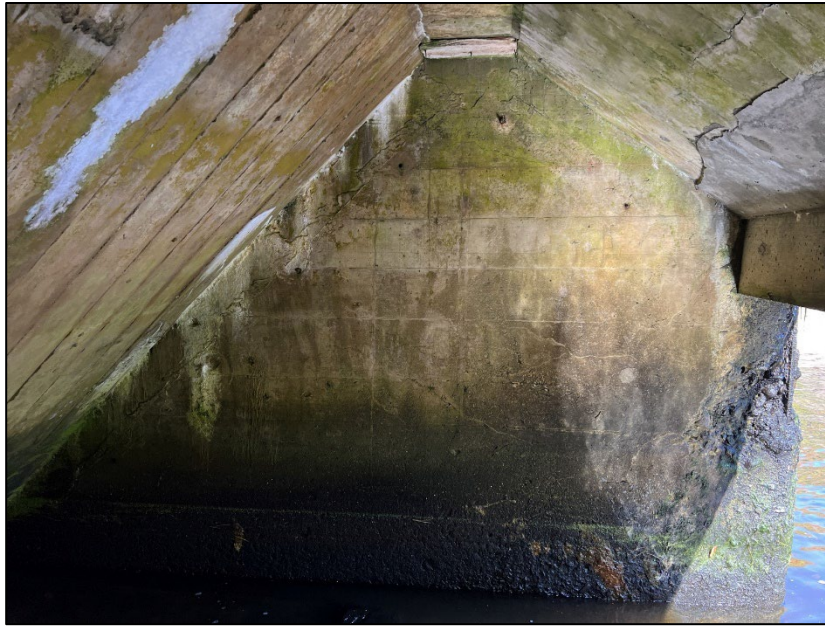
Photo No. 21.: Left Wall. Note debonded rebar and spalling on the downstream end of the wall.
