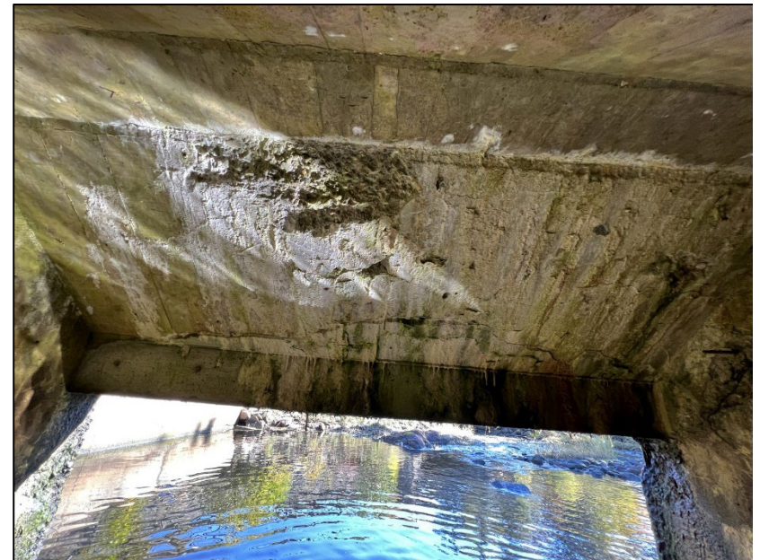
Photo No. 36.: Delamination, spalling, and efflorescence throughout the downstream sloped portion of the ceiling.
