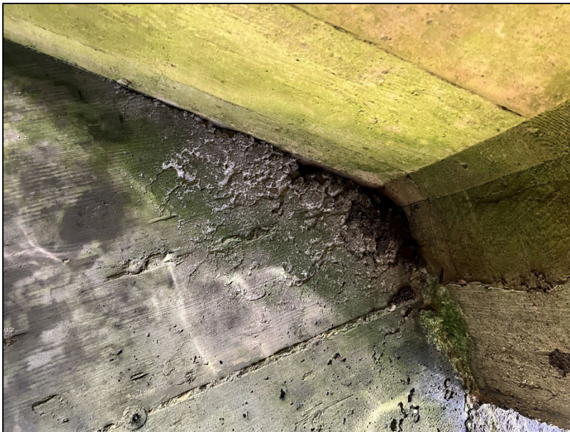
Photo No. 42.: Poor concrete consolidation at the downstream end of the left wall.
