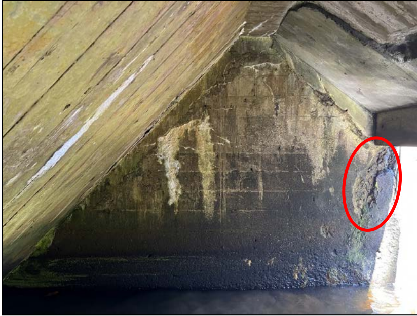
Photo No. 17.: Left Wall: Note concrete spalling on the downstream end of the wall beneath the spillway.
