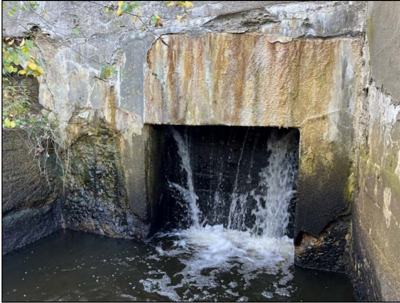
Photo No. 49.: Leakage through the low-level outlet timber gates. Note concrete deterioration throughout the downstream wall.
