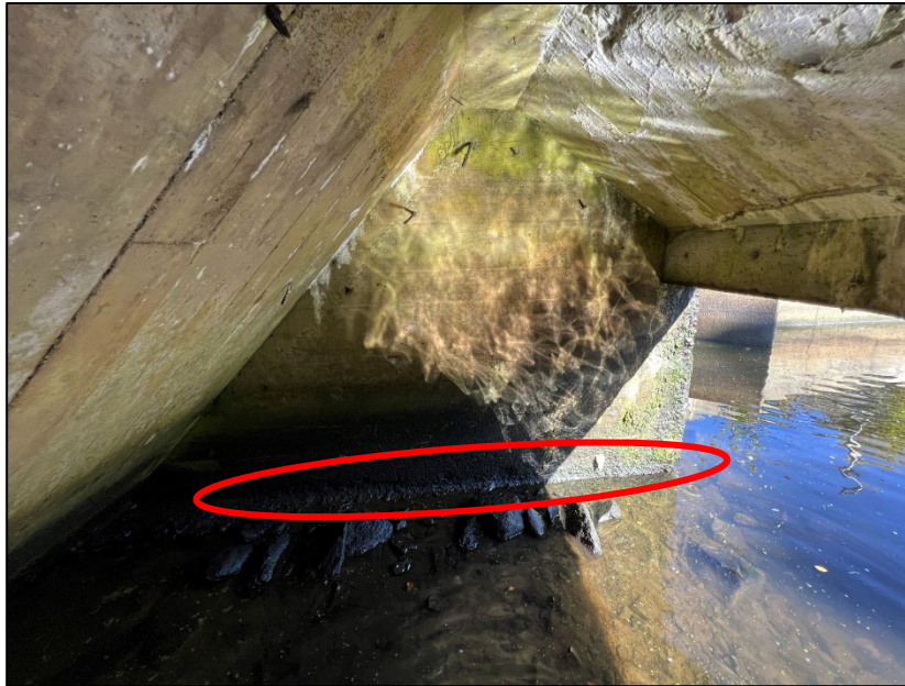
Photo No. 33.: Left Wall. Note scour up to 1.25 inches deep along the bottom 5 inches of the wall.
