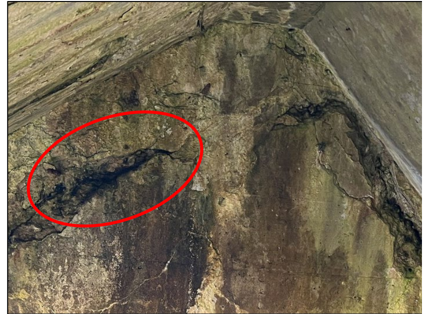
Photo No. 35.: Close-up view of the top of the deterioration of the right wall. Note location of previously noted leakage not observed during this inspection.
