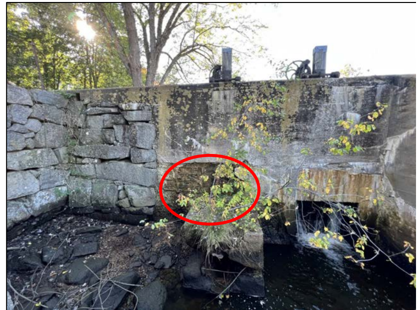
Photo No. 48.: Downstream face of the low-level outlet structure. Note further concrete smalling noted when compared to 2019 inspection report.
