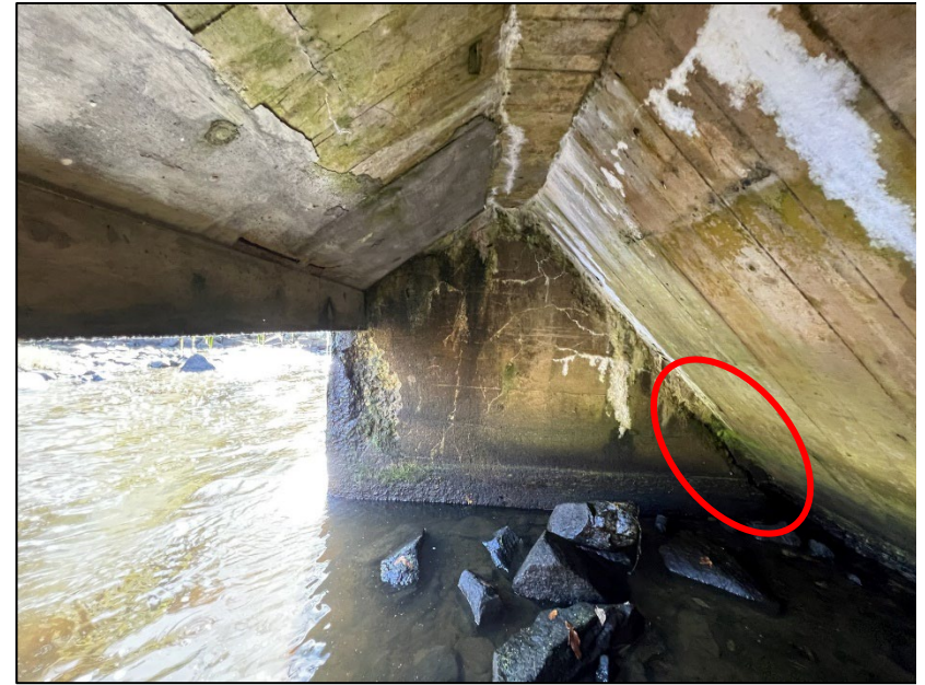
Photo No. 23.: Right wall. Note crack with 1/2" of left to right displacement.
