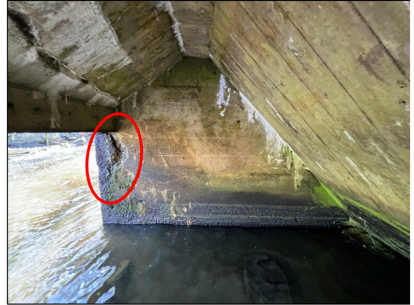
Photo No. 19.: Right wall. Note scour and spalling at the downstream end of the wall. Limited concrete deterioration was observed along ceiling face no. 5.
