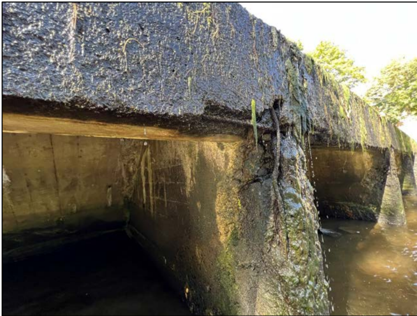
Photo No. 18.: Debonded rebar along the top of the rib between Cell 3 and Cell 4.
