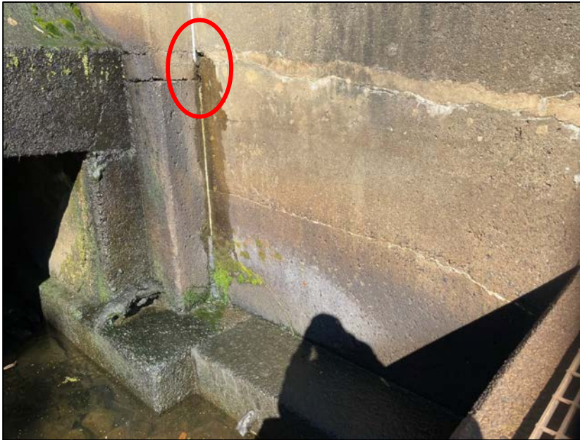
Photo No. 5.: Minor leakage between the left channel wall and the fish ladder wall.
