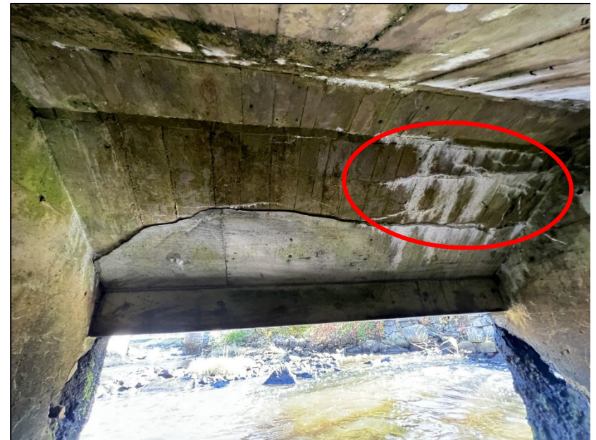
Photo No. 16.: Downstream sloped portion of the ceiling: Note delamination along the top of the concrete repair and cracking and efflorescence along the right side of the ceiling.
