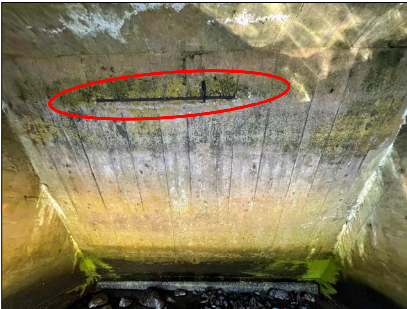
Photo No. 38.: Exposed deteriorated rebar near the top of the upstream portion of the ceiling.
