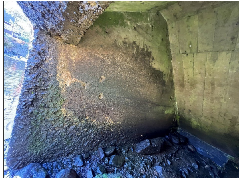
Photo No. 43.: Right wall. Note scour and concrete deterioration at the downstream end of the wall.
