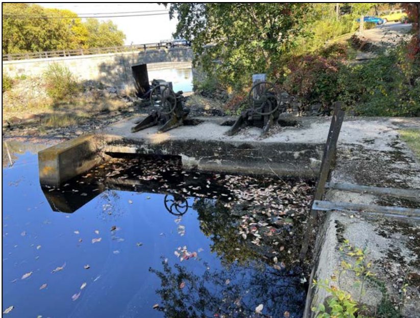
Photo No. 46.: Overview of the upstream side of the low-level outlets. Note concrete deterioration along the upstream face of the concrete wall.
