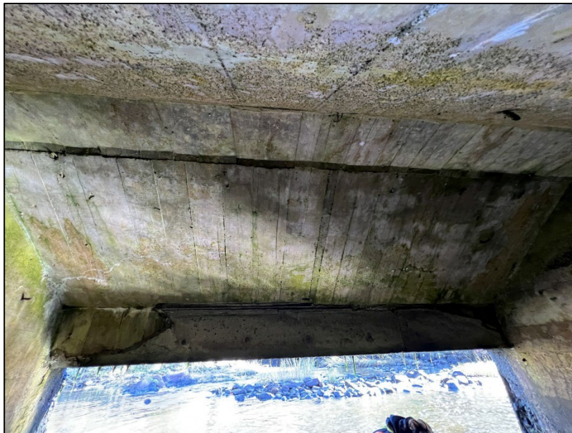
Photo No. 26.: Downstream portions of the ceiling. Note minor map cracking along ceiling face no. 3.
