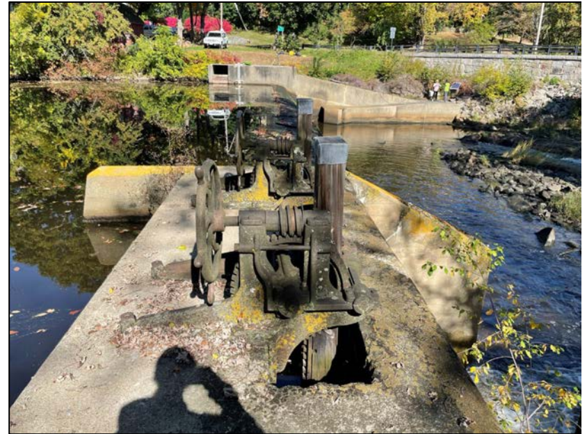
Photo No. 47.: Top of the low-level outlet control structure and gate operators.
