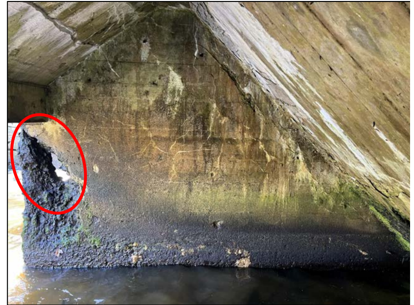
Photo No. 15.: Right wall. Note 100% section loss beneath the downstream end of the spillway. The hole pictured has continued to deteriorate since the previous inspection.
