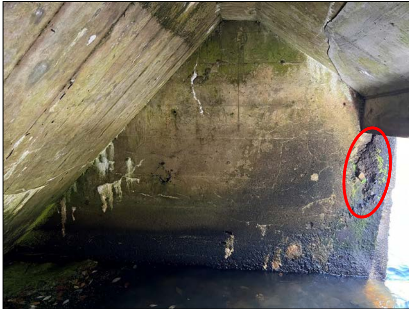
Photo No. 13.: left Wall. Note spalling and cracking beneath the downstream end of the spillway.
