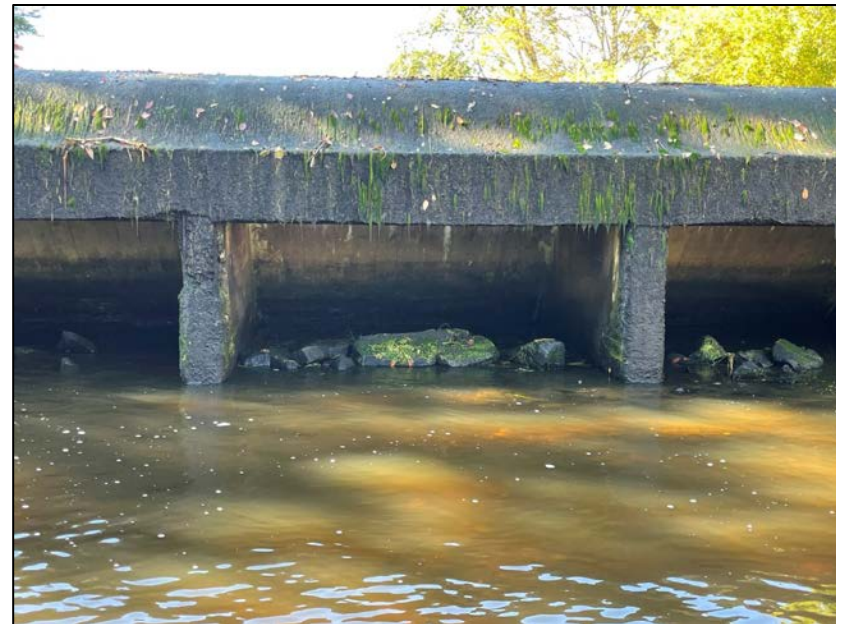
Photo No. 28.: Downstream face of the cell. Note the exposed rebar extending from the top of the stem between Cell 5 and Cell 4 to the mid-height of the stem.
