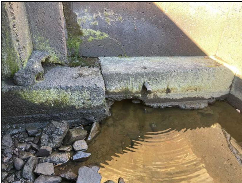
Photo No. 54.: Scour hole at bottom of right fish ladder wall at the downstream channel. Note void was probed approximately 36 inches.
