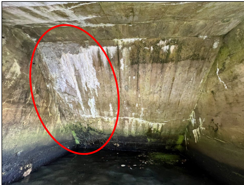
Photo No. 14.: Delamination and concrete deterioration along the right (photo left) portion of the upstream sloped ceiling (ceiling face no. 5).
