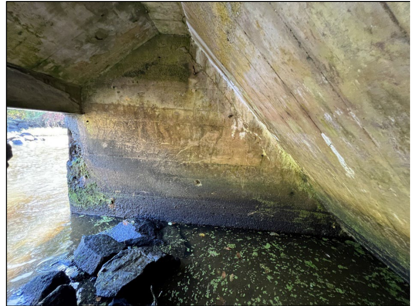
Photo No. 27.: Right Wall. Note debonded rebar and spalling at the downstream end of the wall.
