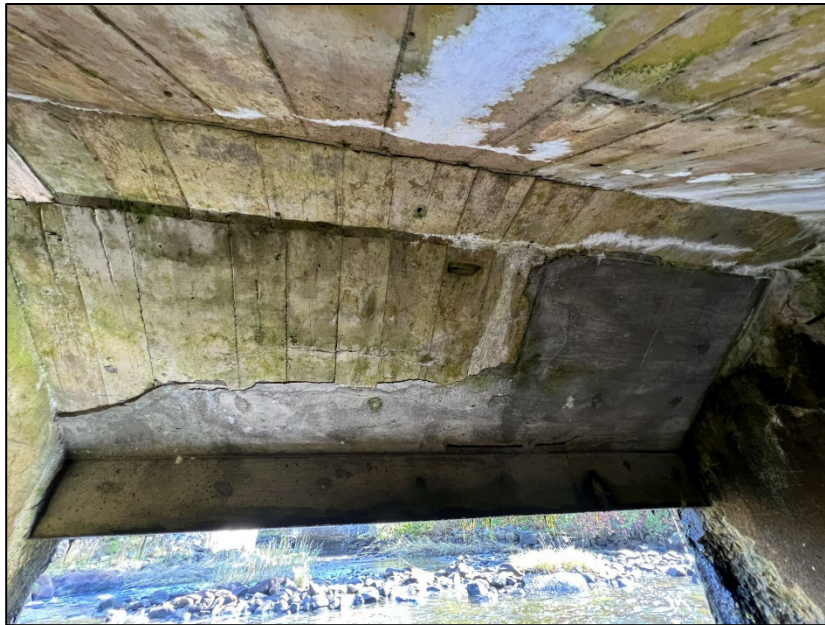
Photo No. 22.: Overview of the downstream slope of the ceiling (ceiling face no. 3).
