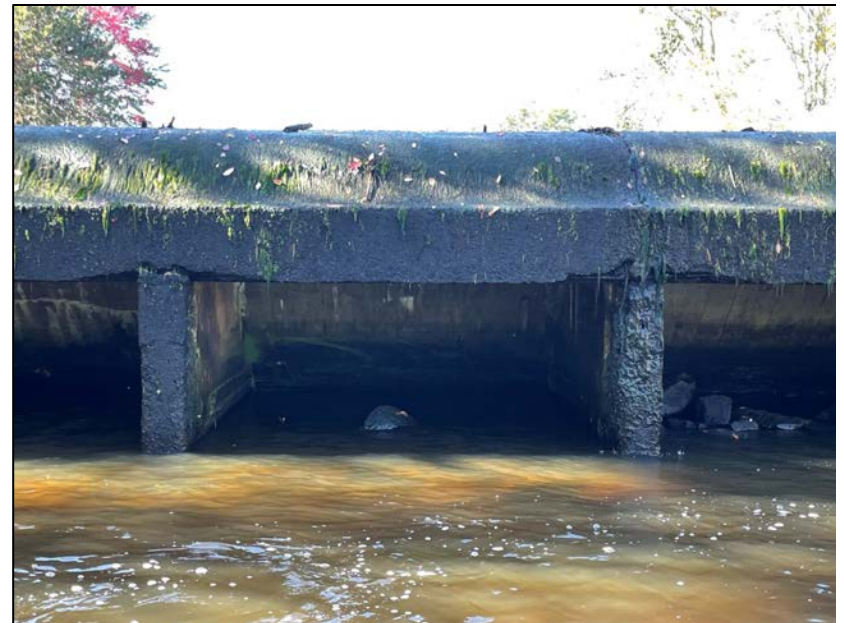
Photo No. 8.: Close-up view and typical downstream face conditions of the spillway cells.
