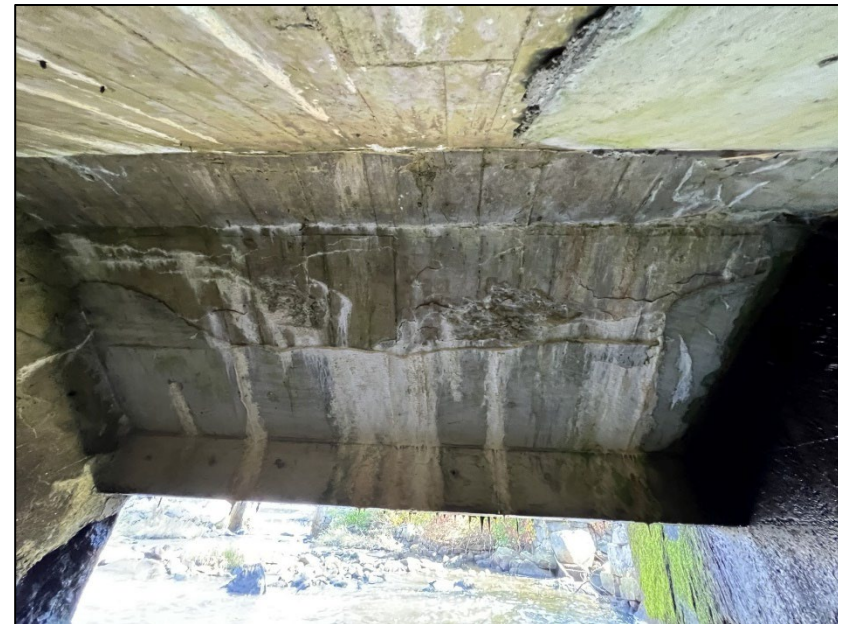
Photo No. 12.: Repair along the downstream sloped ceiling section (ceiling face No. 3). Note delamination above the repair with efflorescence staining.
