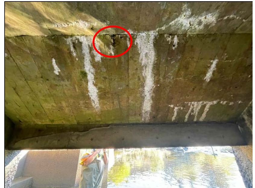
Photo No. 40.: Exposed deteriorated rebar and concrete spall on the downstream sloped portion of the ceiling.
