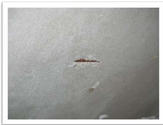
Concrete Spall at Underside of Deck
