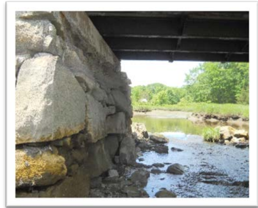
Bulging at West Abutment
