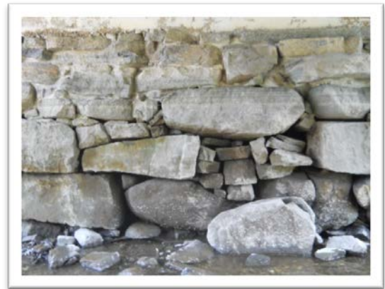
Bulging at West Abutment
