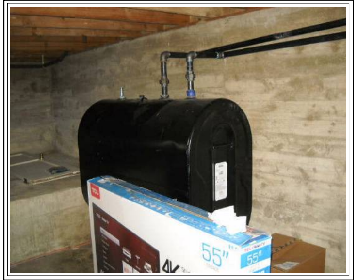
Basement, Oil Tank
