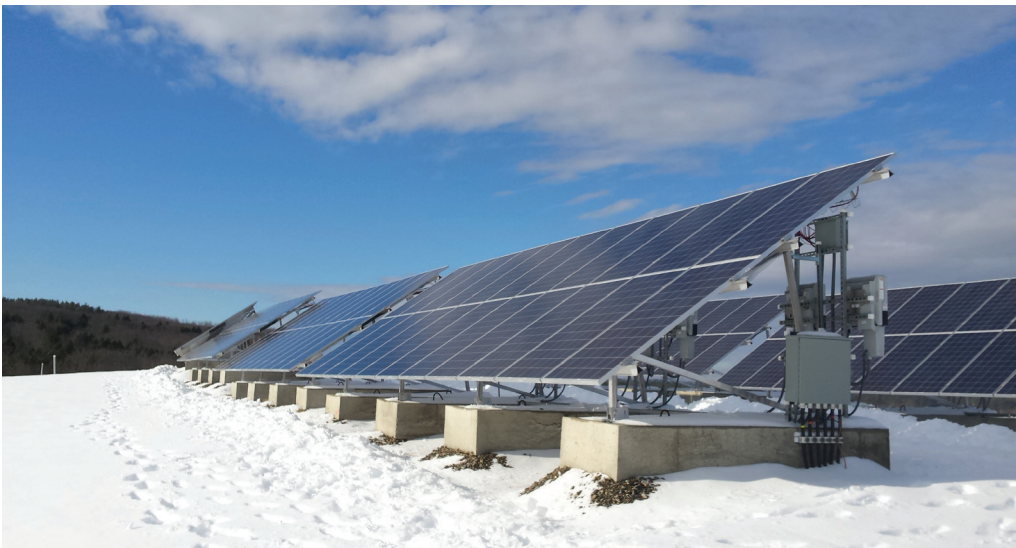
Solar panels working efficiently throughout the winter in an array for the City of Belfast in Maine. Low temperatures don't stop panels from converting available sunlight to power.
