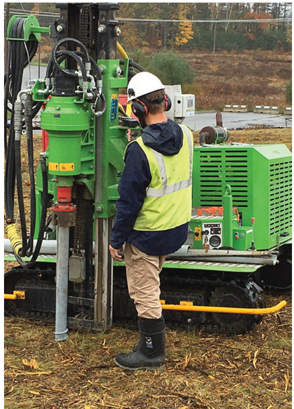
A member of our newly-formed Solar Foundations Division driving a groundscrew into place with our Pauselli 900 pile driver.
