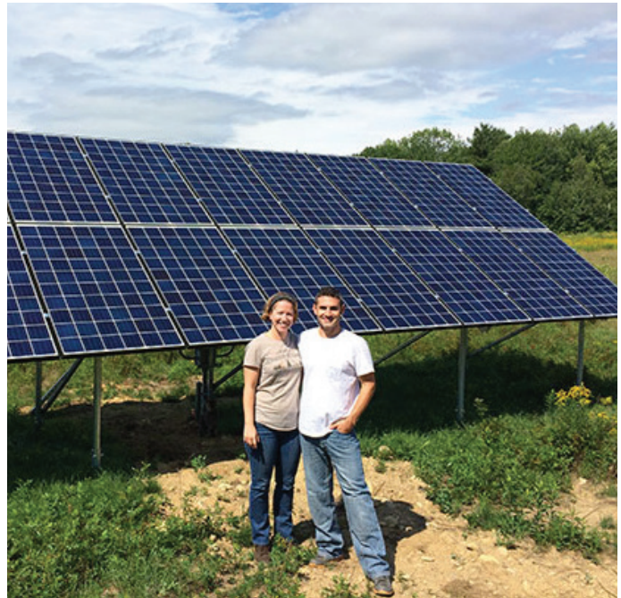
Solar homeowners Lauren and Nate Zike in front of their 5.83 kW solar electric array. Their solar array will meet close to 100% of their energy needs, allowing them to control their energy costs, all while helping to reduce strain on the local energy grid and reducing pollution from fossil fuel sources.
