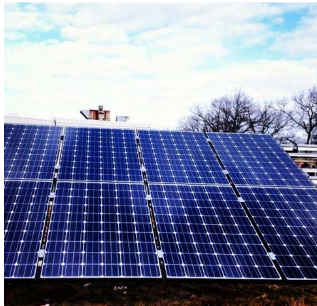
Completed installation showing gaps between panels
