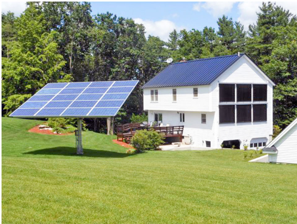
Tracker Mounted Residential System: Courtesy Revision Energy
