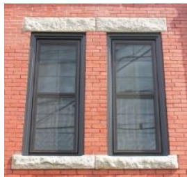
All windows in masonry buildings shall have a distinct lintel over the windows, providing structural, or at least convincing visual, support to the window opening. (86)
