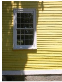
The narrow clapboards brings an intimate scale to the main structure of the Three Chimney's Inn (46)
