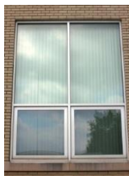
There is no lintel, or special treatment, over this window, so it appears that the brick above would simply collapse. (95)
