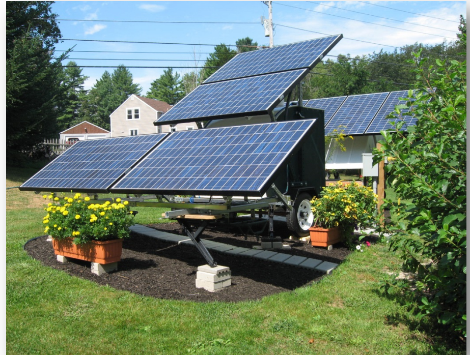
Photo 5: Locally Installed Solar Panels (Photo Credit: Jack Palmer)
