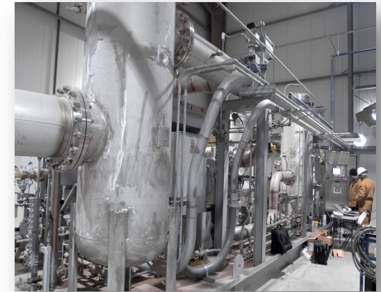
Photo 6: Processing Plant at Waste Management Turnkey Recycling and Environmental Enterprise (TREE)
