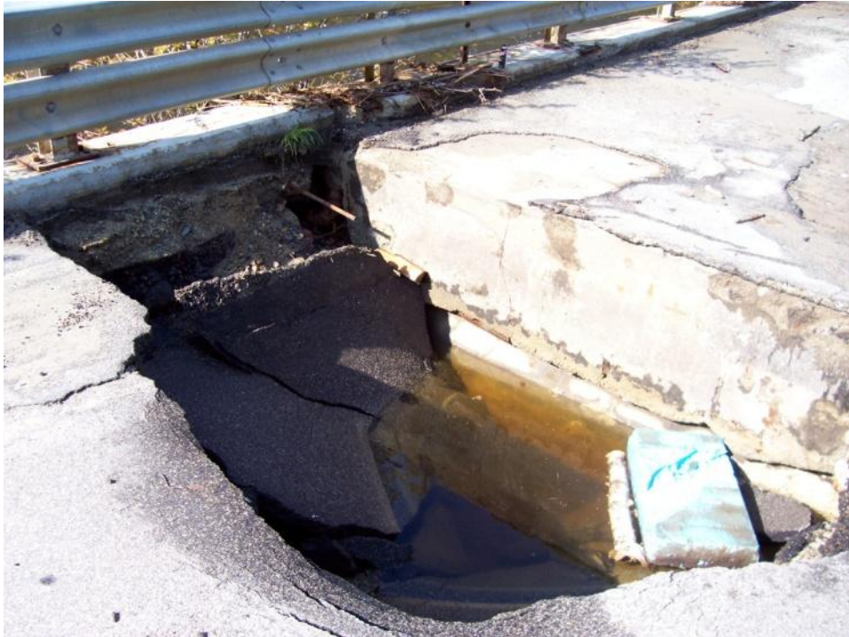
Wiswall Bridge, May 2006 Flood
