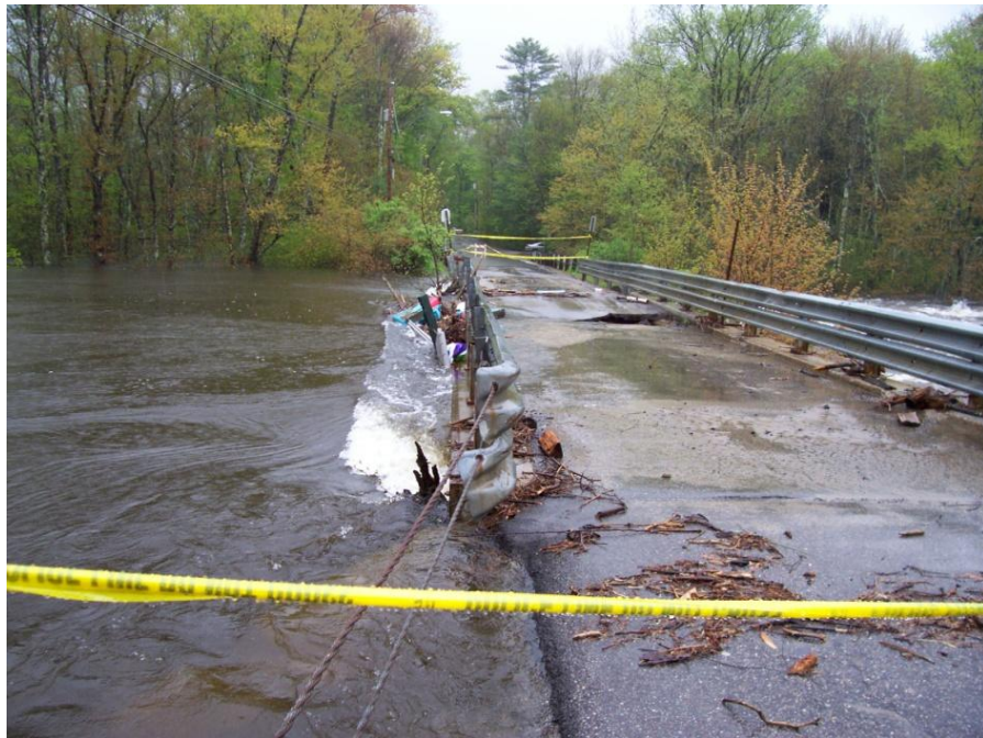
Wiswall Bridge suffered a collapse of the center pier during the May 2006 Flood Event.
