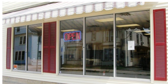
The base/bulkhead is too low and the expanse of large glass panes is too extensive. (136)
