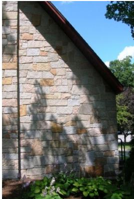
Only natural stone shall be used, as in St. George's Church. Stone shall be laid in roughly horizontal patterns or it will have an artificial wallpaper quality. (118)
