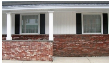
Multicolor, salvage-style brick is not appropriate. (123)
