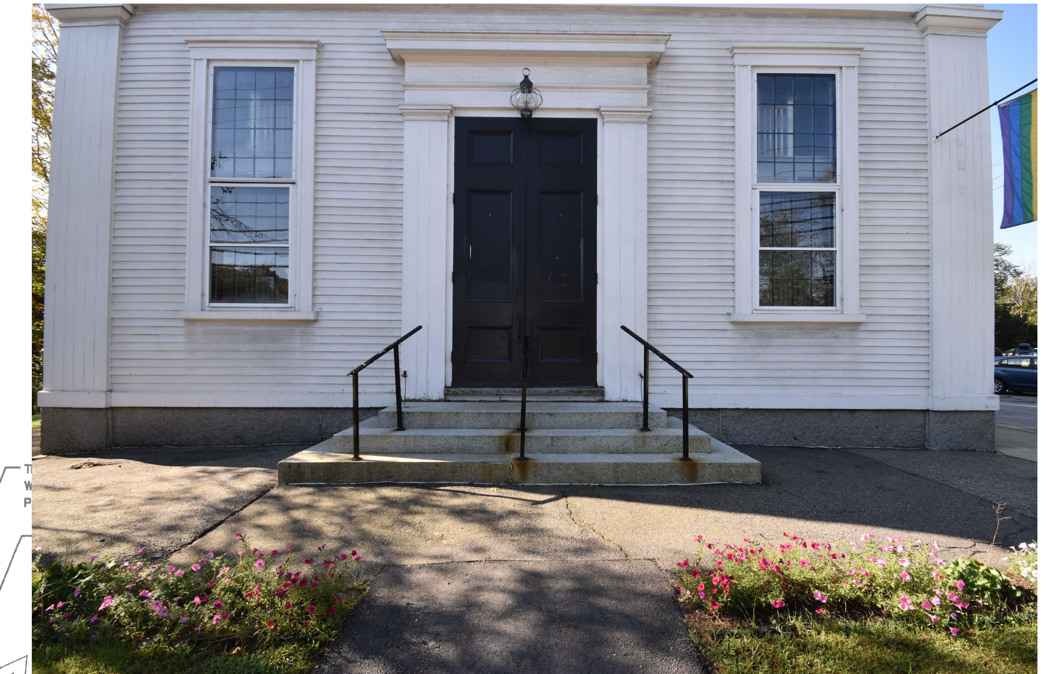
Image of Affected Pavement & Landscaping
