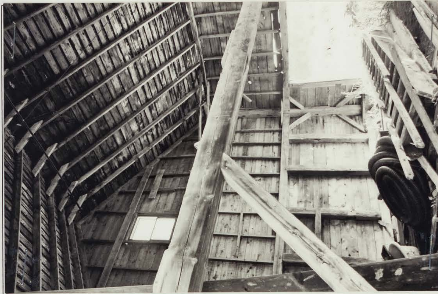
Photo 10 description: Interior framing of barn, looking at NE corner of building Roll: 1 Frame: 11 Direction: NE
