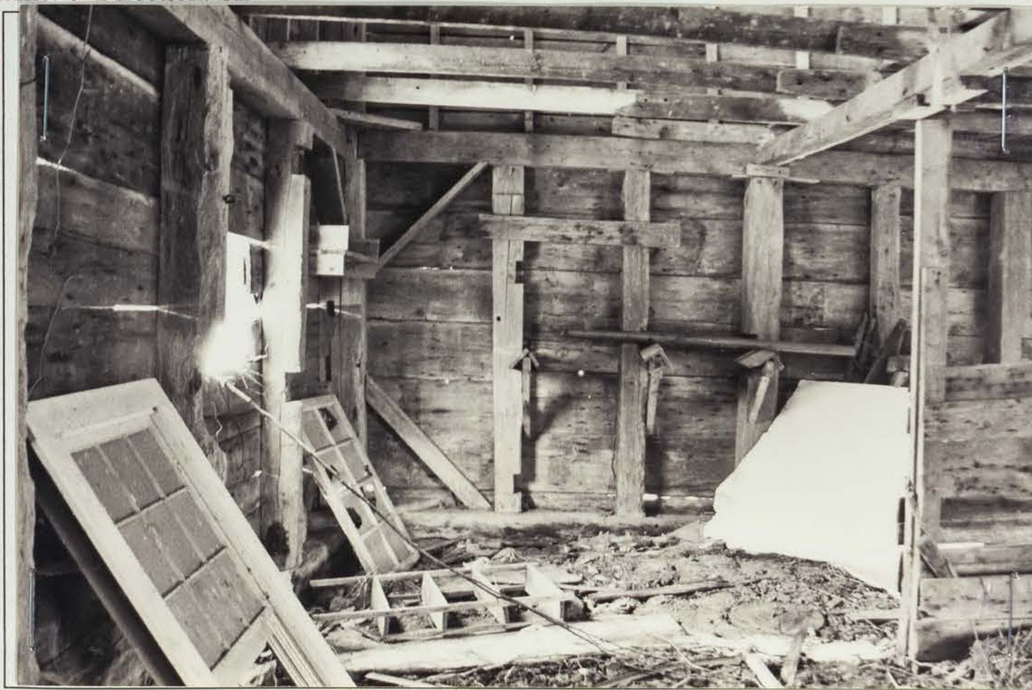
Photo 15 description: Looking at west (eaves) wall in south bay Roll: 3 Frame: 9 Direction: W Address: 97 Newmarket Road Date taken: October 2004-January 2005 Negative stored at: NHDHR
