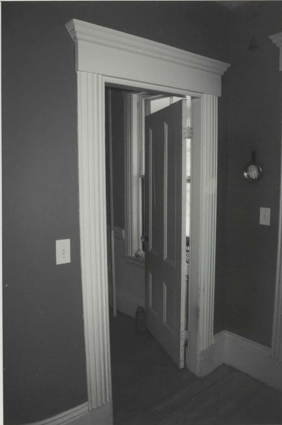
Photo 8. First-floor doorway from central stairhall looking into north-side parlor; note 4-panel door. Looking: NE Image file: DUR000_08
