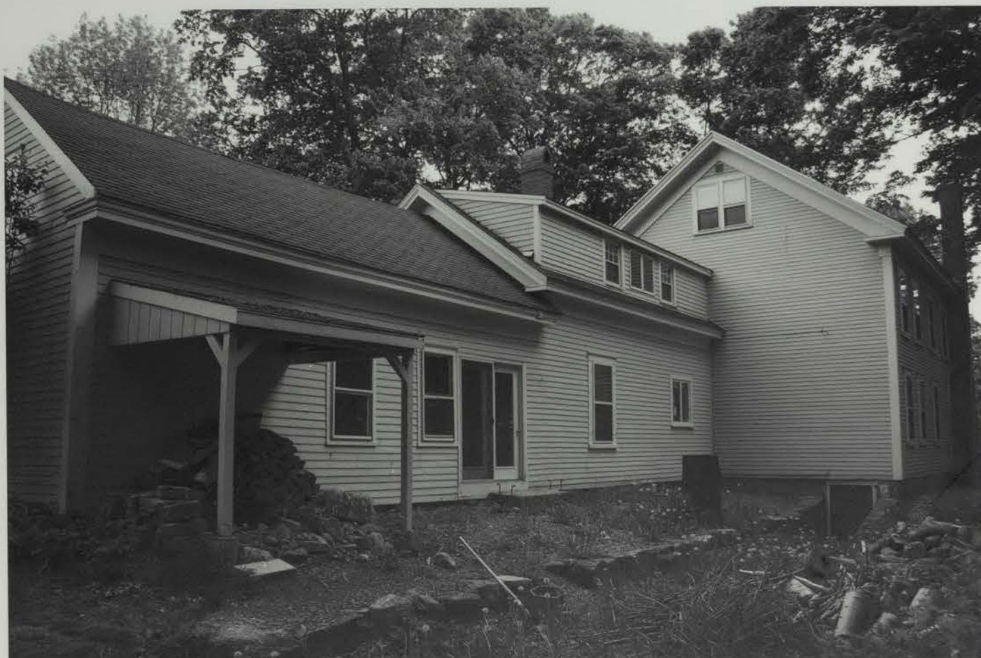
Photo 5. Rear (north) side of house; shed dormer on kitchen wing is later addition. Looking: SE Image file: DUR000_05
