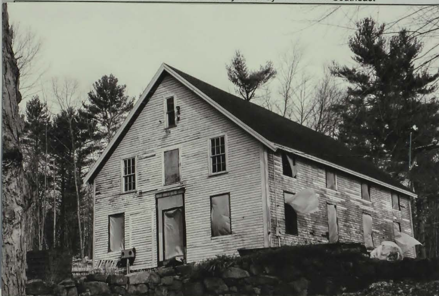
Photo # 19 Description: Cider mill has recently been gutted because of water damage due to leaking roof. Reference (file name or frame#):: Cyderhouse 2016 Direction: Northwest
