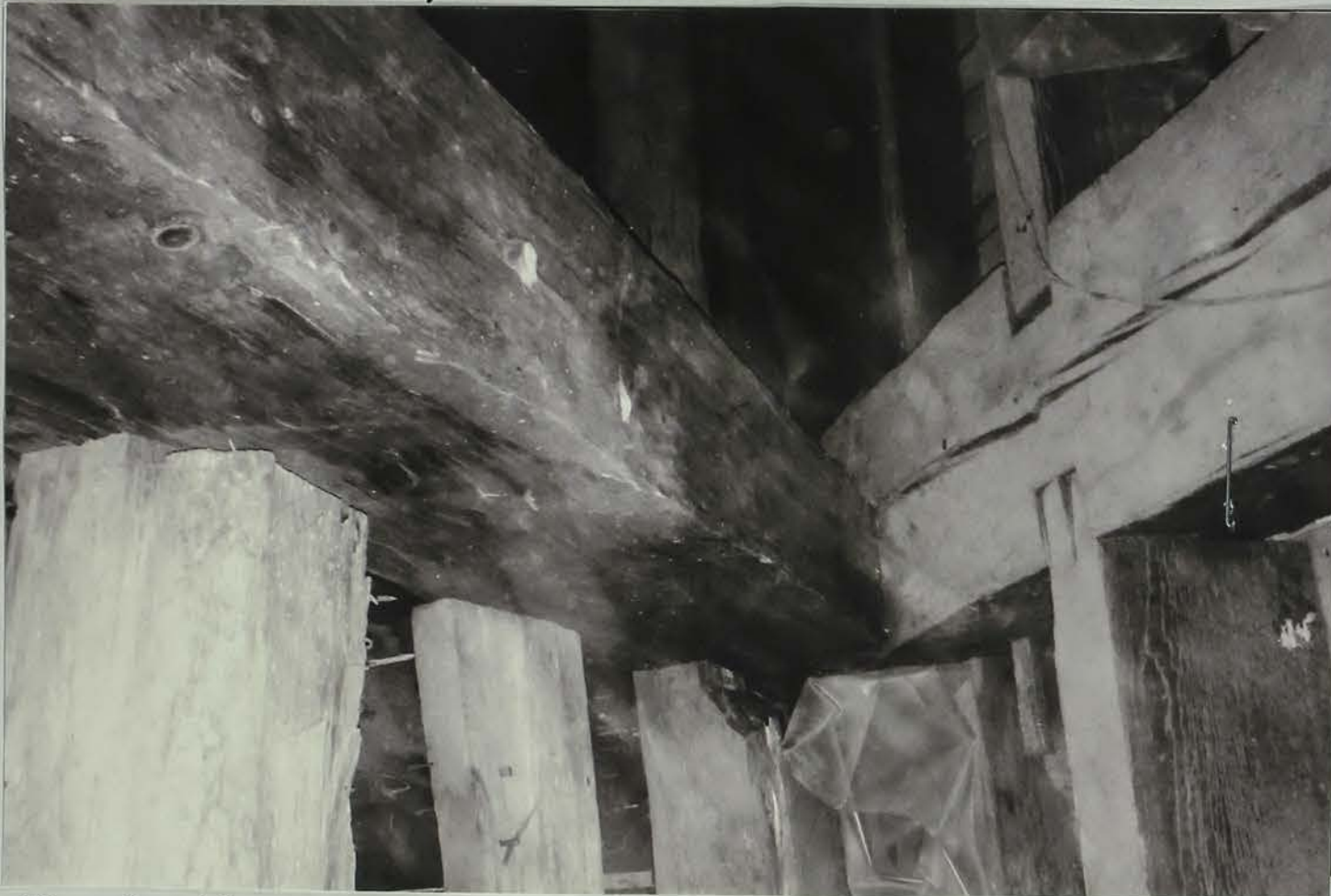
Photo # 33 Description: Timberframe construction in attic roof. Reference (file name or frame#):: Mortise and Tenon in Attic Direction: South
