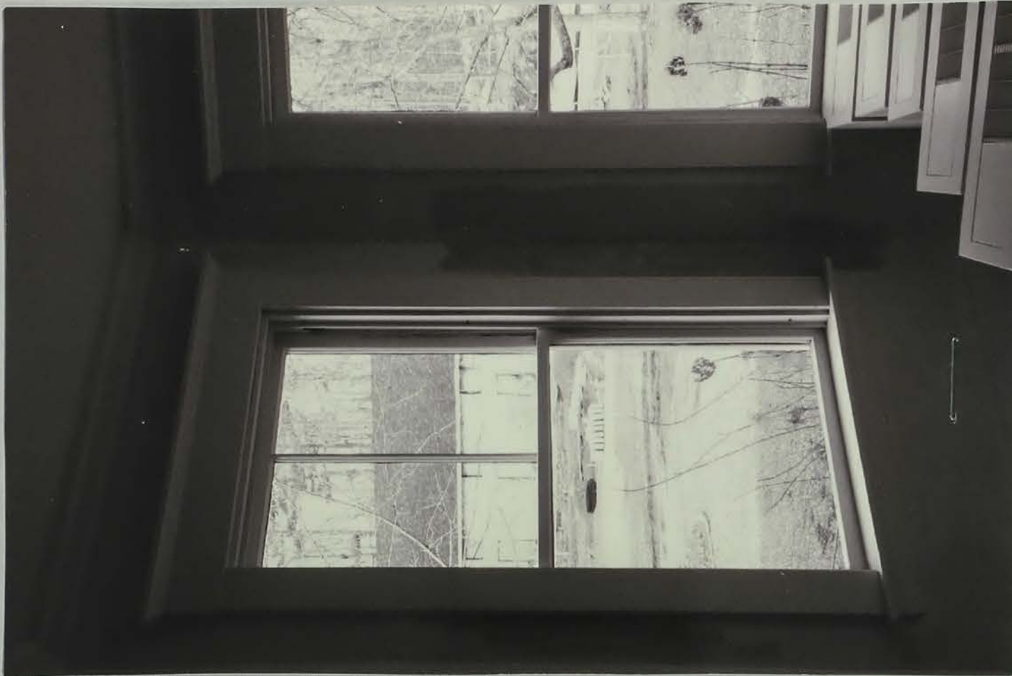
Photo # 34 Description: Example of first floor window trim with cornice molding. Reference (file name or frame#):: Interior Window detail Direction: West
