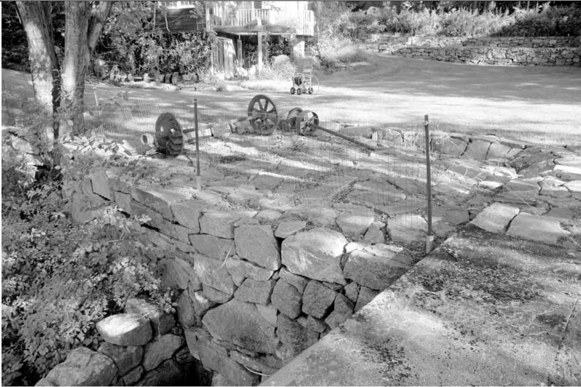
Photo 20: Stone patio drain, mill foundation wall, rebuilt ca. 2007, rear of 20 Newmarket Road in back Direction: SE
