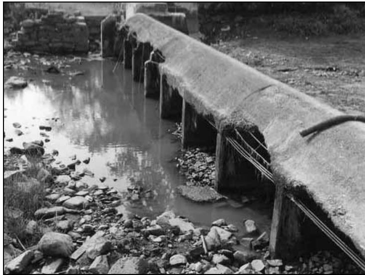
1974 before repairs, facing SSW (Durham Historic Association)
