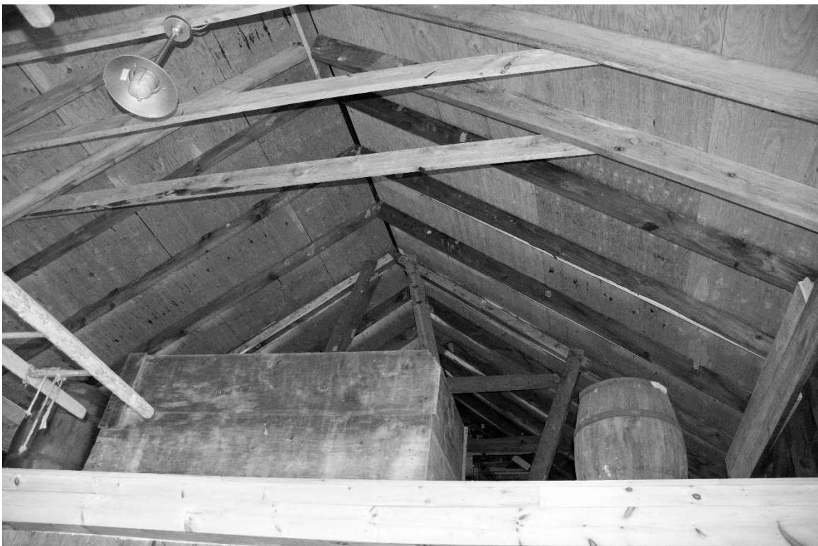
Photo 44) ell attic, showing junction of old and rebuilt roof Reference (file name): PIC_0639
