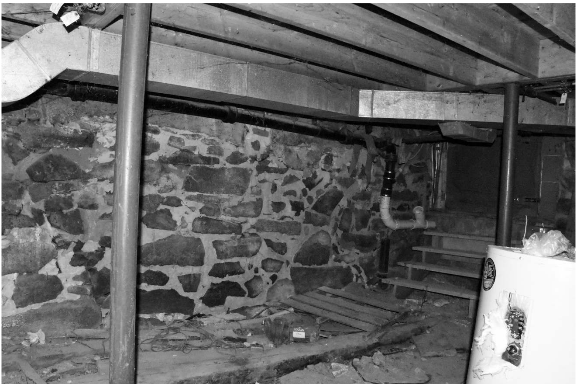
Photo 35) south foundation wall and rebuilt kitchen floor framing looking toward bulkhead Reference (file name): PIC_1870
