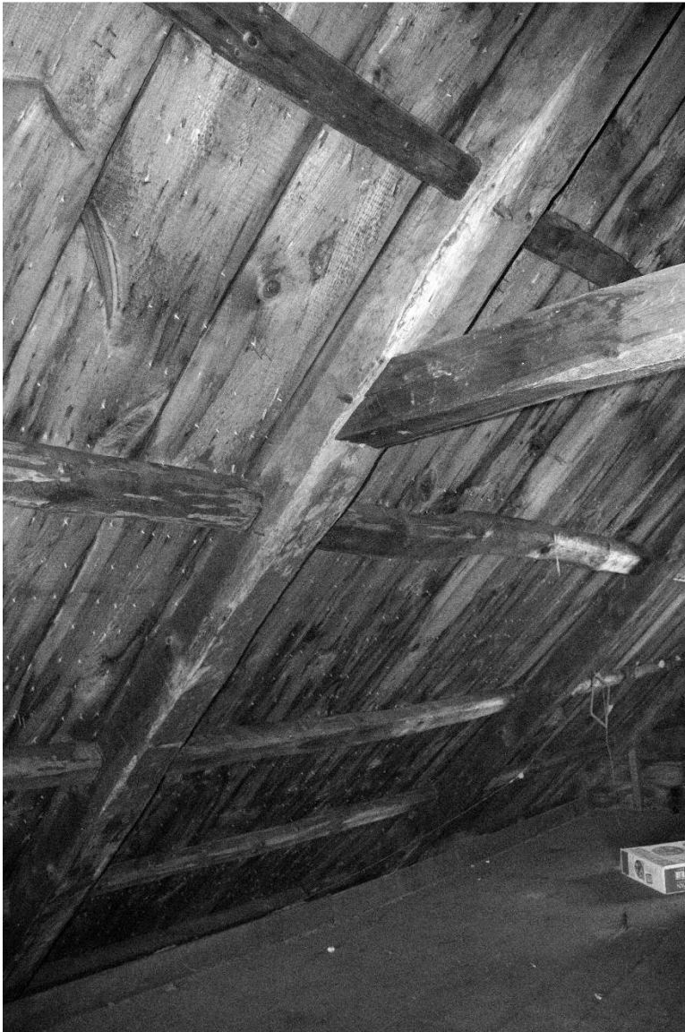
Photo 42) roof framing detail showing pegs and scribe marks Reference (file name): PIC_0611
