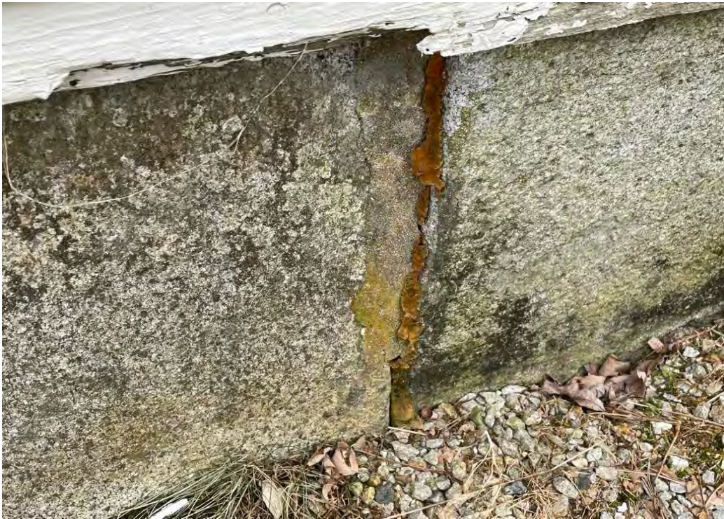
Image 44: Detail of foundation stone joint showing typical mortar loss and Spray foam repair.
