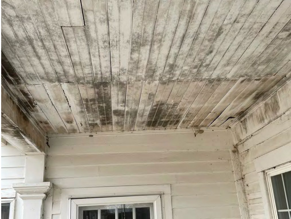
Image 41: Detail of the porch ceiling looking west, showing mold growth and warping due to past water infiltration.
