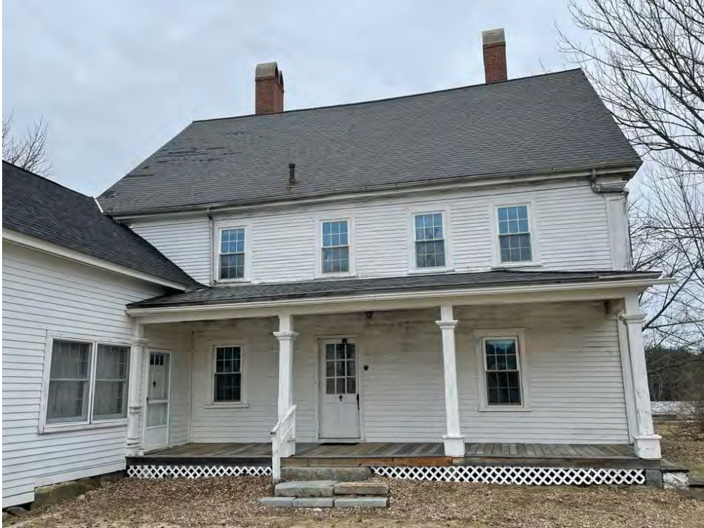
Image 39: View of the porch looking north, showing downward settling to the east.
