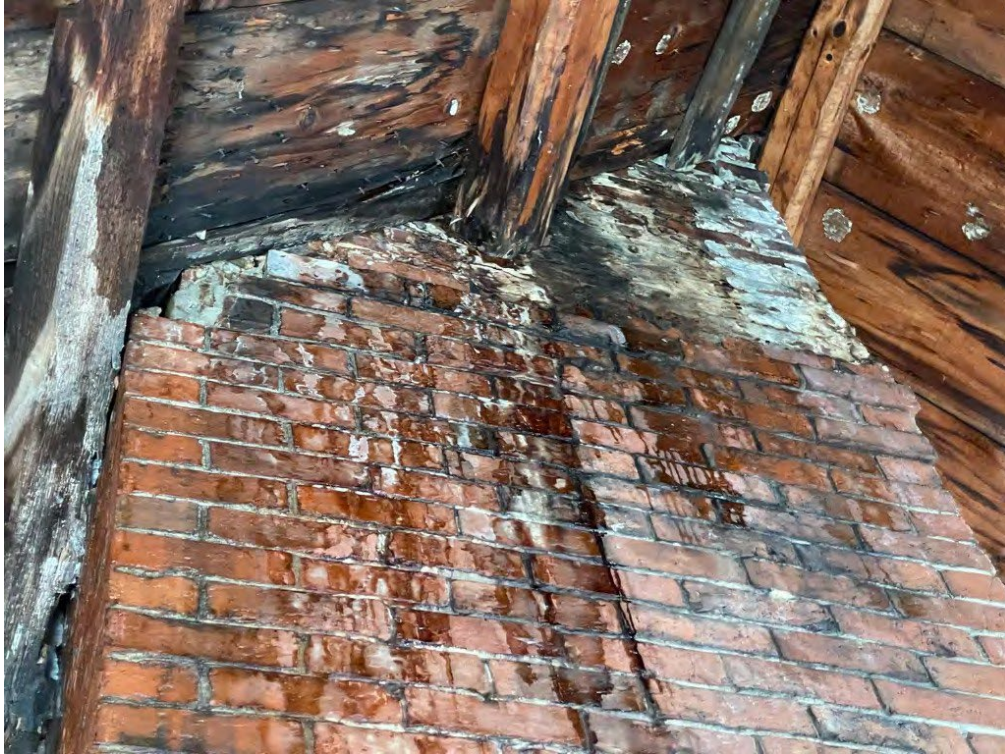
Image 35: Detail of east chimney showing the stack extension on top of the original corbel, and old water staining.
