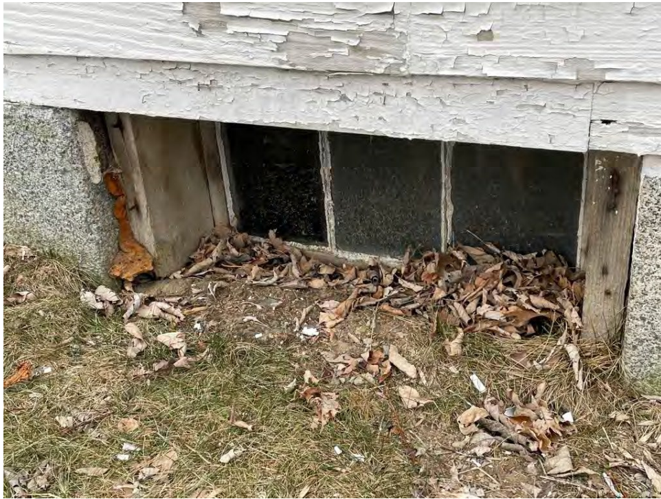
Image 51: Detail of a basement window, east elevation, showing encroaching grade and decay of the window elements.
