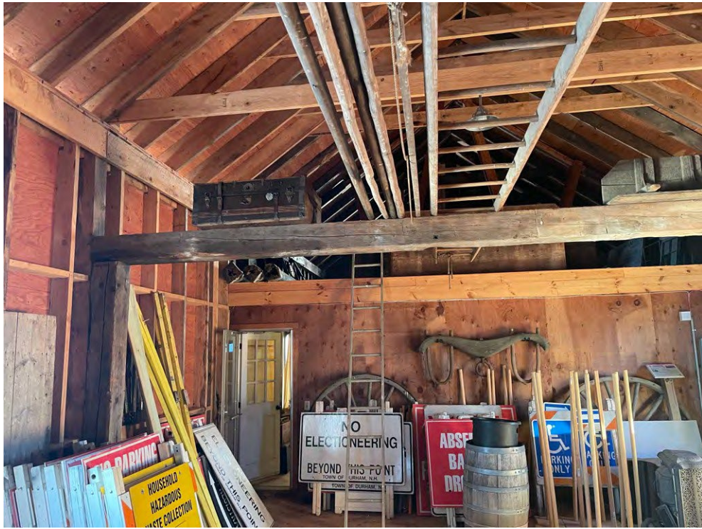
Image 17: View of the roof framing of the original portion of the ell looking north from the modern portion of the ell.
