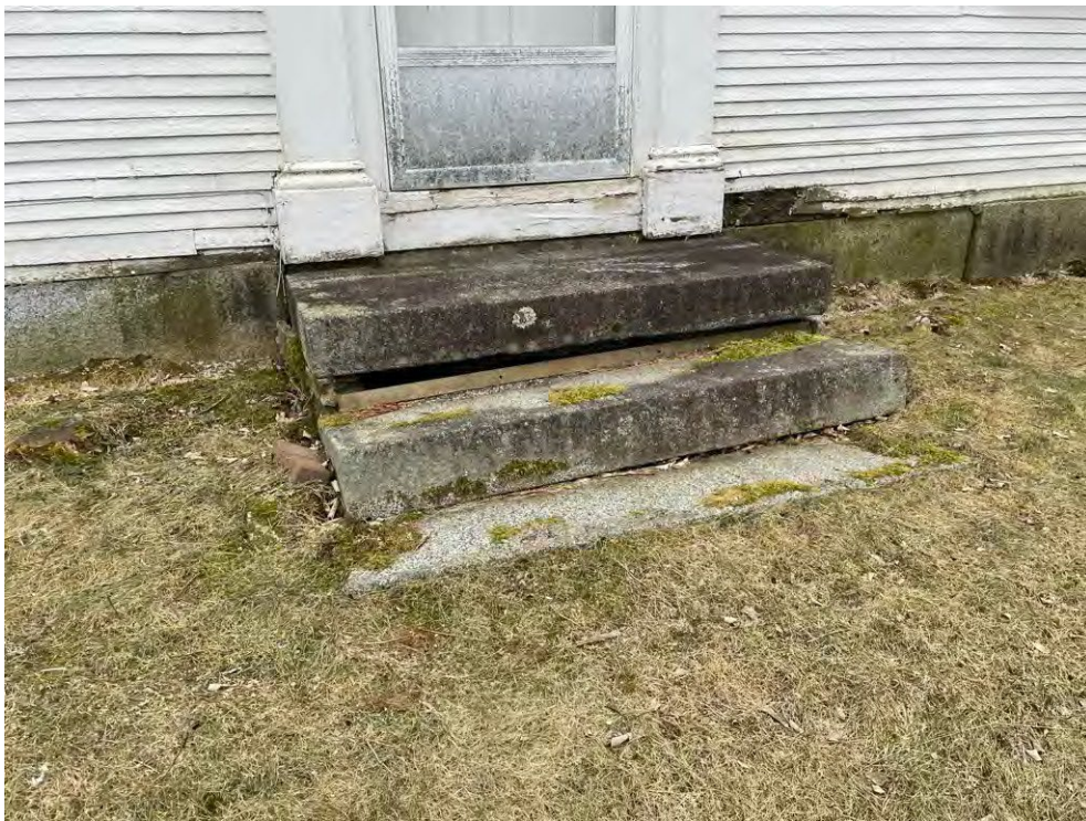
Image 38: Detail of the front entrance showing decay in original wooden elements and deflection of the stone steps.
