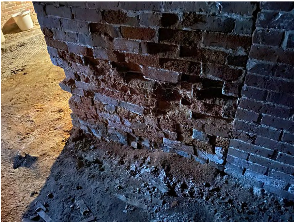
Image 42: Detail of the west chimney base in the basement showing typical brick deterioration from rising damp.
