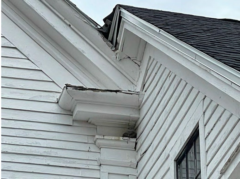
Image 37: Detail of cornice return and intersection of the main house to the ell, west elevation, showing water-related damage due to poor flashing and drainage.
