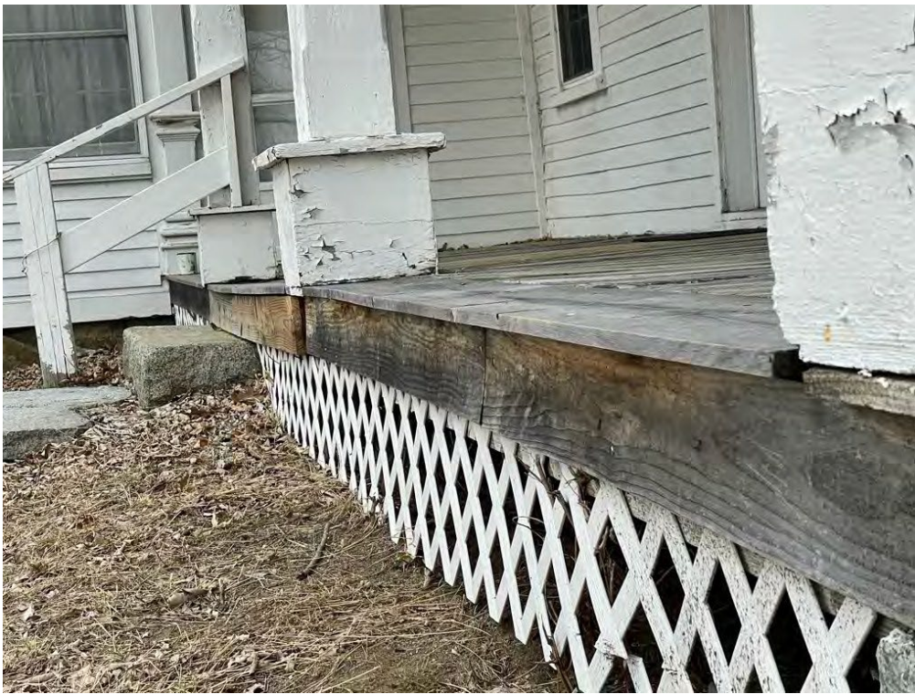
Image 40: Detail of the porch showing downward settling and decay of wooden elements.
