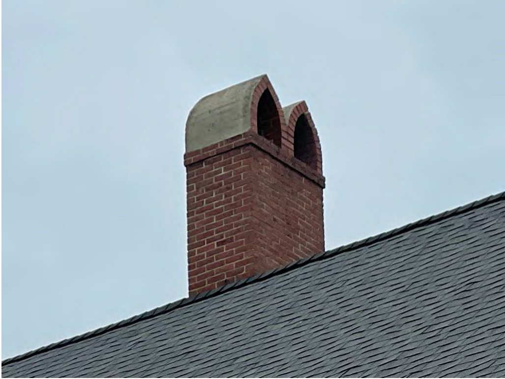
Image 43: View of the east chimney stack looking southwest, showing typical, minor mortar loss.
