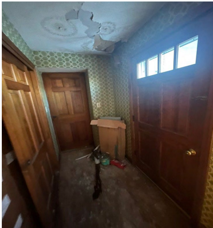
Image 50: View of the entrance to the ell apartment showing collapsed drywall from a past leak.
