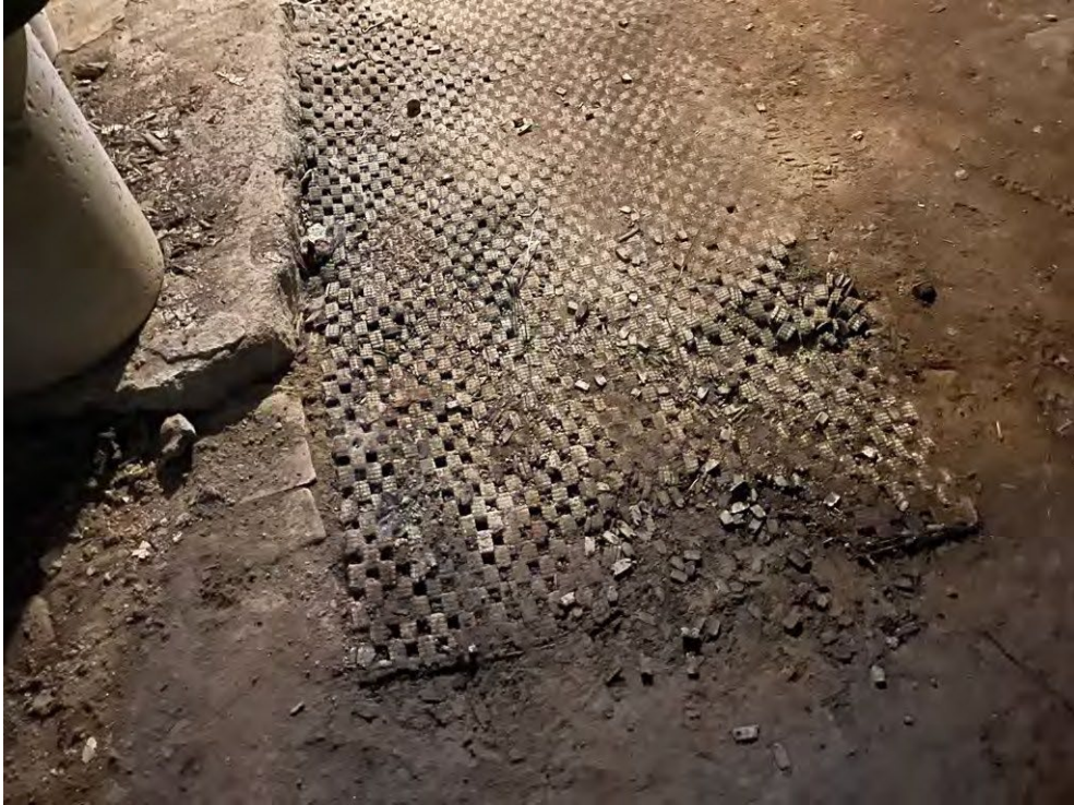
Image 49: Detail of the basement floor showing compacted soil from past water infiltration, and degraded floor mats.
