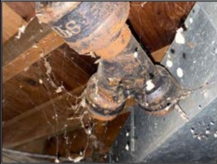
Surface rusting on cast iron drains Rusting on cast iron unions
