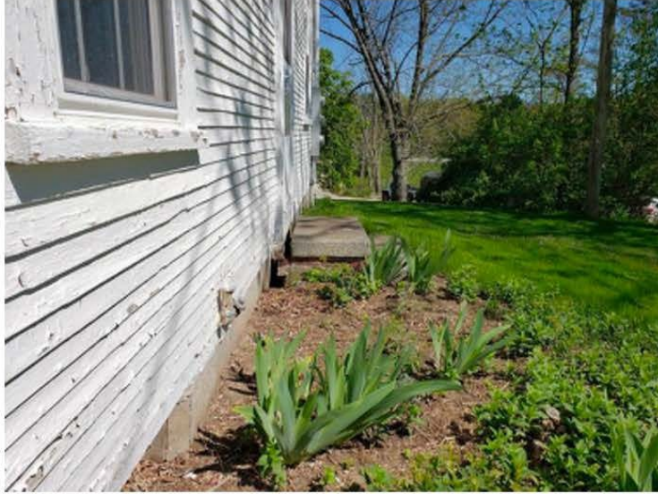
Photo 7 Shifted stones at east entry of main house (facing north)
