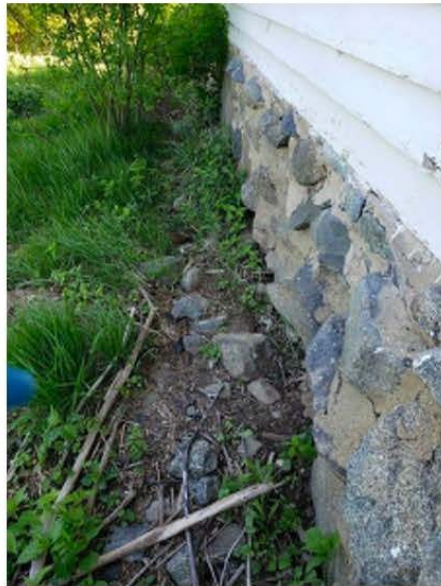
Photo 8 Foundation buckling inward at west wall of ell (facing north)
