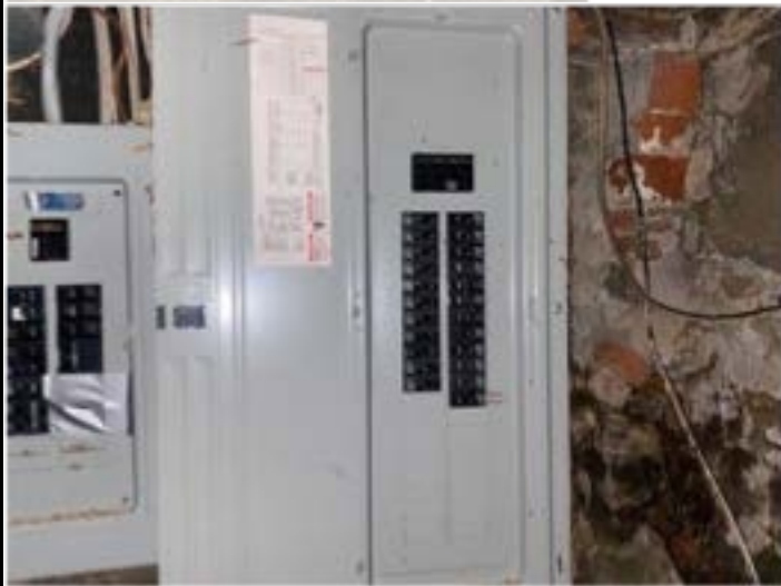
House panel with cover removed
