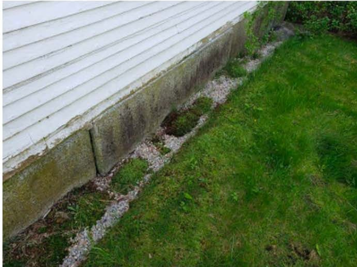
Photo 3 Shifted stones at north elevation of main house (facing southwest)
