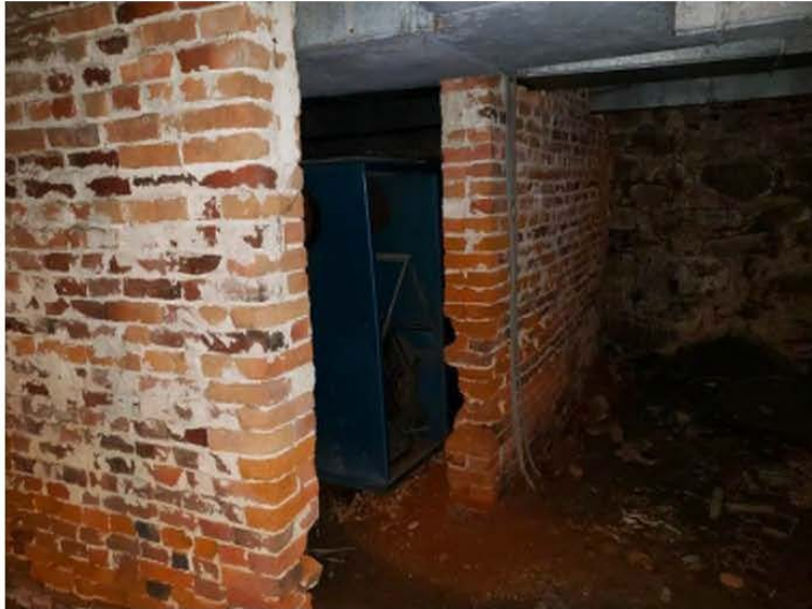
Photo 11 Deteriorated bases of brick walls
