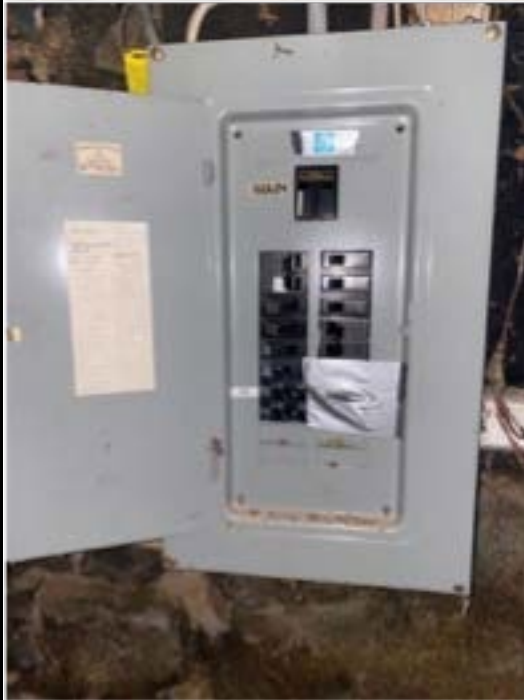
"Garden" panel with cover removed
