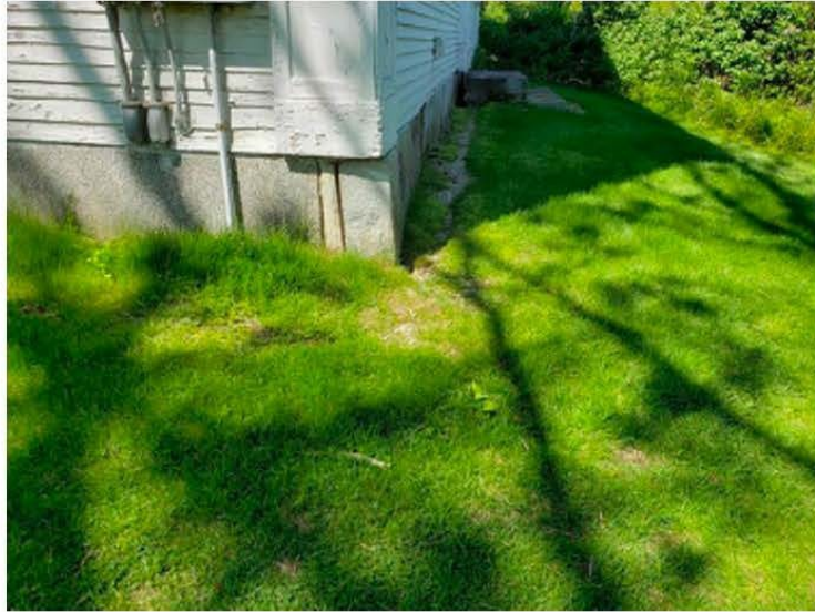
Photo 5 Shifted stones at northeast corner of main house (facing west)
