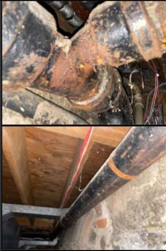
Heavy rusting at union Example of rusting in drain lines
