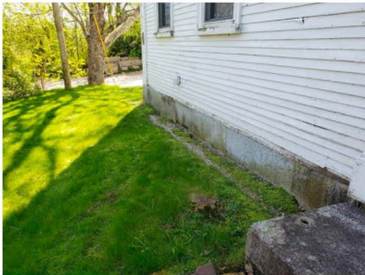
Photo 4 Shifted stones at north elevation of main house (facing southeast)
