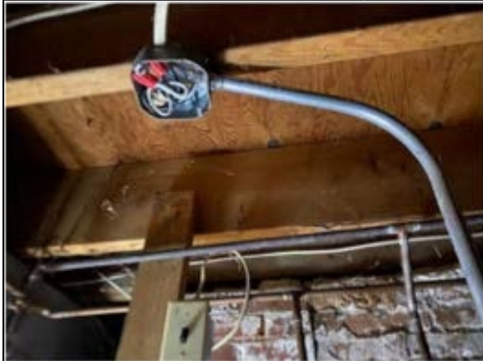
Example of open junction box
