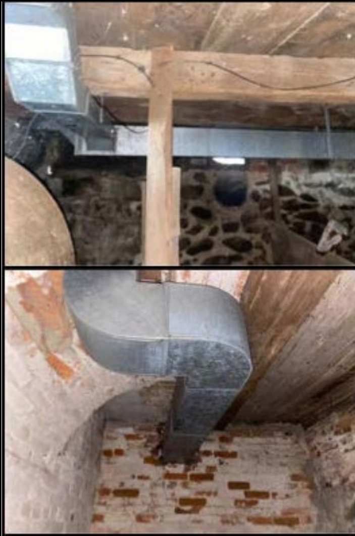
Furnace duct work uninsulated Furnace duct work uninsulated
