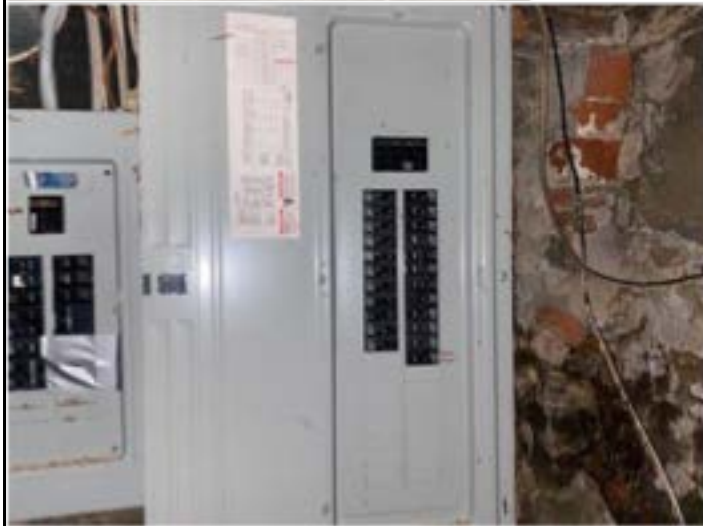
House panel with cover removed
