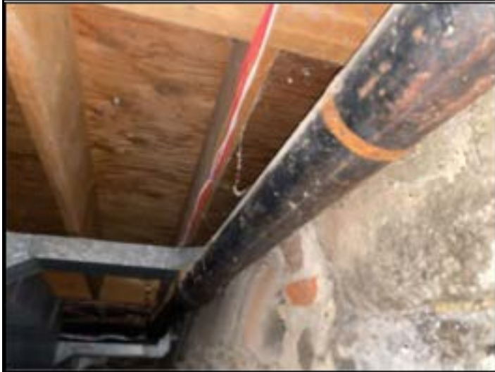
Heavy rusting at union Example of rusting in drain lines
