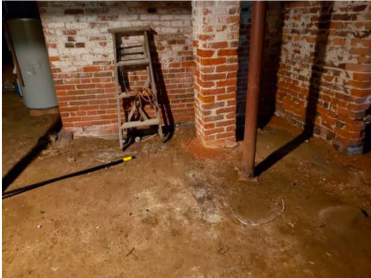
Photo 10 Corroded column base and deteriorated bases of brick walls and pier
