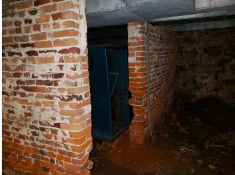
Photo 11 Deteriorated bases of brick walls
