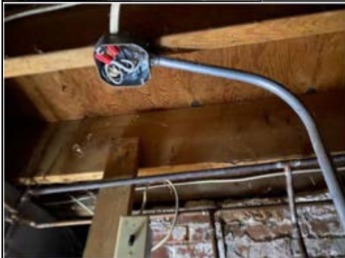
Example of open junction box
