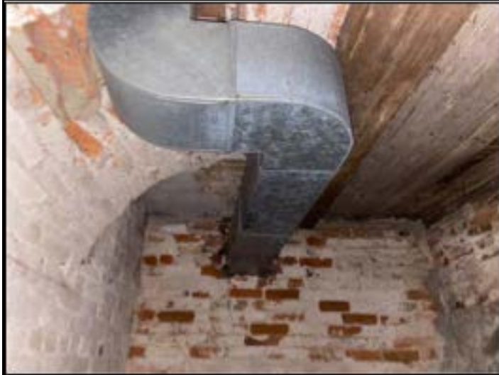
Furnace duct work uninsulated Furnace duct work uninsulated
