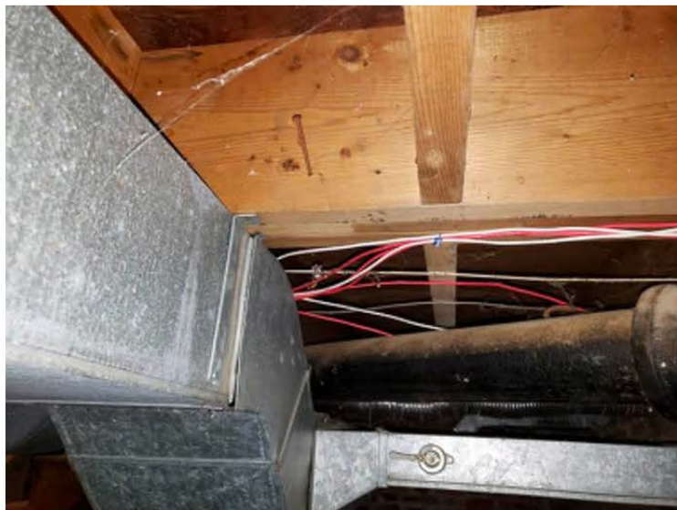
Photo 16 Reframed area at southwest corner of main house lacking hangers at common joists, beam is improperly spliced
