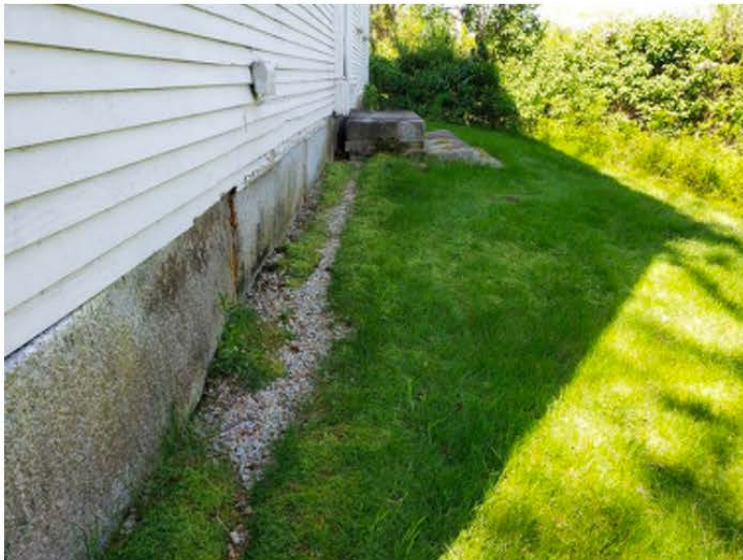
Photo 6 Shifted stones at north elevation, including steps (facing west)
