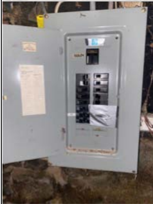
"Garden" panel with cover removed
