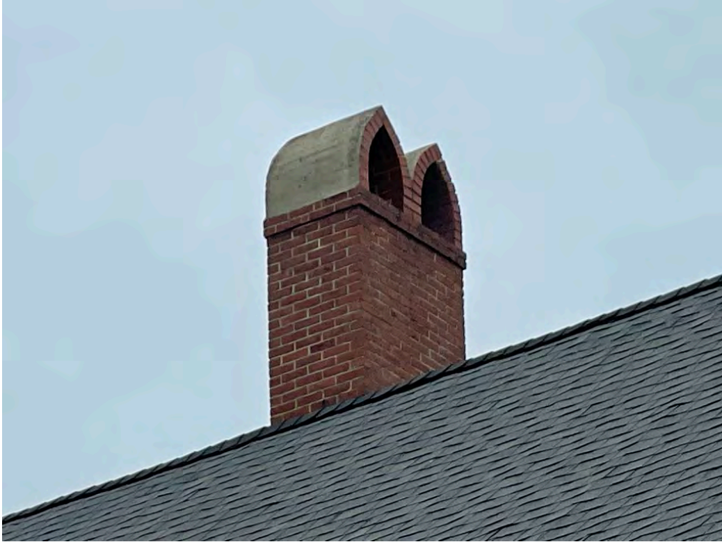
Image 43: View of the east chimney stack looking southwest, showing typical, minor mortar loss.
