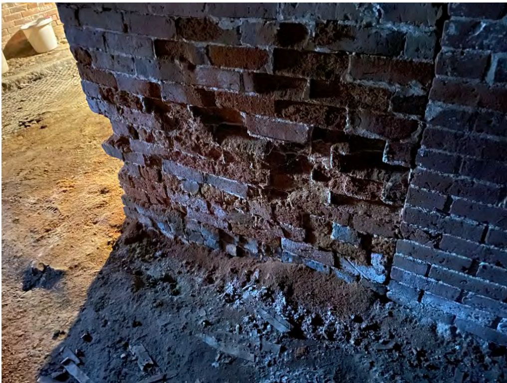
Image 42: Detail of the west chimney base in the basement showing typical brick deterioration from rising damp.
