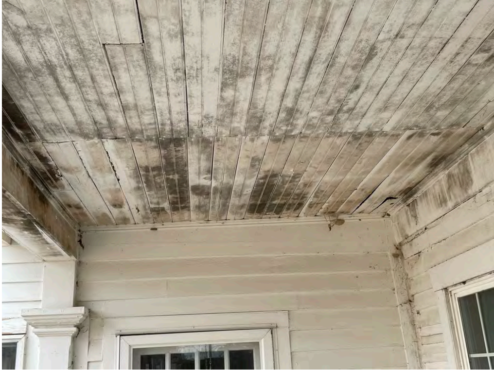
Image 41: Detail of the porch ceiling looking west, showing mold growth and warping due to past water infiltration.
