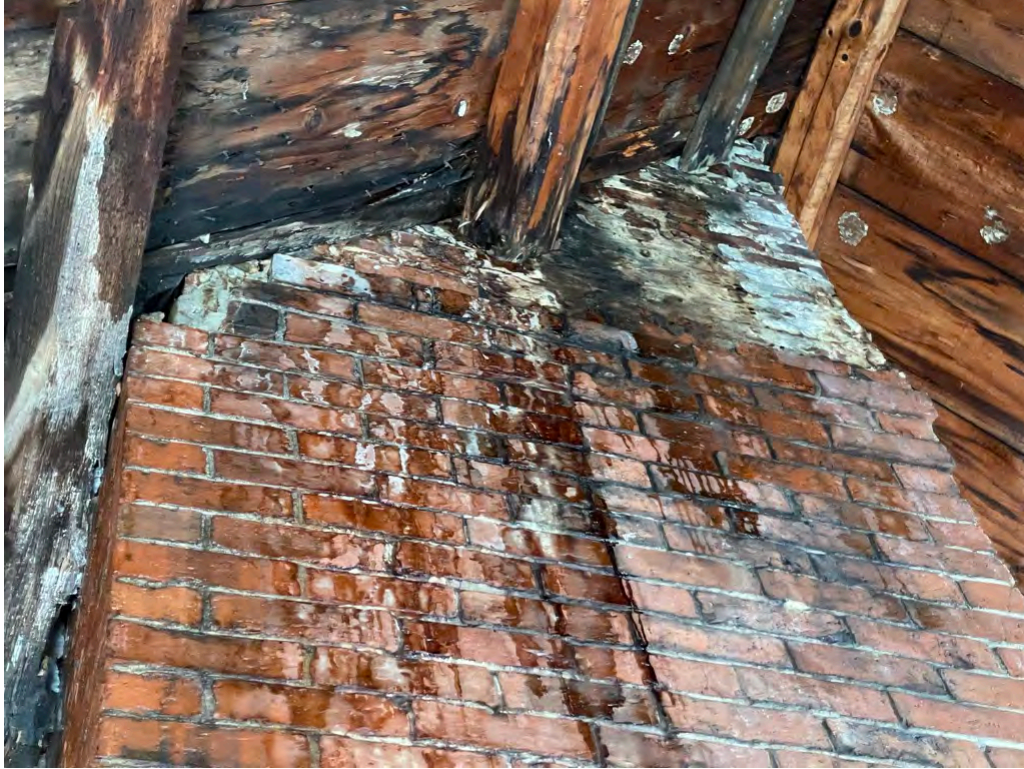
Image 35: Detail of east chimney showing the stack extension on top of the original corbel, and old water staining.
