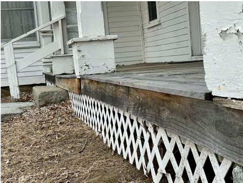
Image 40: Detail of the porch showing downward settling and decay of wooden elements.
