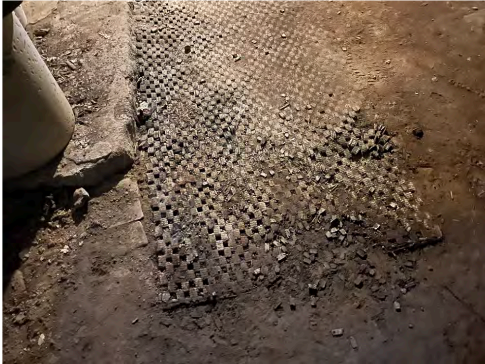
Image 49: Detail of the basement floor showing compacted soil from past water infiltration, and degraded floor mats.
