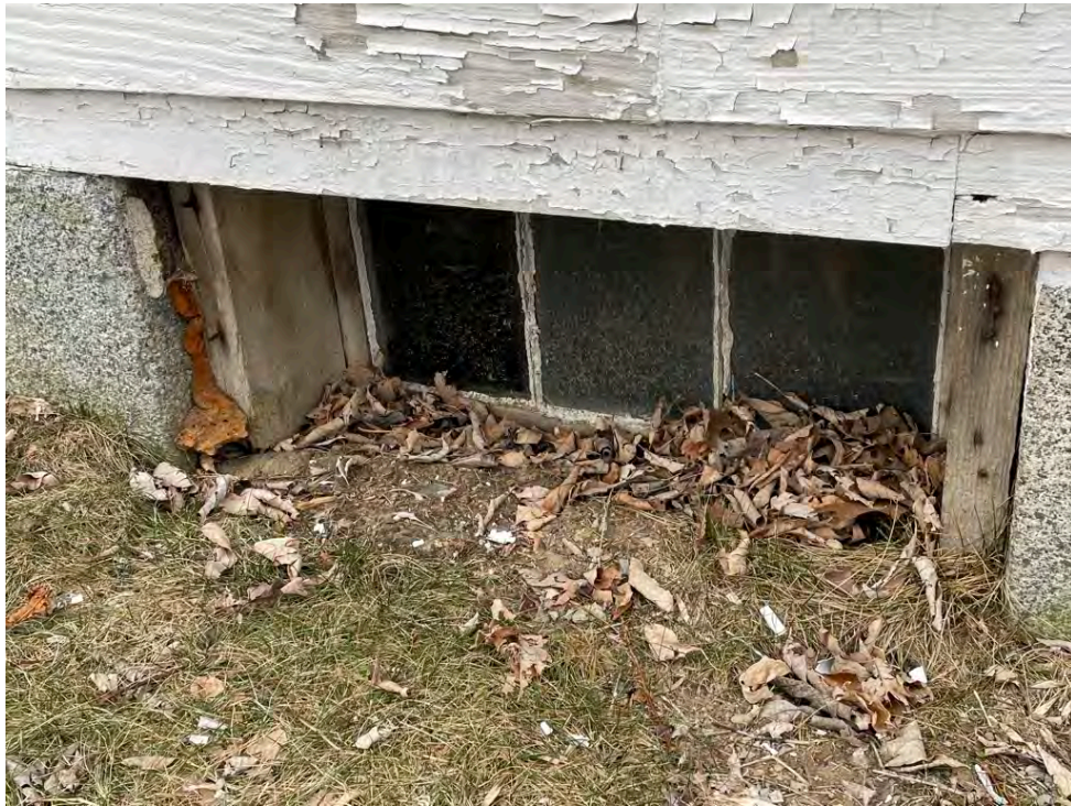
Image 51: Detail of a basement window, east elevation, showing encroaching grade and decay of the window elements.
