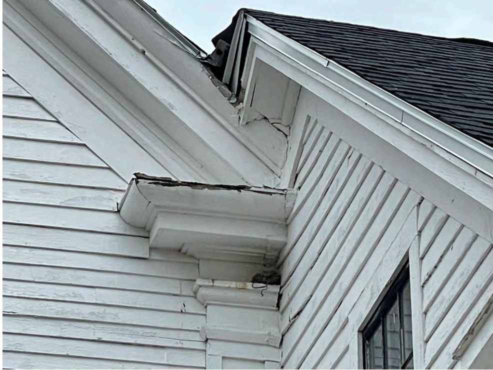
Image 37: Detail of cornice return and intersection of the main house to the ell, west elevation, showing water-related damage due to poor flashing and drainage.
