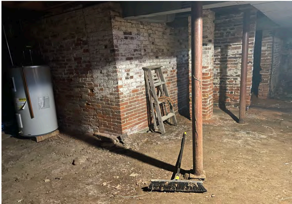
Image 10: View of basement looking northwest showing the west chimney base, added brick room partition and steel lolly columns.
