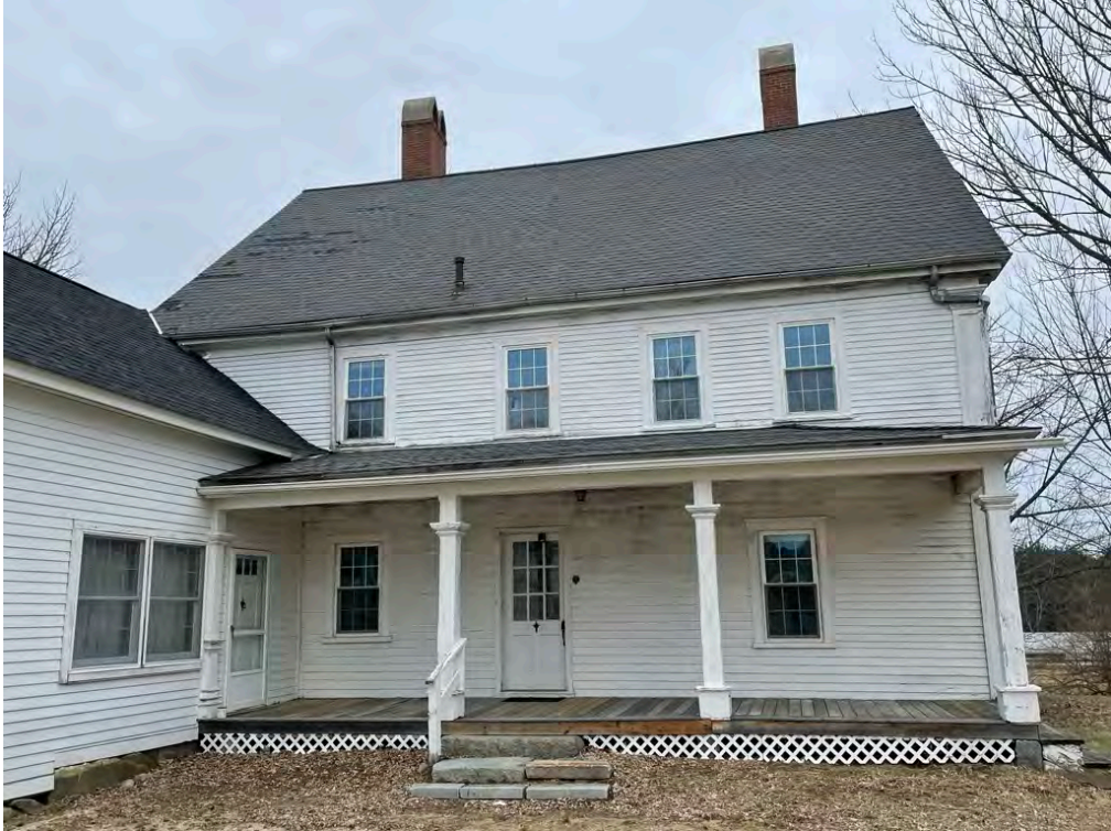
Image 39: View of the porch looking north, showing downward settling to the east.
