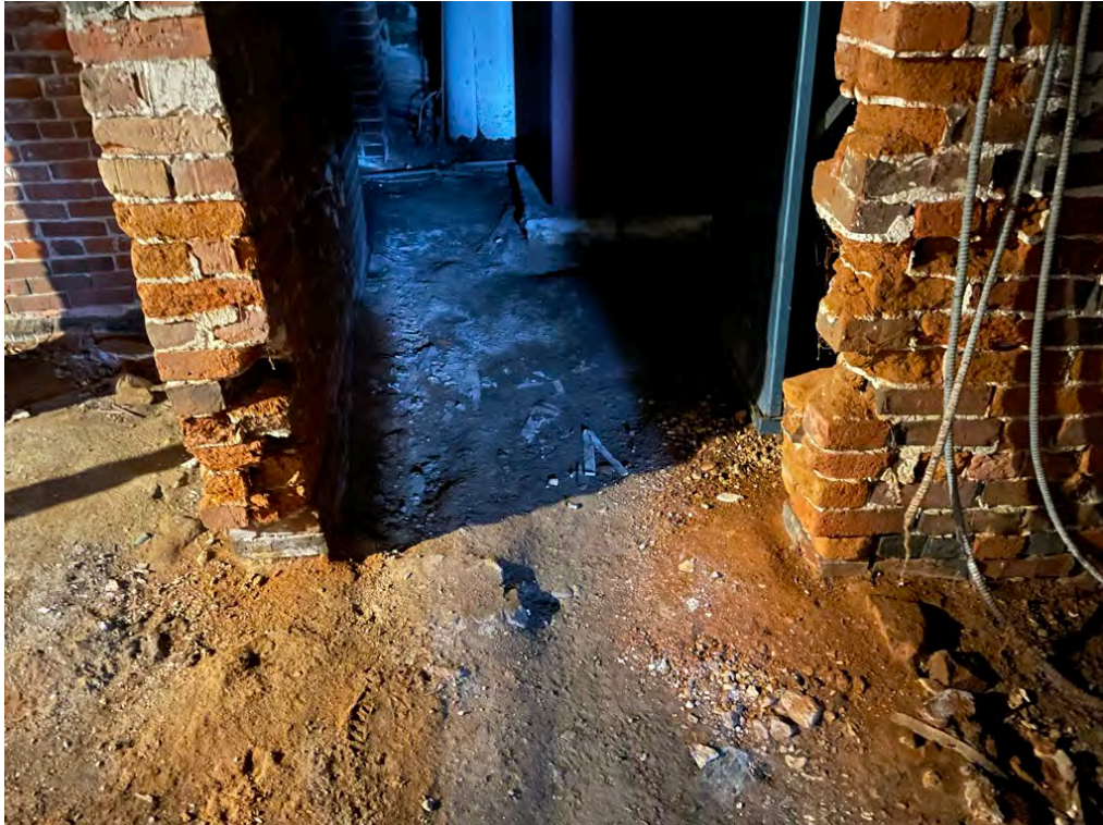
Image 34: View of typical rising damp in basement brick elements.
