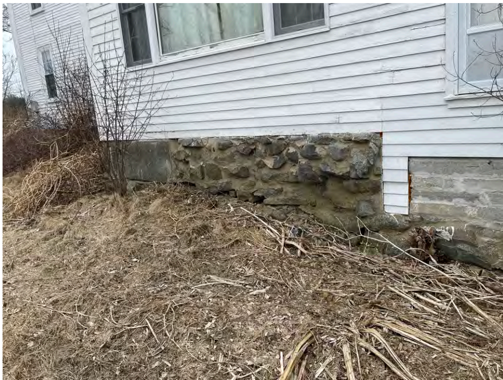
Image 48: View of the west elevation of the ell's foundation, showing variable materials and conditions.
