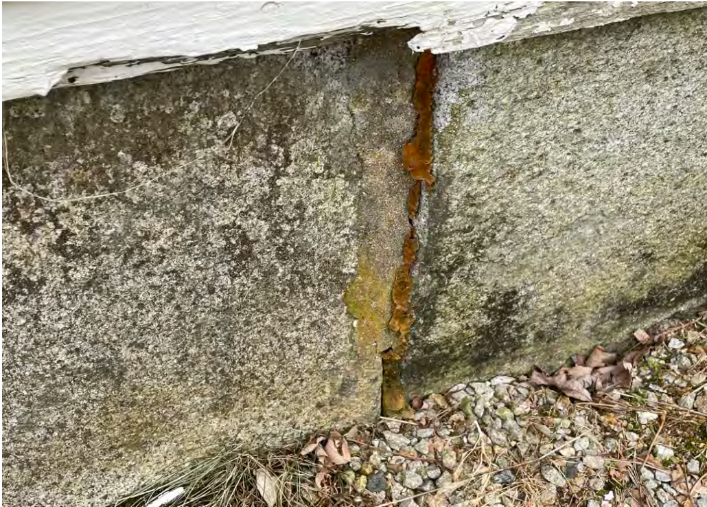
Image 44: Detail of foundation stone joint showing typical mortar loss and Spray foam repair.
