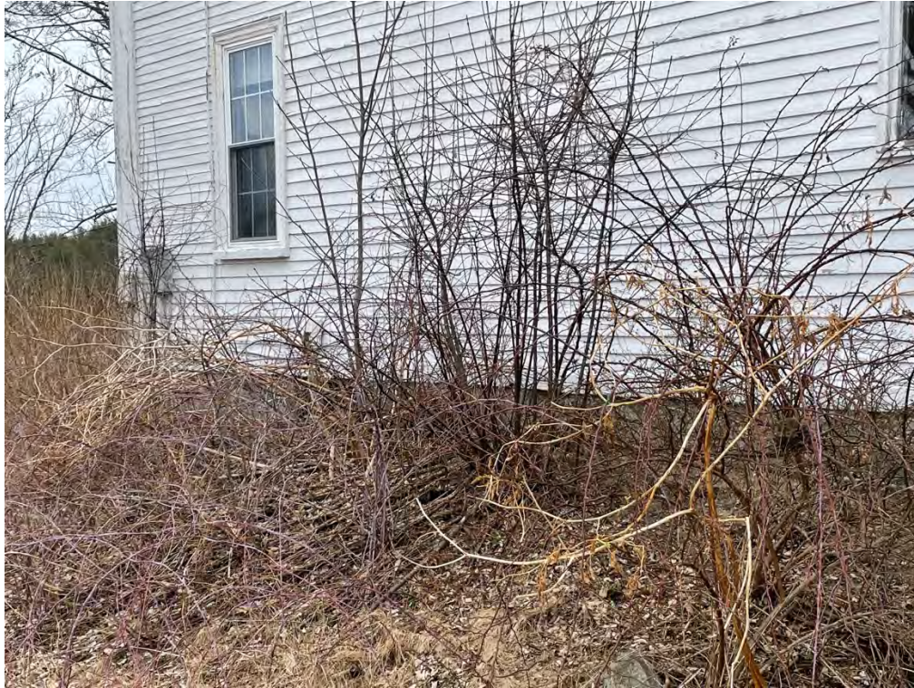
Image 45: View of the west elevation foundation, main house, showing overgrowth.
