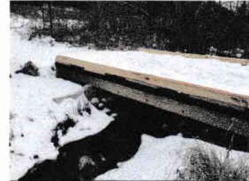
Recently installed bridge over tributary stream for pedestrian use and field maintenance equipment.
