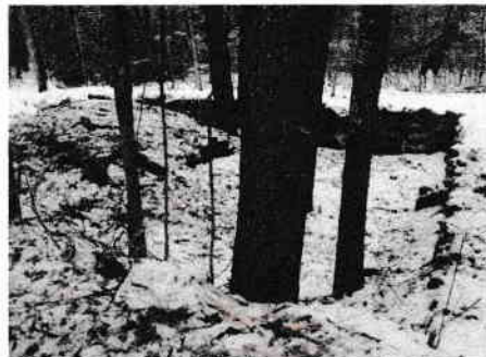
Trees within cellarhole may need eventual removal to prevent damage to walls.
