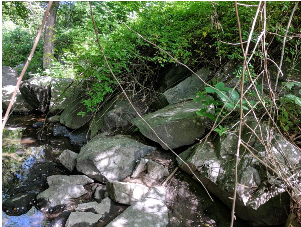
Picture G - Rip rap armoring on steep bank that was either placed in the stream, or has failed and fallen into the stream. Note the relative lack of vegetation here compared to other pictures of the stream and banks.
