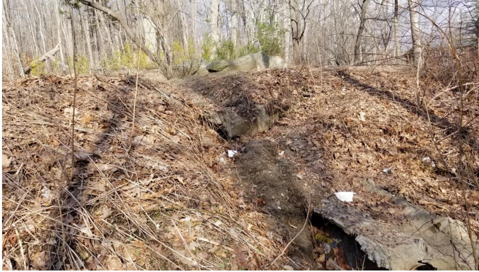
Picture F - Steep bank instability resulting from direct impervious cover runoff over bank
