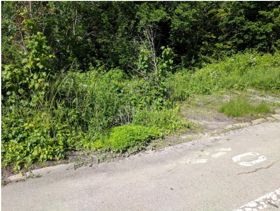
Picture D - Direct impervious cover runoff over steep bank and into riparian corridor
