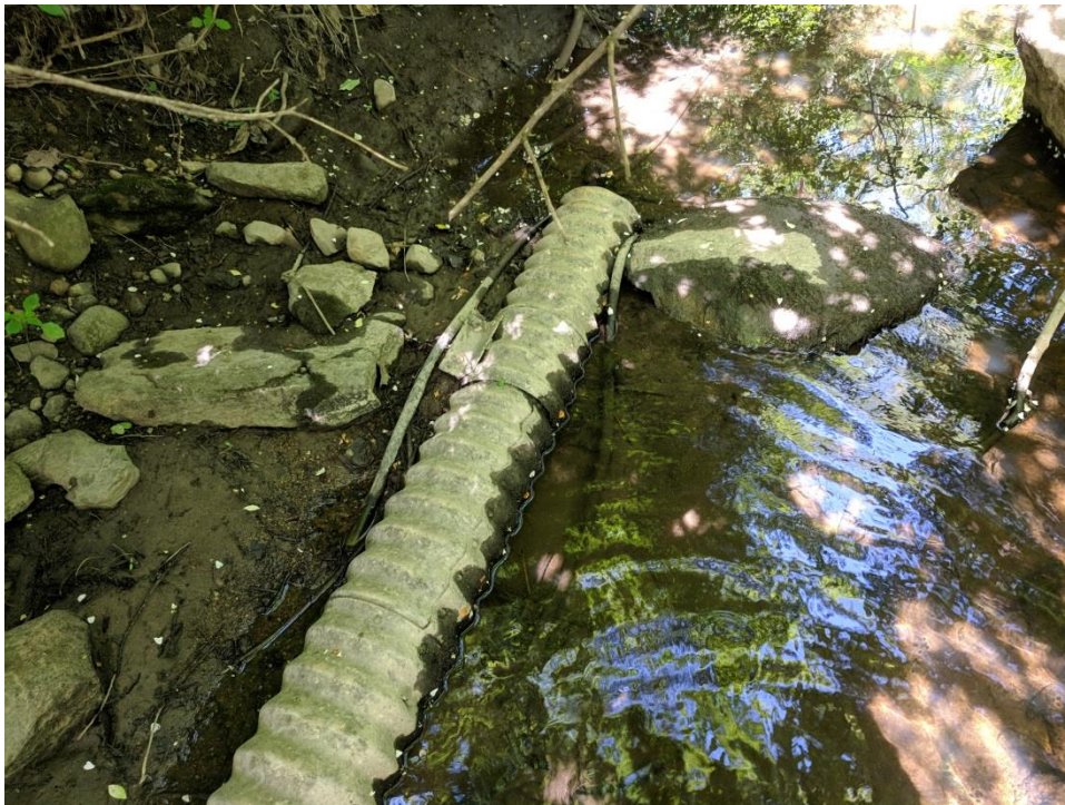
Picture I - Example of some of the trash that is in the stream and could be cleaned up. This section of CMP culvert was either tossed here or failed and was carried here, now half-buried.
