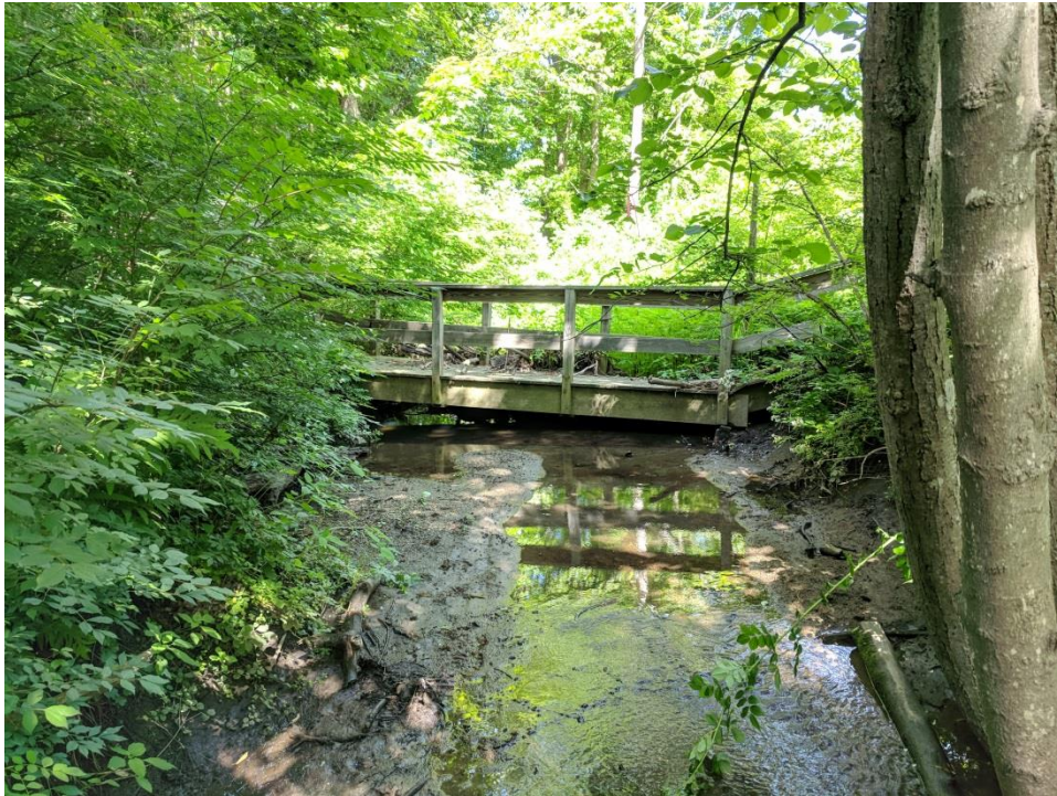
Picture H - Existing foot bridge that is no longer in use (it is blocked off at both ends). Note that this structure was built almost in the stream, and the effects of it on the channel at this location are noticeable.
