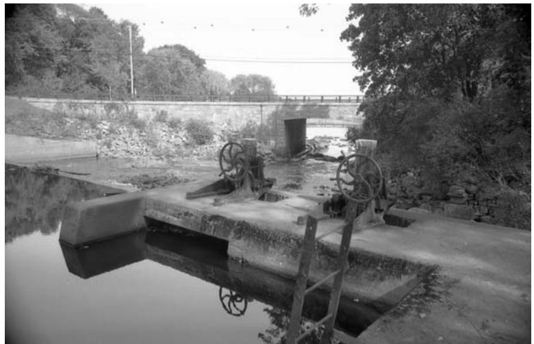
fig.8 neg0023 back of control structure looking ENE bridge over rt 108 visible in background
