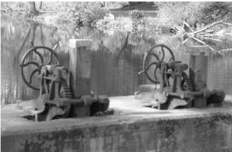
fig.7 neg0035 control structure looking WNW turbine gate on left, waste gate on right.
