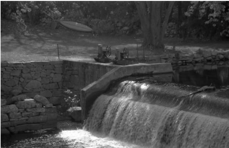
fig. 5 neg0008 control structure and dam looking SSW remains of Jenkins Mill foundation and gat
