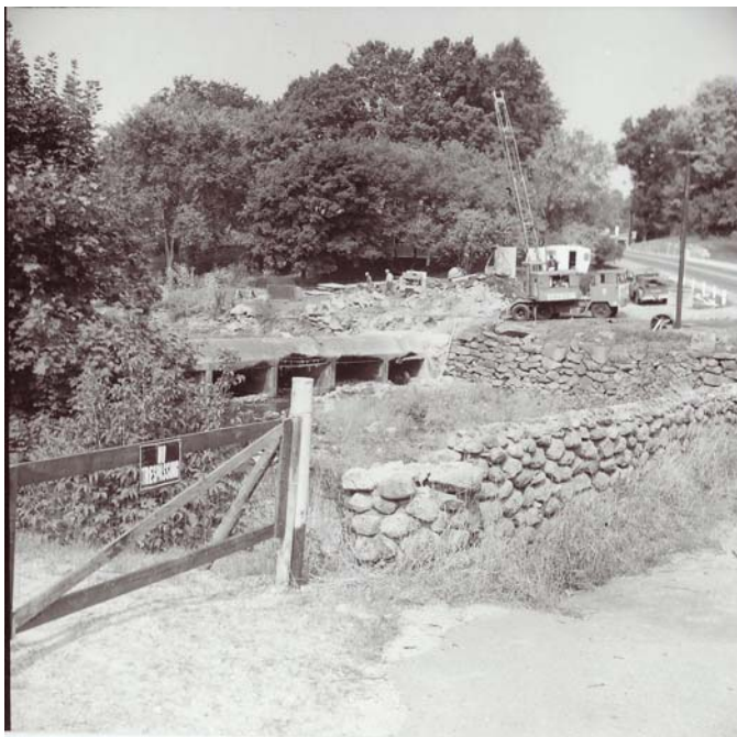
Gateway to Jenkin's cottage in forground. Work on dam about to begin looking NW
