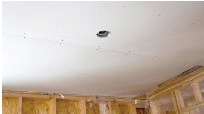
The IRC does not require the gypsum board applied to the underside of the I-joist floor systems to be covered with tape and joint compound.
