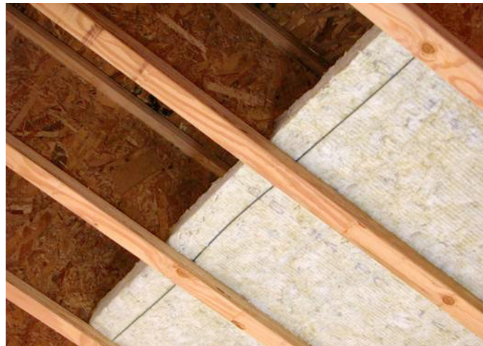
Installing mineral wool between I-joists is one of several methods builders and installing dealers can use to meet the IRC provisions.
