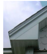
Porkchop eaves are clunky and inappropriate. (77)
